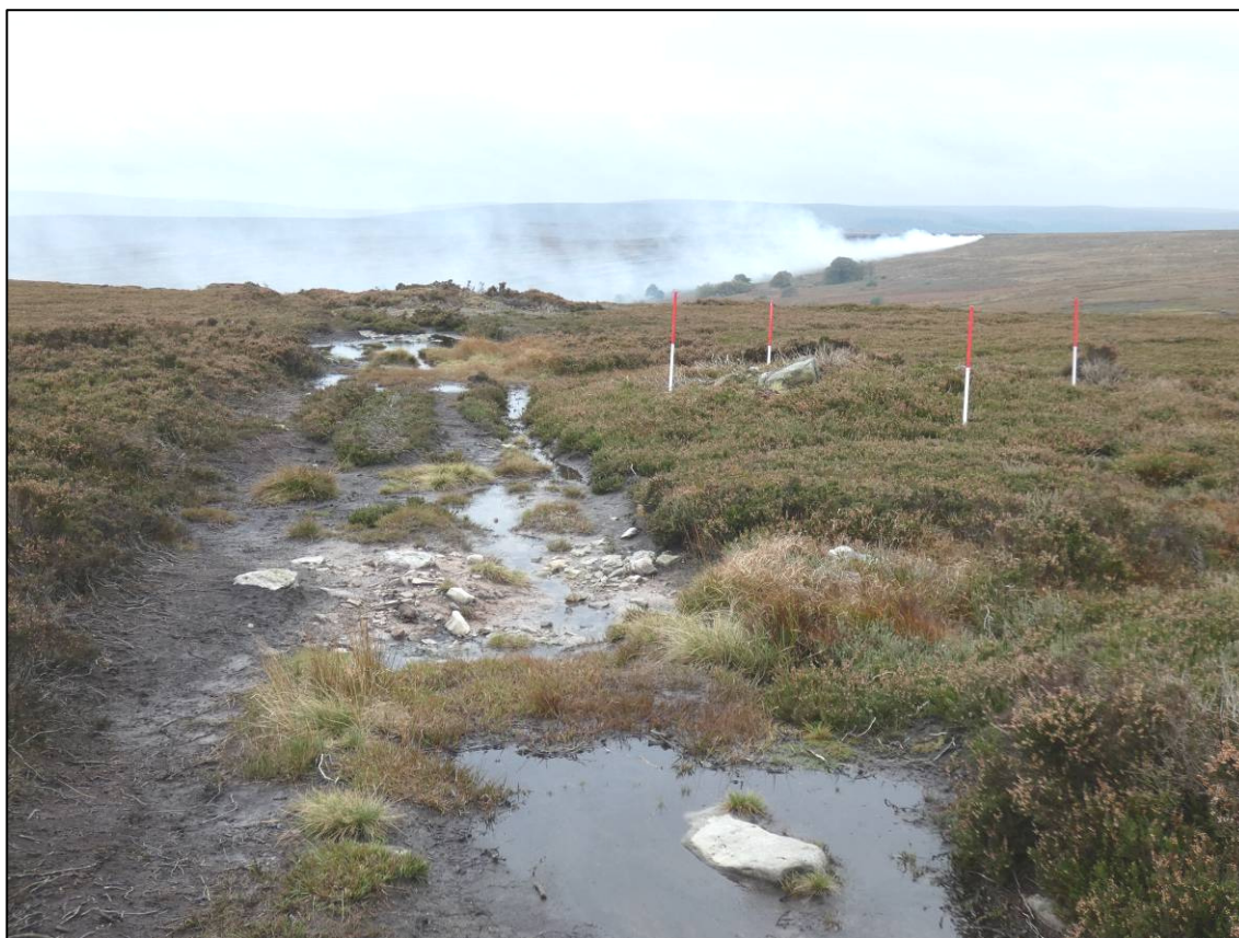
Plate 2: General view of shooting track showing proximity to cairn, water ponding and previous repairs (10th October 2019).
