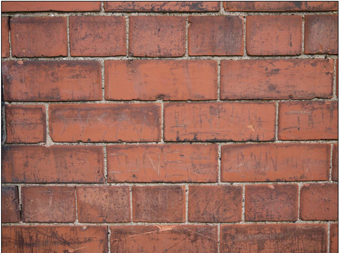
Plate 10: 1911 school building (Block 1), detail of graffiti on gable of central projection to south elevation, looking NE (photo 1/140).
