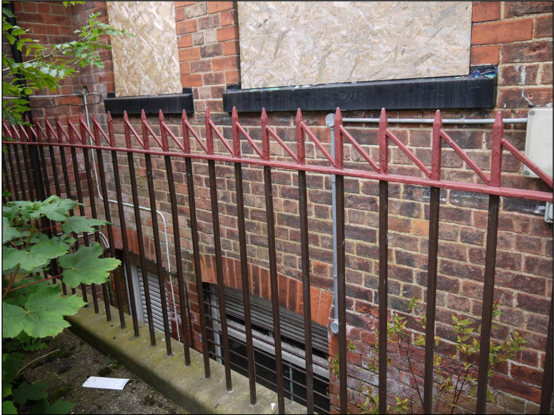
Plate 13: 1911 school building (Block 1), north elevation, detail of railings to boiler house steps, looking SW (photo 1/130).
