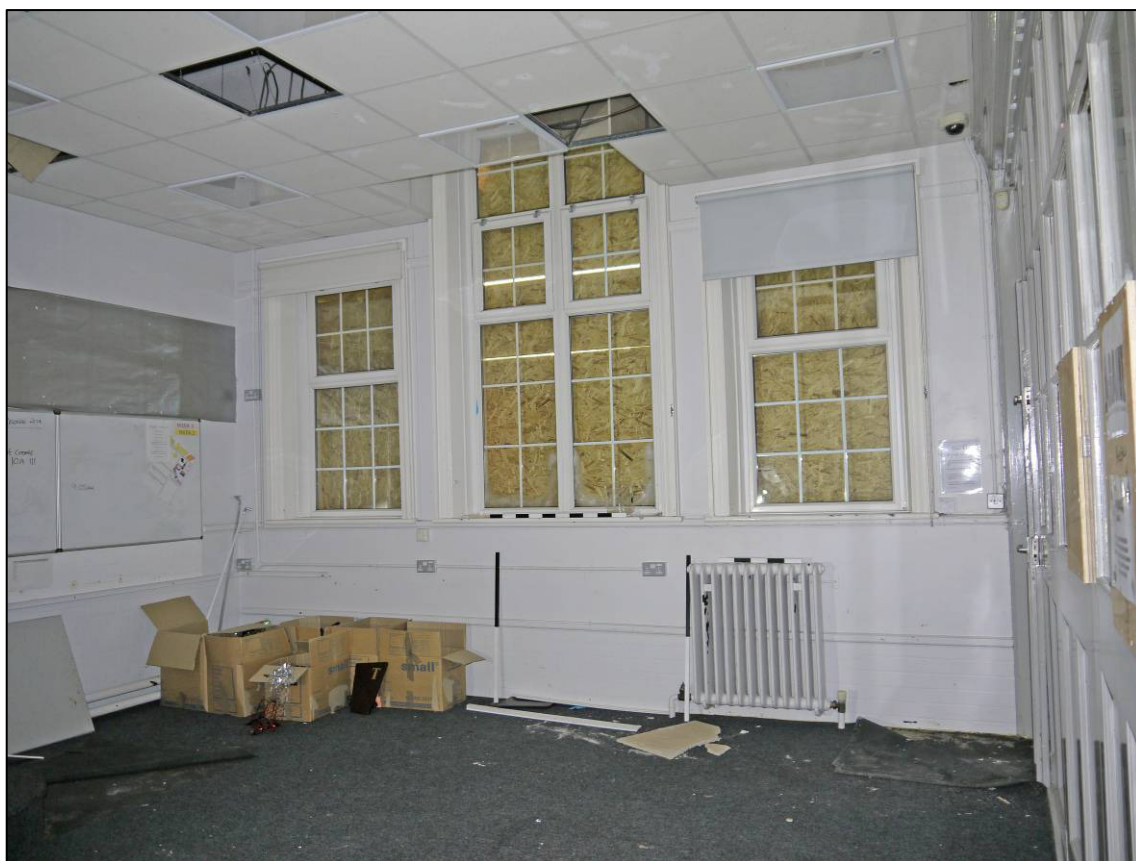
Plate 23: 1911 school building (Block 1), classroom (G/005), windows and rib-type radiator to east wall, looking E (photo 1/019).
