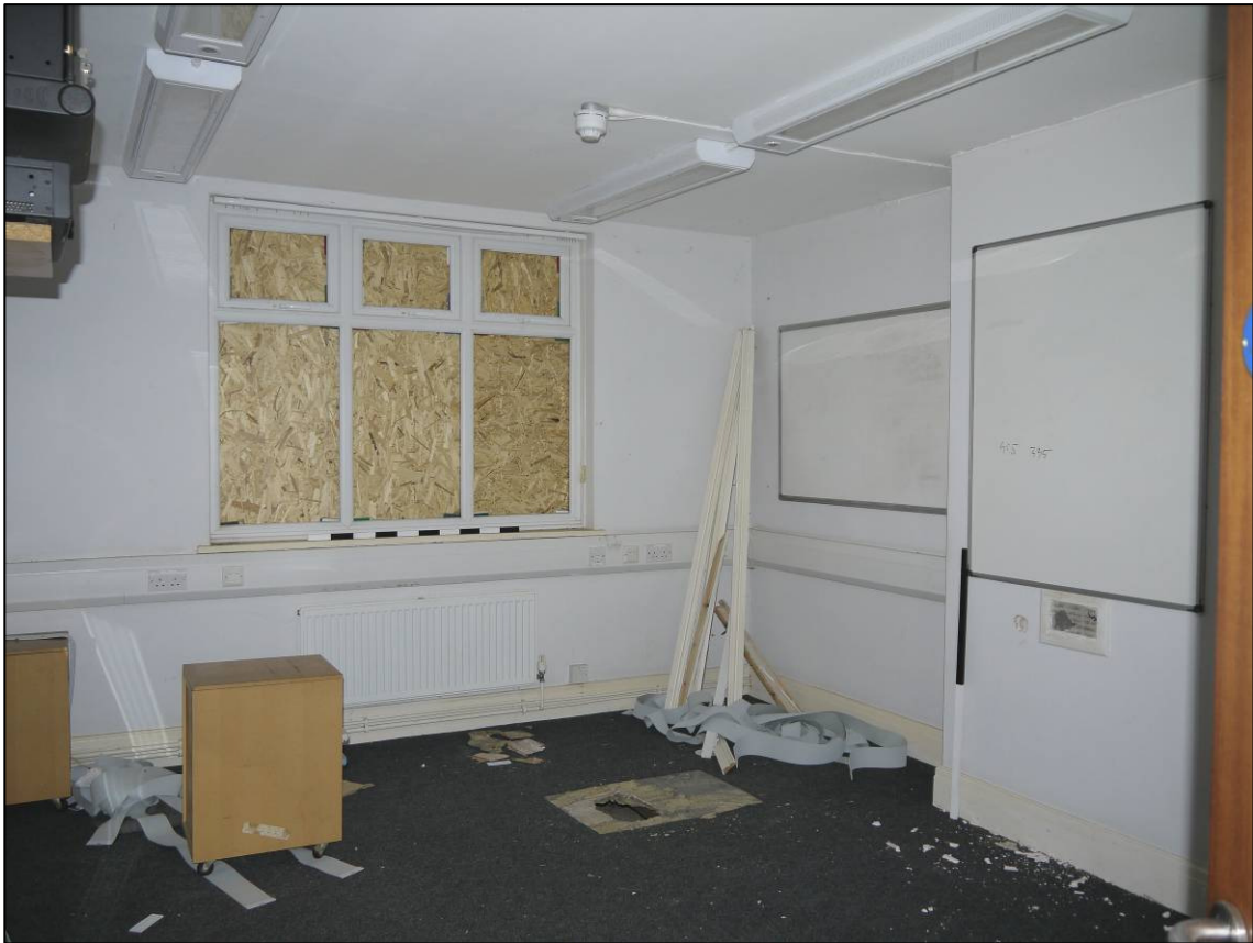
Plate 37: 1923 house (Block 3), former canteen (G/003) showing blocked fireplace in west wall, looking W (photo 1/051).
