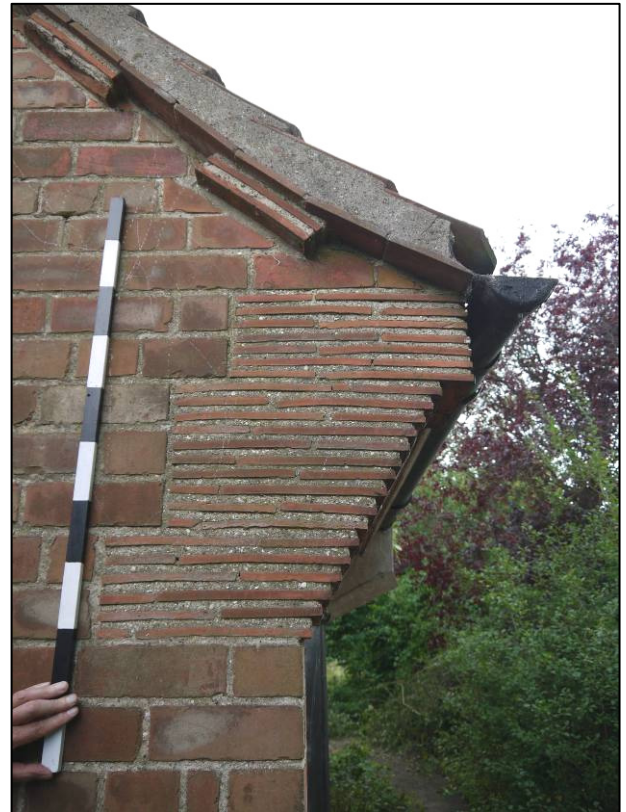
Plate 32: 1923 house (Block 3), north elevation, detail of tiled kneeler and decoration to eaves, looking SW (photo 1/159).
