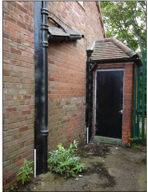
Plate 27: 1923 house (Block 3), porch to north side, with adjacent blocked window, looking W (photo 1/166).
