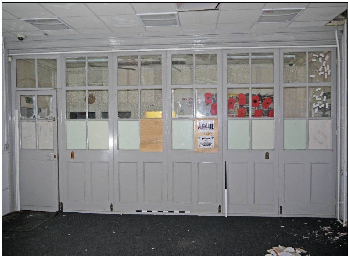
Plate 22: 1911 school building (Block 1), classroom (G/005), folding screen to south wall, looking SW (photo 1/021).
