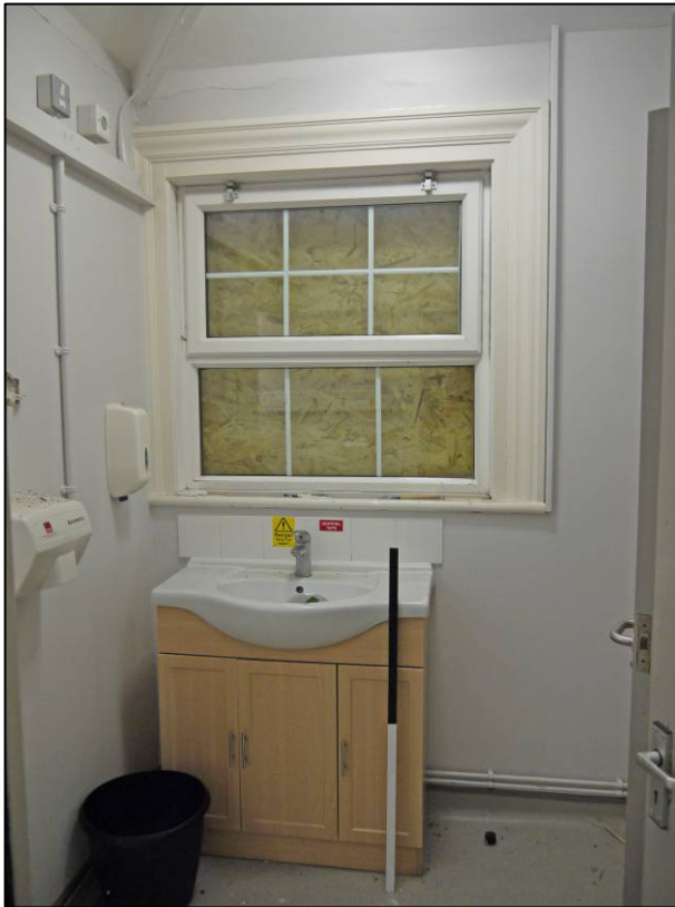
Plate 26: 1911 school building (Block 1), WC (G/009B), window to west wall, looking NW (photo 1/043).
