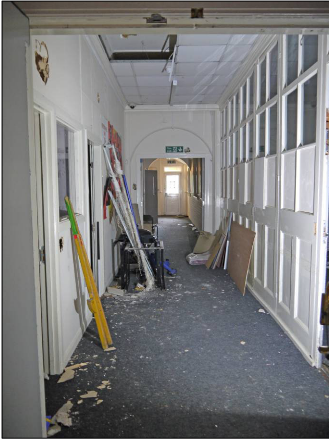
Plate 20: 1911 school building (Block 1), central part of internal corridor (G/001), with folding screen to right, looking NW (photo 1/006).
