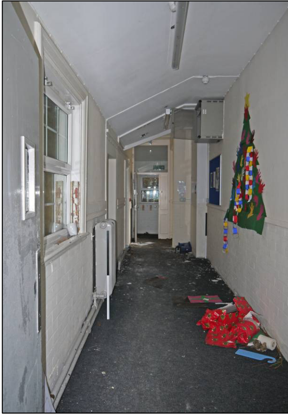
Plate 17: 1911 school building (Block 1), east end of internal corridor (G/001), looking SE (photo 1/001).
