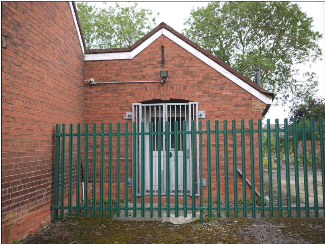
Plate 5: 1911 school building (Block 1), former girls' entrance in south elevation, looking NE (photo 1/151).
