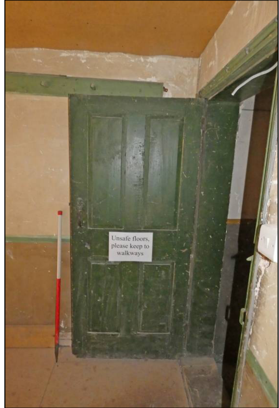
Plate 65: South range, first floor room (1F6), doorway to west wall stairs, looking SE (photo 3/583).
