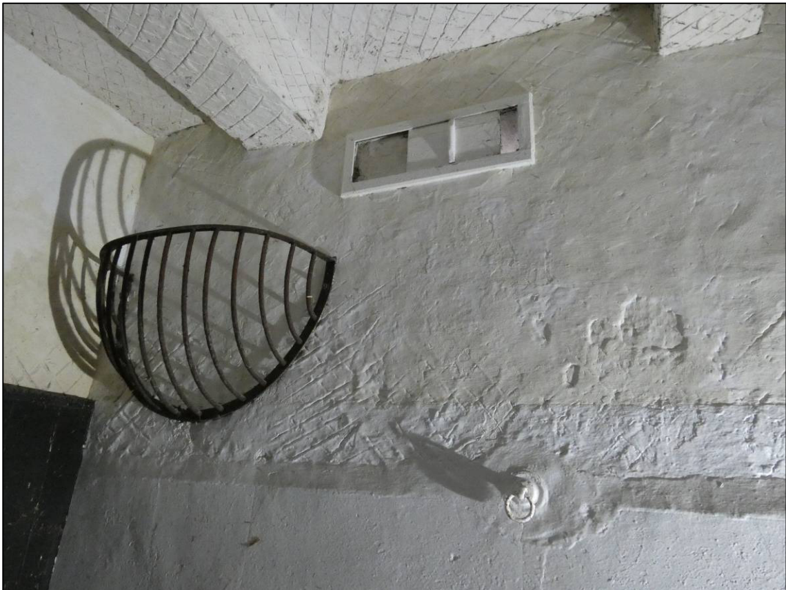
Plate 33: East range, ground floor loose box (GF2), hay rack, tethering ring and wooden ventilator, looking NE (photo 1/708).
