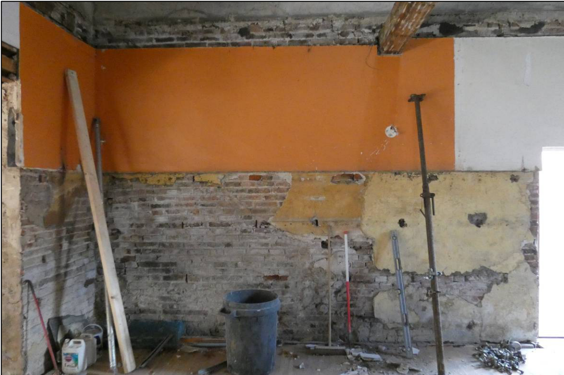
Plate 49: South range, ground floor room (GF9 - cafe) during alterations, showing scar of ramped stall partition to west wall, looking SW (photo 4/791).
