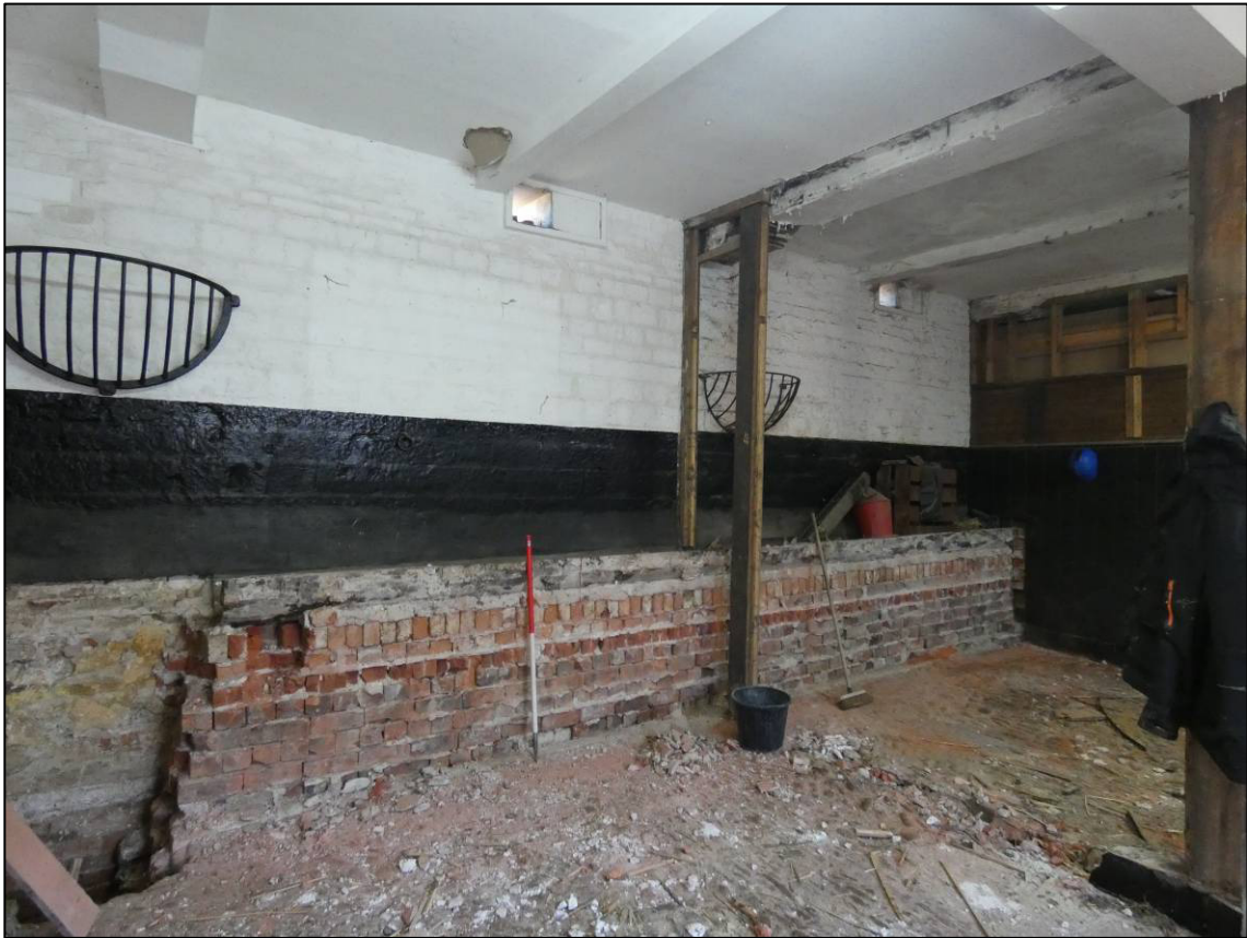
Plate 46: East range, ground floor loose boxes (GF5 and GF6) during alterations, showing hay racks, manger, ventilators and stonework to east wall, looking E (photo 2/135).
