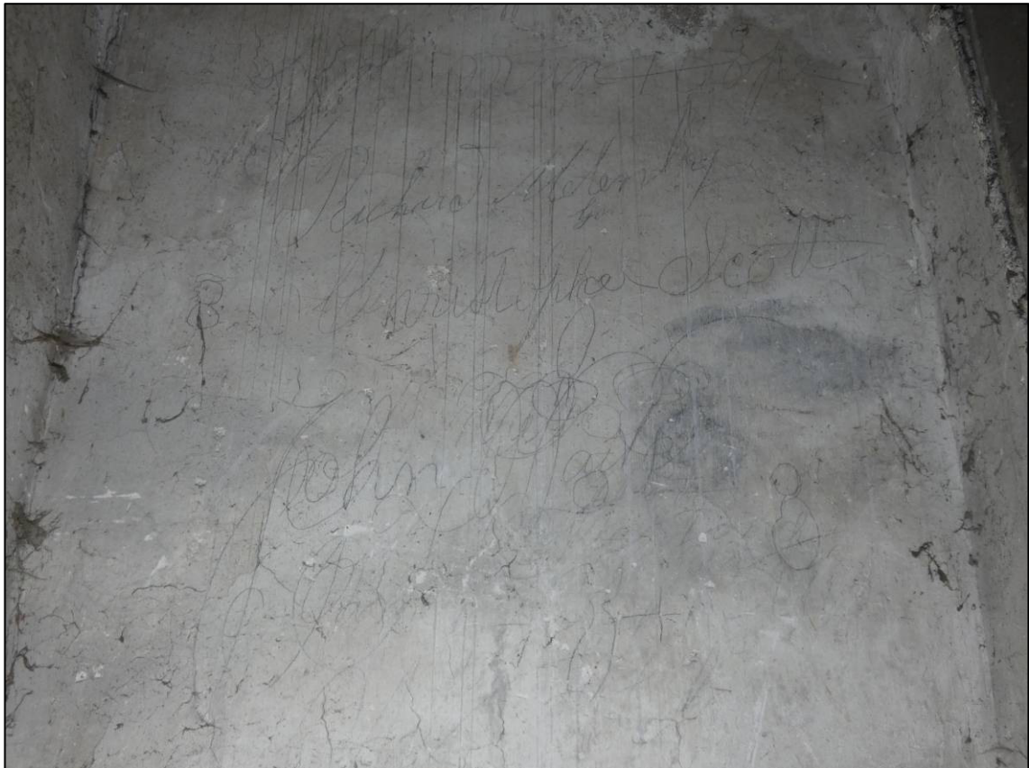
Plate 79: South range, western stairs to first floor rooms, graffiti to wall at head of stairs (photo 1/803).
