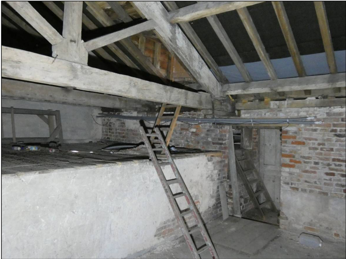
Plate 84: South range, first floor room (1F9), showing raised area at east end, looking E (photo 1/827).
