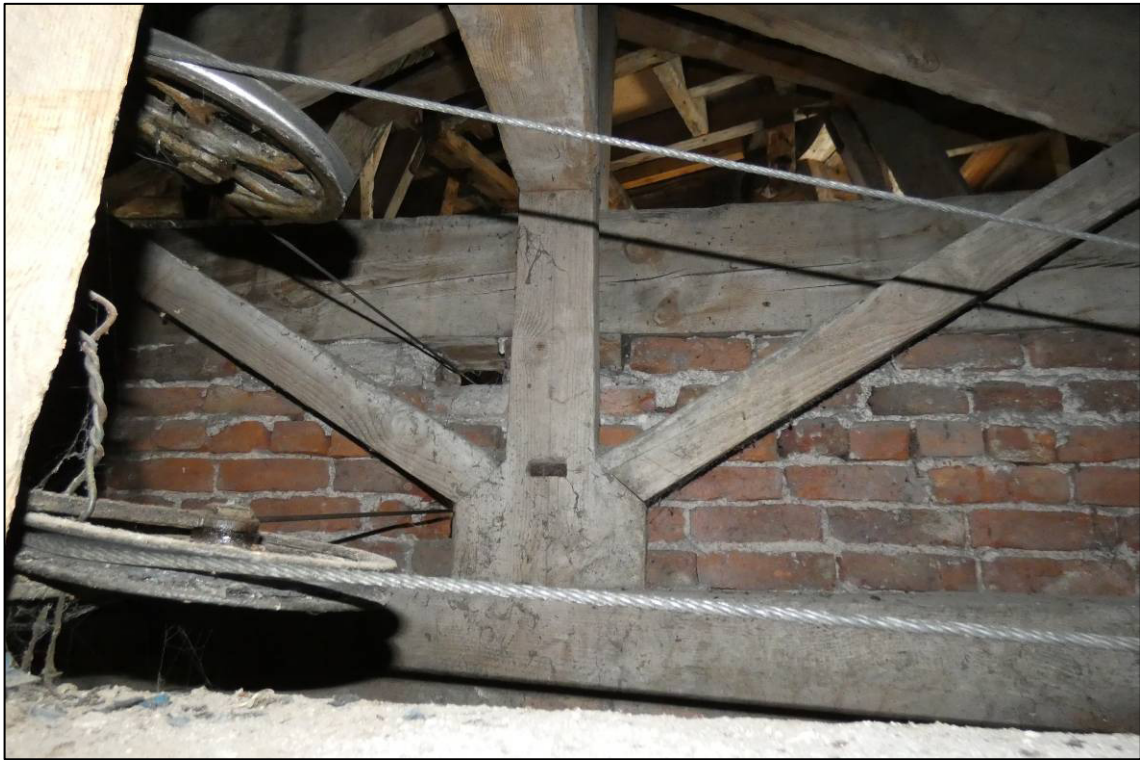
Plate 70: South range, first floor room (1F6), truss to west wall, looking SW (photo 3/580).
