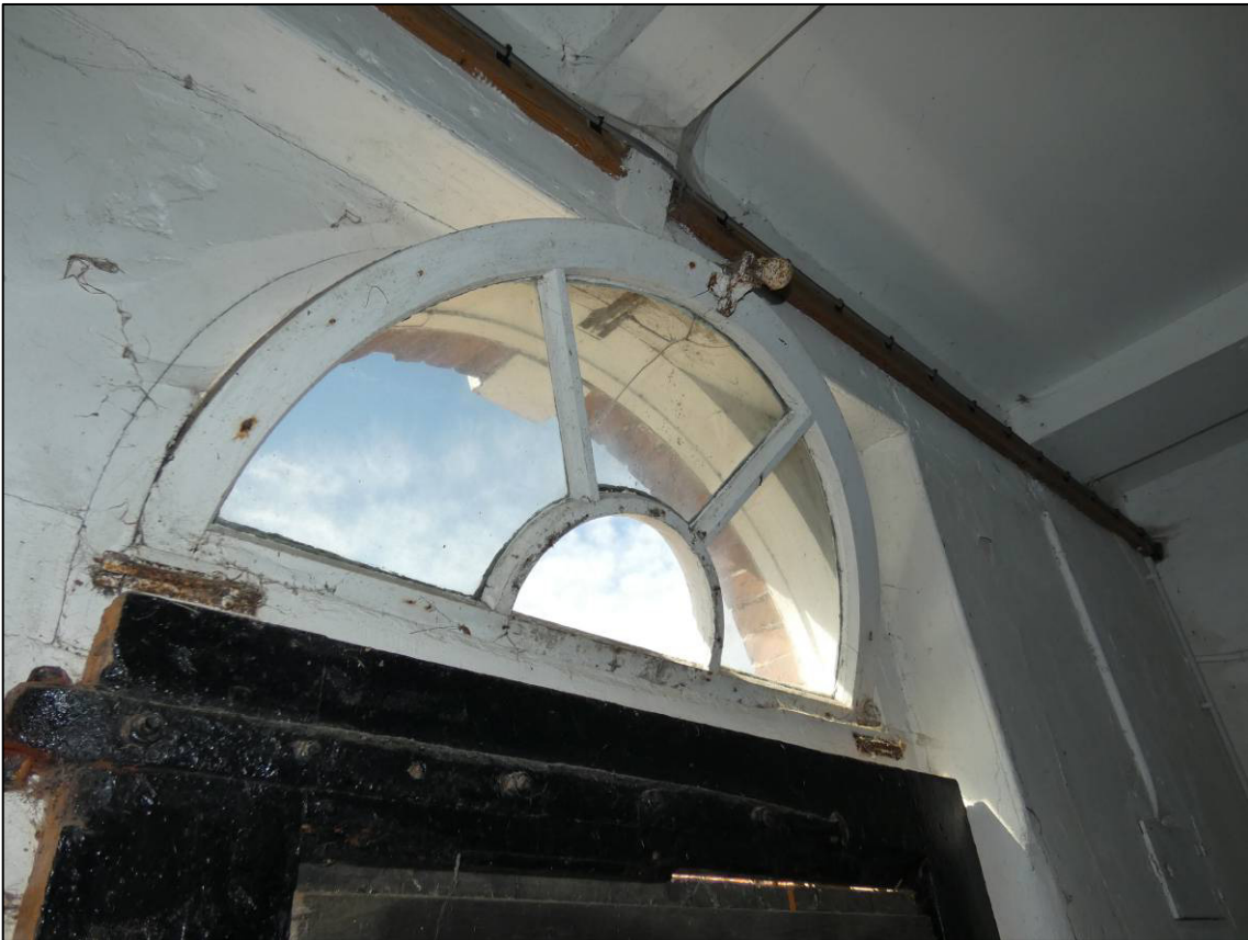
Plate 43: East range, ground floor loose box (GF5), overlight to door in west wall, looking NW (photo 1/746).
