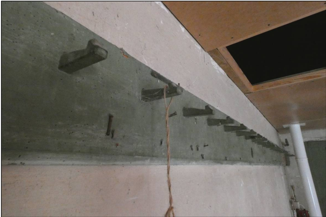
Plate 68: South range, first floor room (1F6), pegs to west wall, looking NW (photo 3/582).
