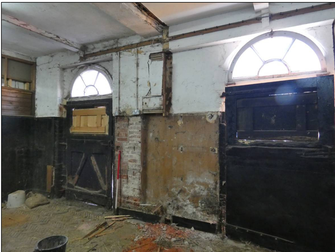
Plate 45: East range, ground floor loose boxes (GF5 and GF6) during alterations, showing joint and lath and plaster panel to west wall, looking S (photo 2/144).
