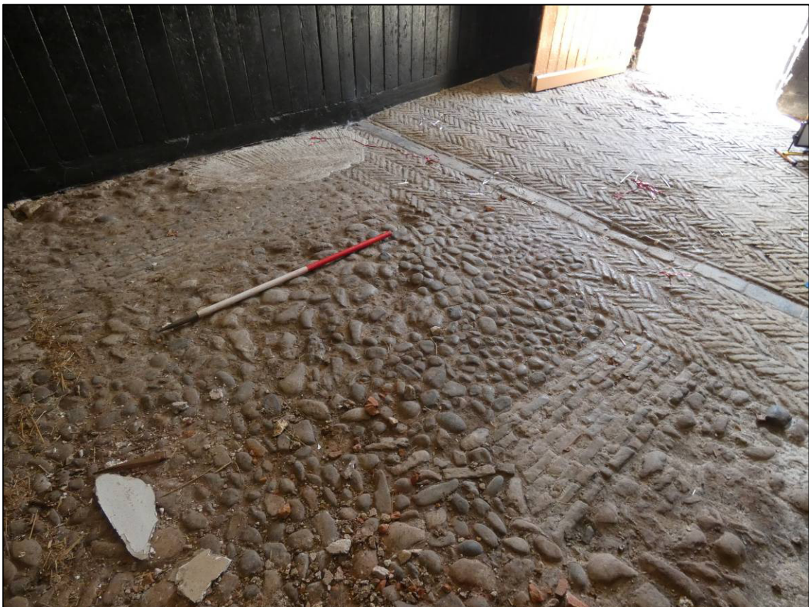
Plate 41: East range, ground floor loose box (GF5), cobble, brick and clinker floor, looking S (photo 1/738).
