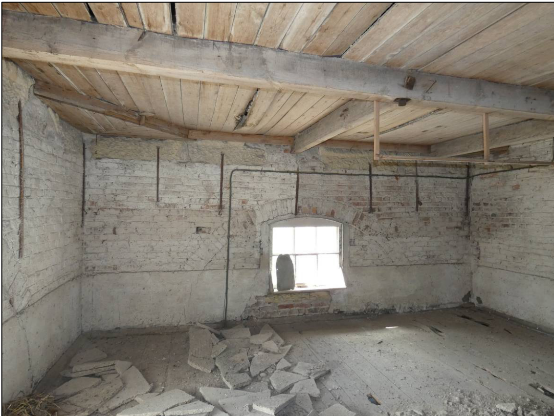
Plate 81: South range, first floor room (1F11), window and stonework with iron clamps to west wall, looking SW (photo 1/815).
