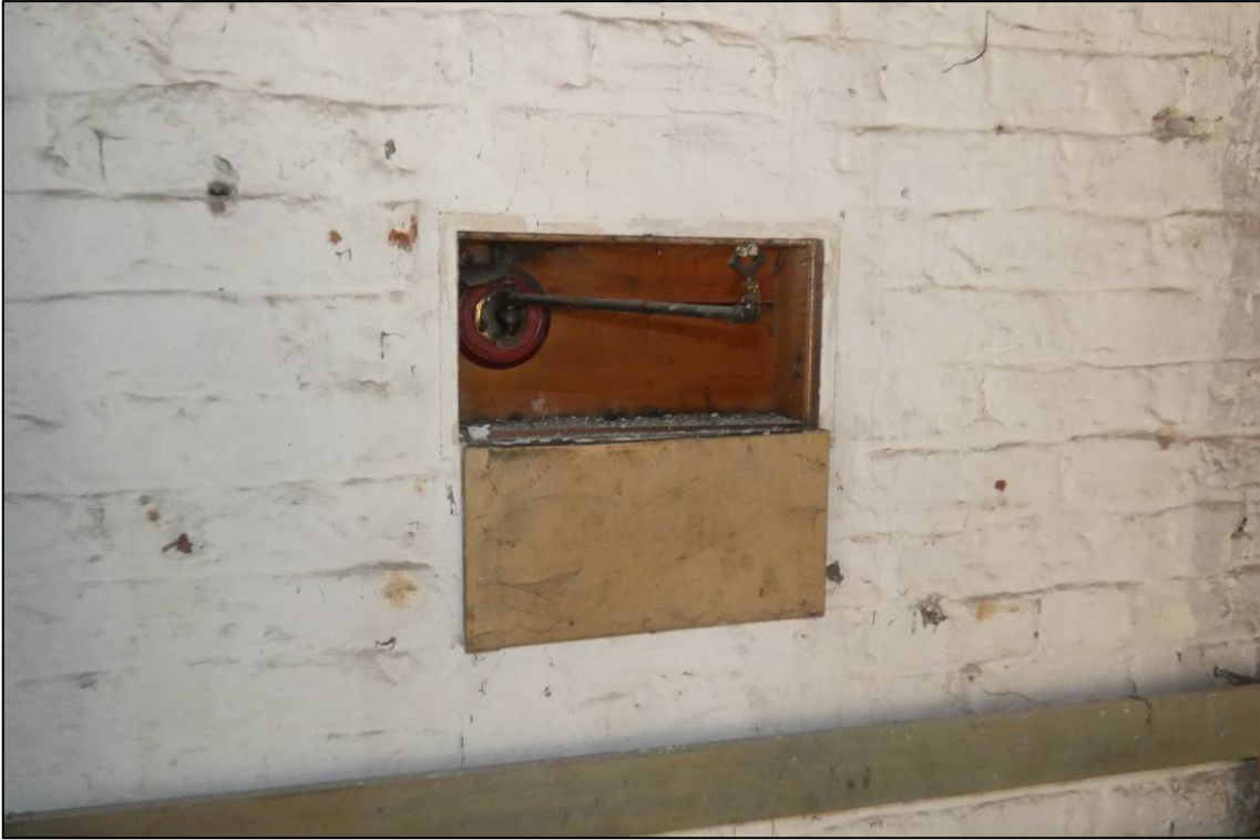
Plate 48: South range, ground floor room (GF8 - cafe), gas light control box with fitting to west wall, looking SW (photo 4/836).
