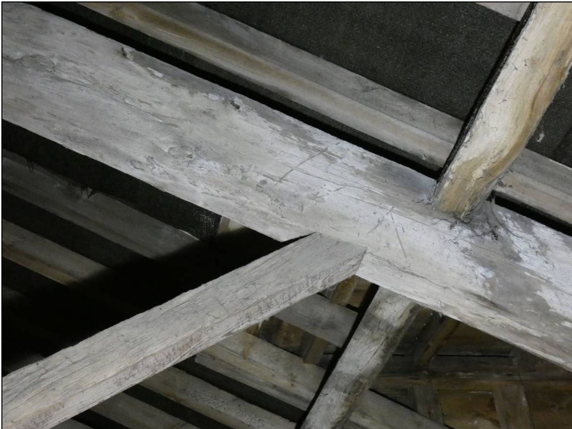
Plate 85: South range, first floor room (1F9), Baltic timber marks to truss, looking S (photo 1/831).
