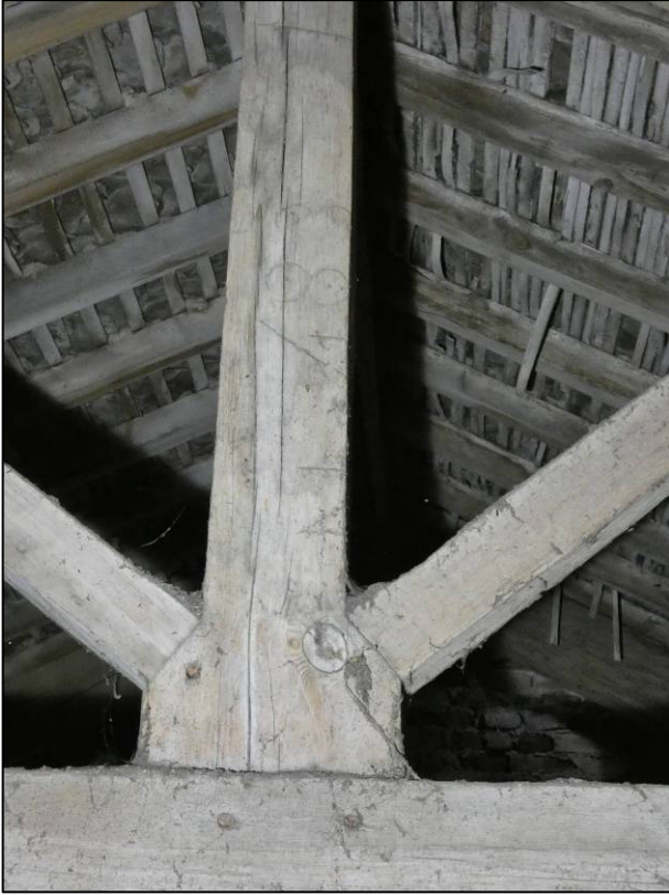
Plate 62: East range, first floor room (1F3), Baltic timber marks to truss, looking SE (photo 1/792).
