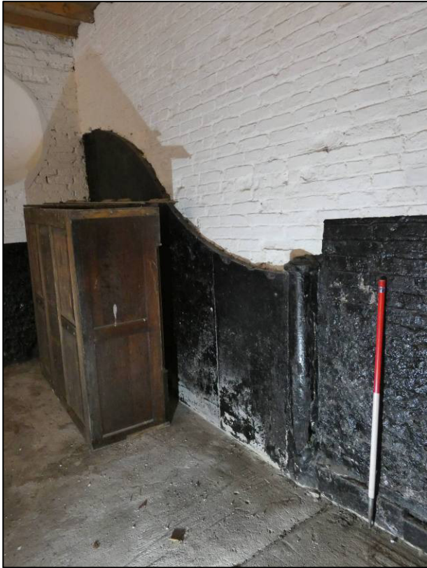
Plate 29: North range, east end, ground floor room (GF1), stall partition to east wall, looking N (photo 1/680).
