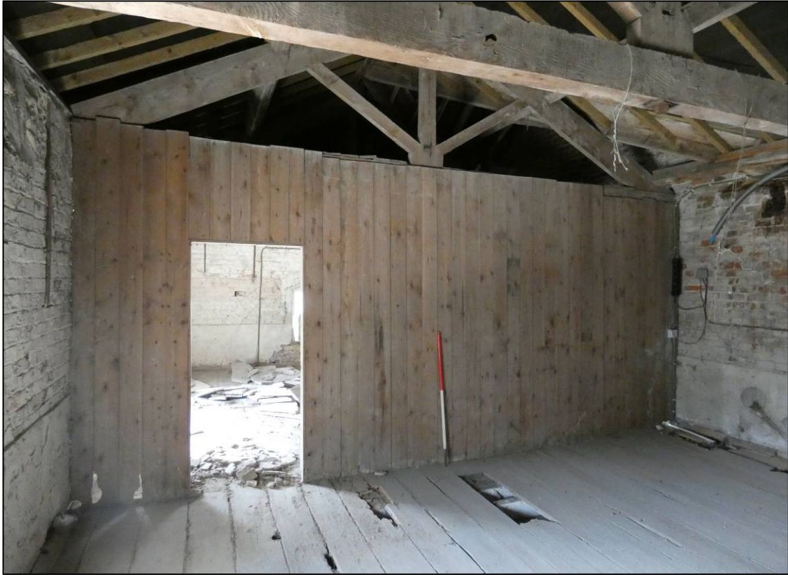
Plate 80: South range, first floor, partition between rooms 1F10 and 1F11, looking SW (photo 1/808).
