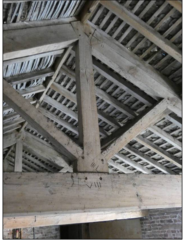
Plate 63: East range, first floor room (1F3), carpenters' marks to truss, looking SE (photo 2/154).
