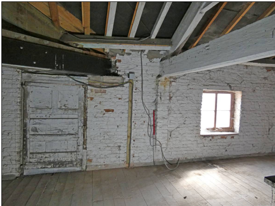
Plate 57: North range, east end, first floor room (1F1), west part of south wall, looking SE (photo 1/839).
