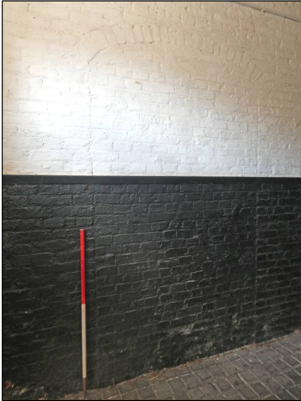
Plate 39: East range, ground floor passage (GF4), blocked opening to north wall, looking N (photo 1/732).
