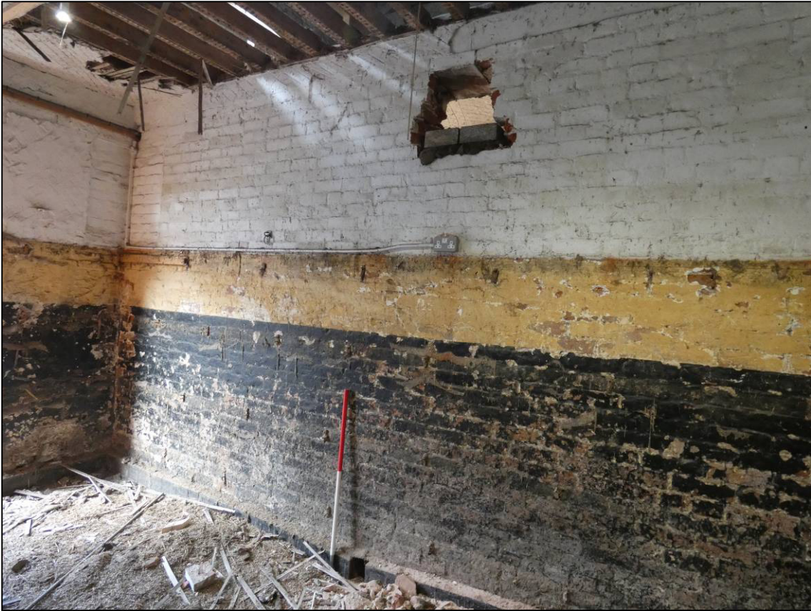
Plate 36: East range, ground floor loose box (GF3) during alterations, north wall showing decoration and blocking at west end, looking W (photo 2/124).
