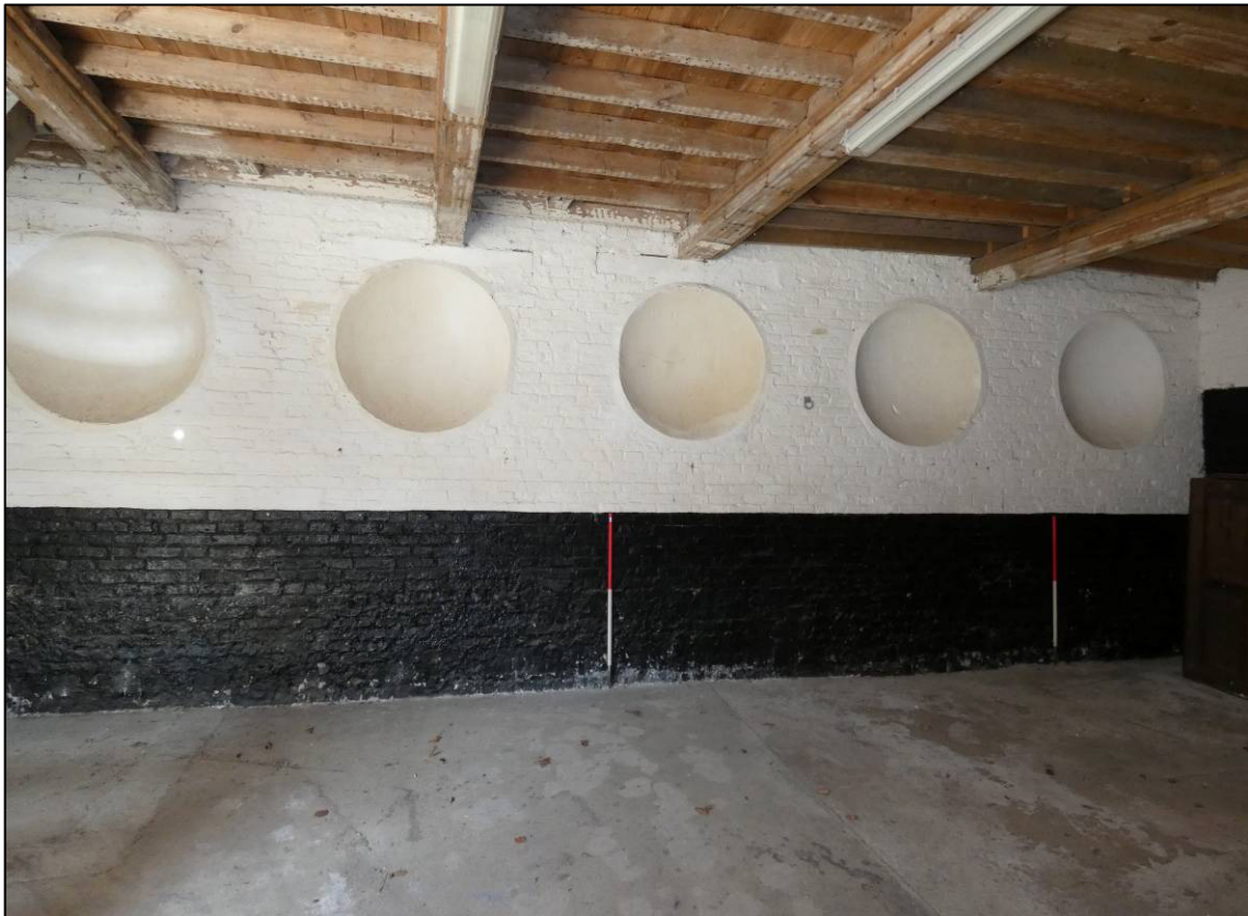
Plate 28: North range, east end, ground floor room (GF1), recesses to north wall, looking N (photo 1/676).
