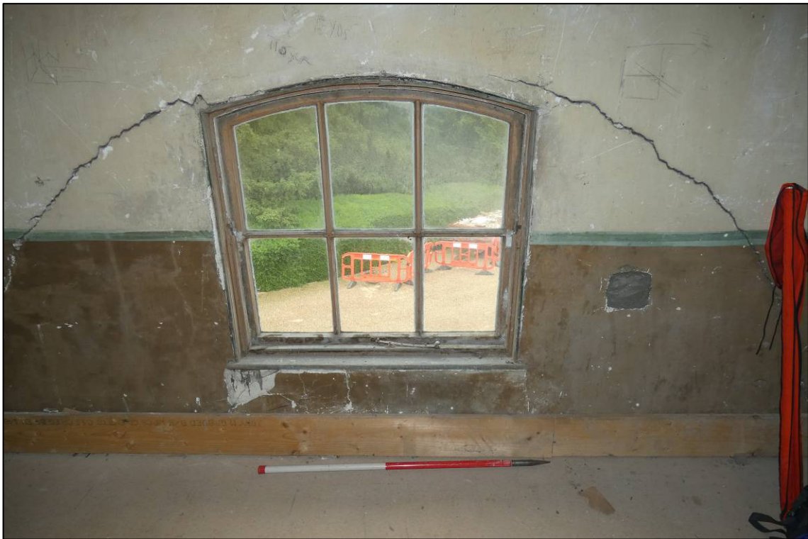
Plate 69: South range, first floor room (1F6), window to south wall, looking SE (photo 3/570).
