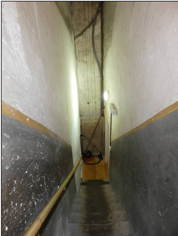
Plate 64: South range, eastern stairs to first floor rooms (1F5 and 1F6), looking SE (photo 1/762).
