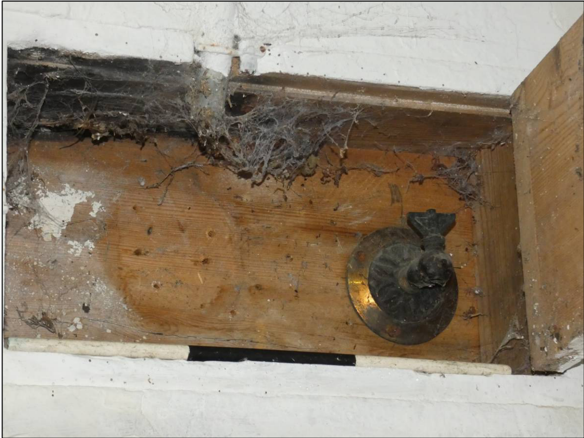
Plate 44: East range, ground floor loose box (GF5), gas light control box with fitting to west wall, looking SW (photo 2/142).
