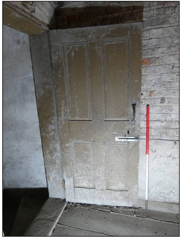
Plate 78: South range, first floor room (1F10), door at head of stairs in east wall, looking SE (photo 1/805).
