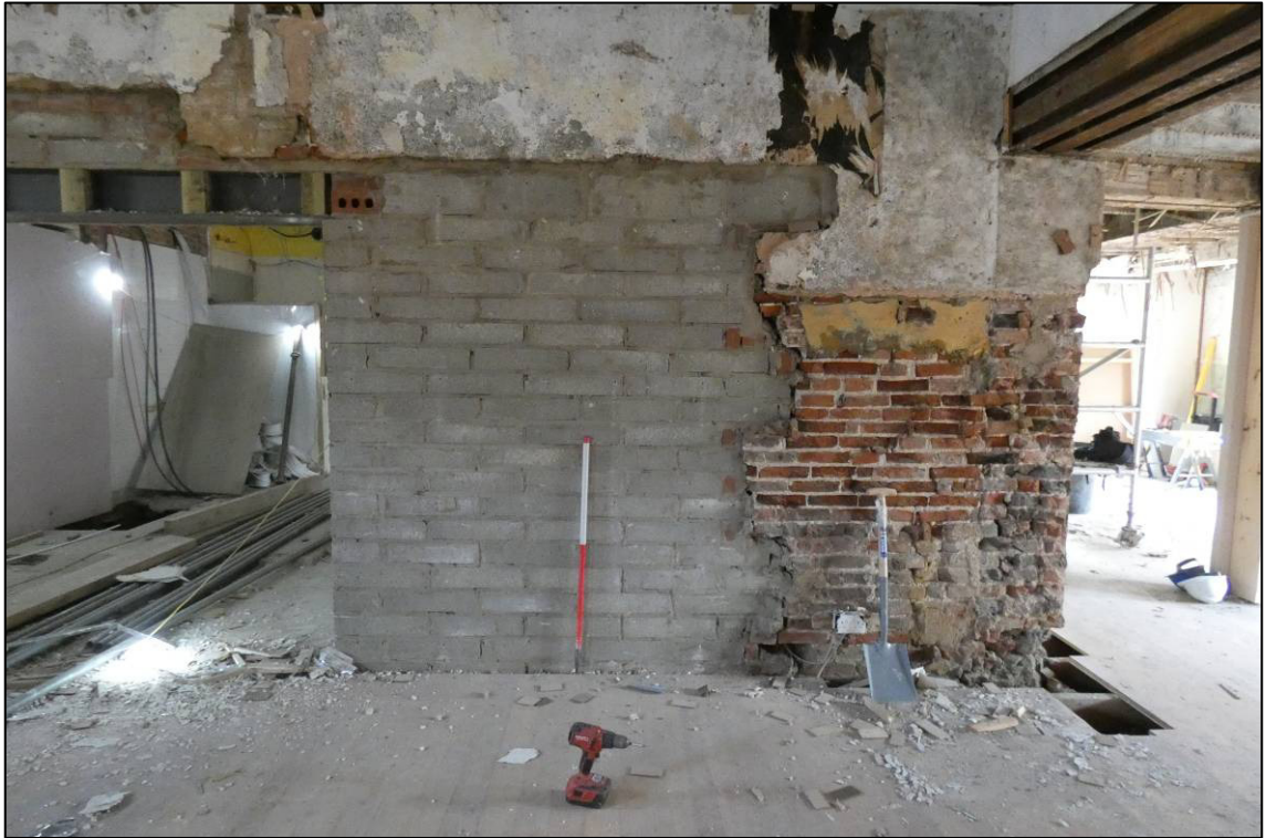
Plate 50: South range, ground floor room (GF9 - cafe) during alterations, showing modern blocking to east wall, looking NE (photo 4/785).
