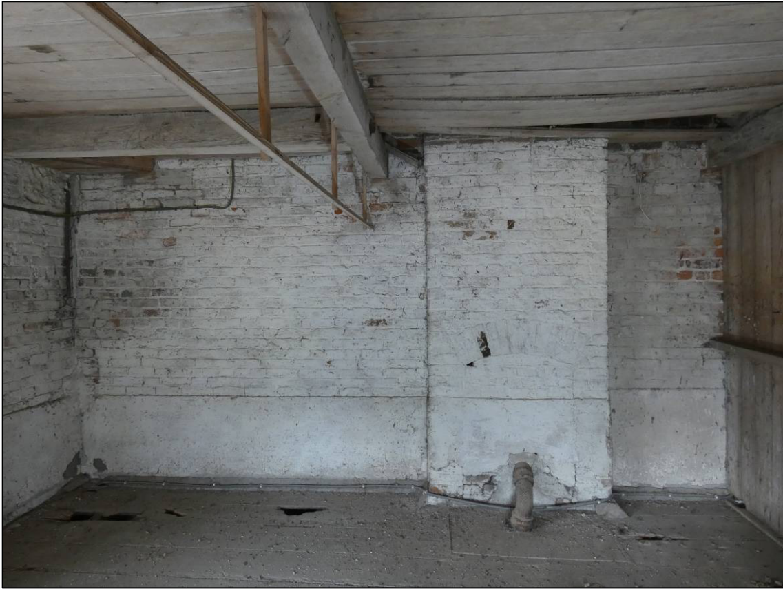
Plate 82: South range, first floor room (1F11), blocked fireplace to north wall, looking NW (photo 1/818).
