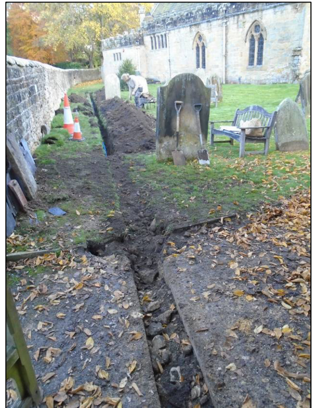
Plate 3: Excavation of fresh water pipe trench, looking E showing cut through path.
