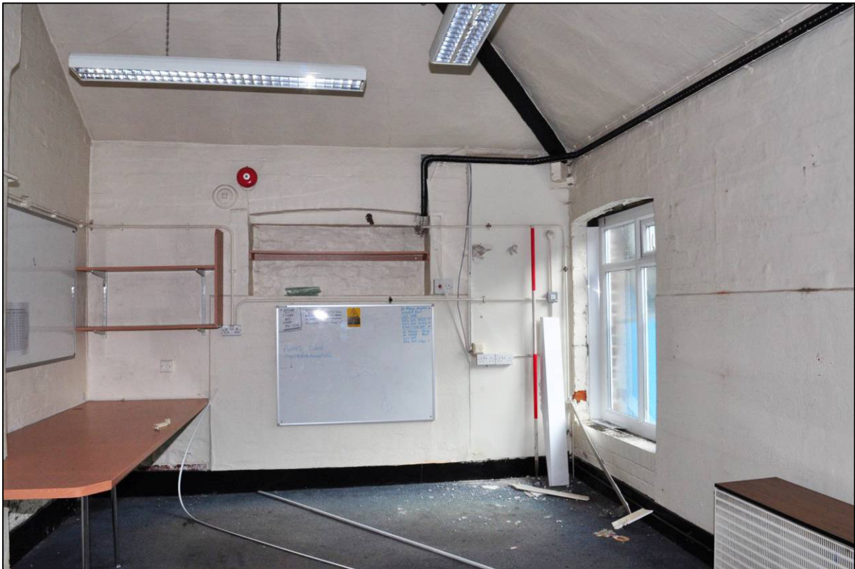
Plate 61: East range, original part, room G18, blocked window to east wall, looking E (photo 1/2897).
