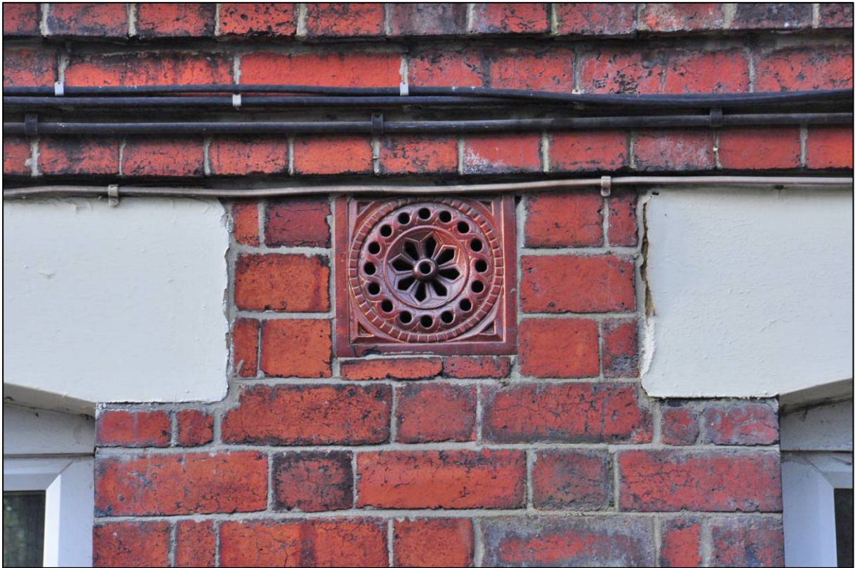
Plate 24: Entrance Block, west end of south elevation, vent detail, looking N (photo 1/3030).
