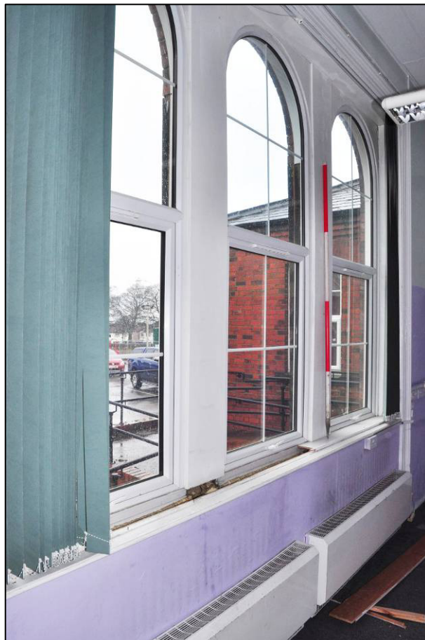
Plate 50: Entrance Block, room G14 (former Board Room), windows in north wall, looking NE (photo 1/2862).
