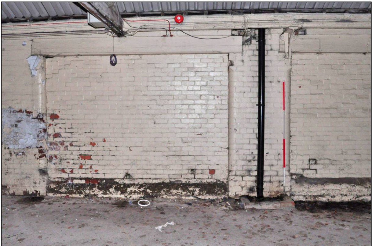
Plate 72: East range, eastern extension, room G22, blocked cart entrances to west side of original part, looking W (photo 1/2895).
