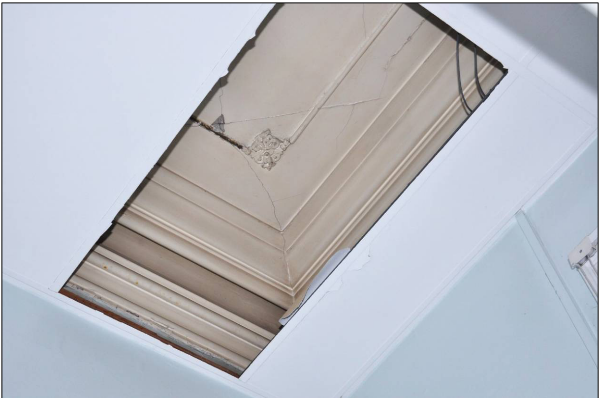
Plate 52: Entrance Block, room G14 (former Board Room), ceiling cornice, looking NW (photo 1/2863).
