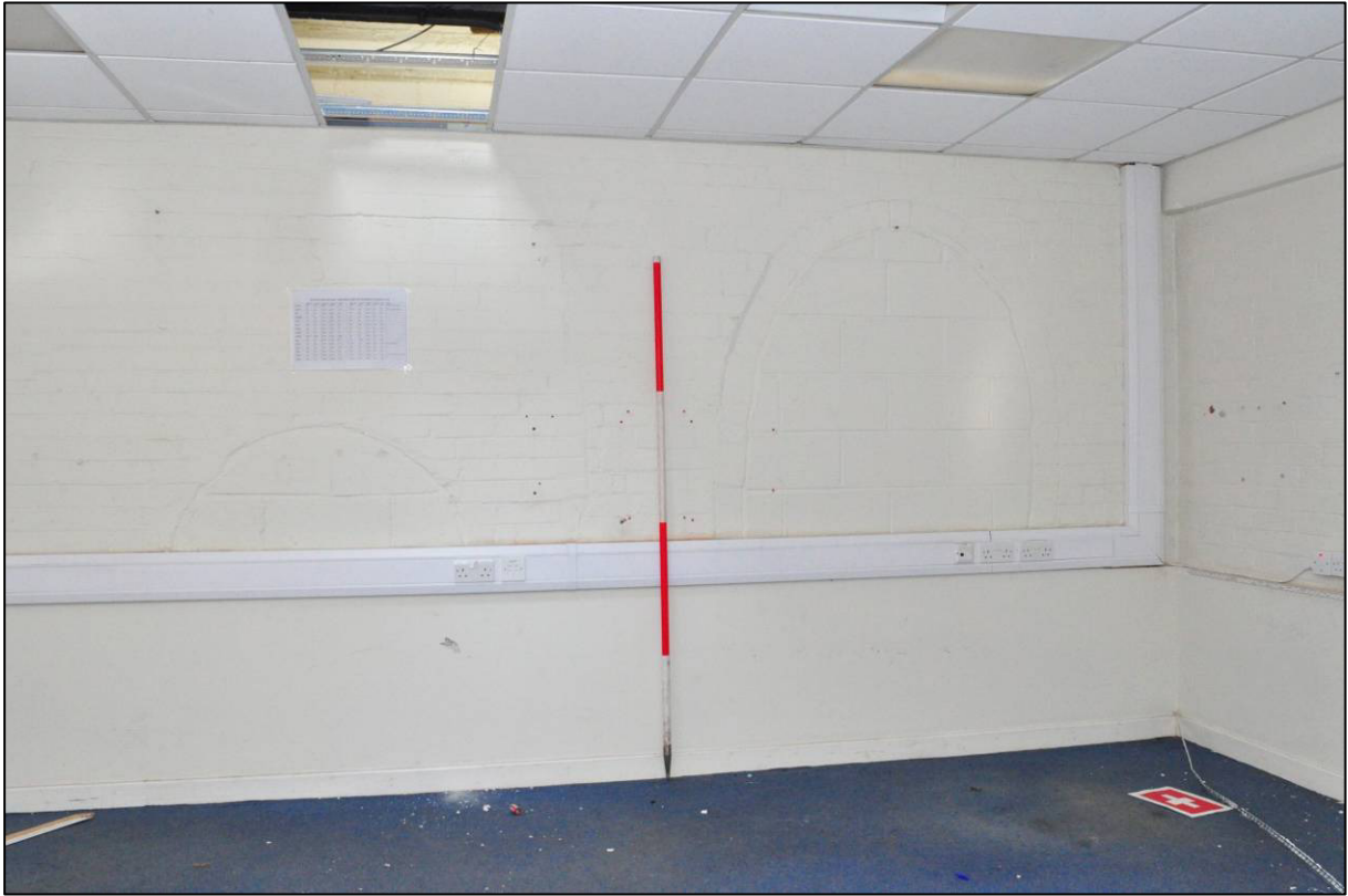
Plate 65: East range, original part, room G20, blocked openings to north wall, looking N (photo 1/2902).
