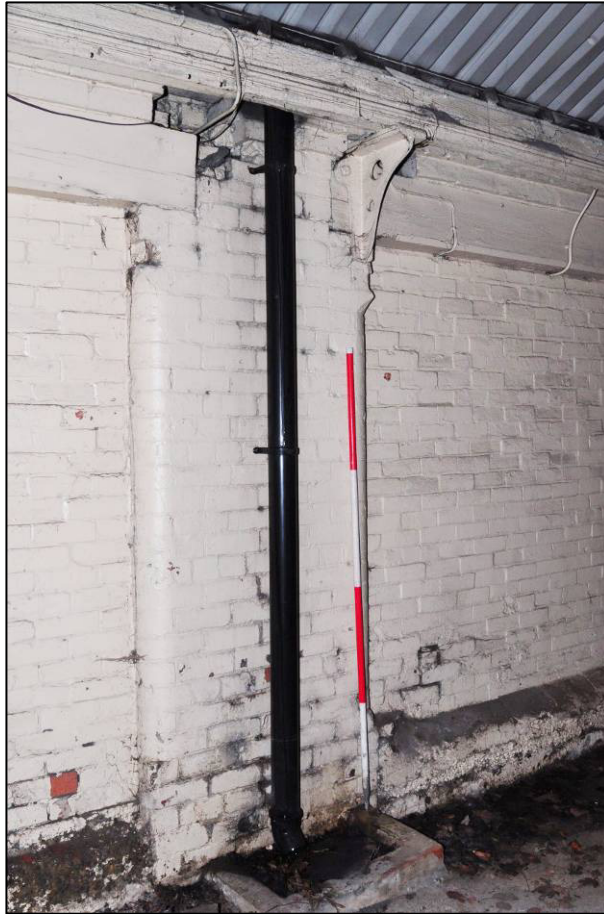
Plate 71: East range, eastern extension, room G22, cast-iron bracket supporting west wall plate, looking NW (photo 1/2893).
