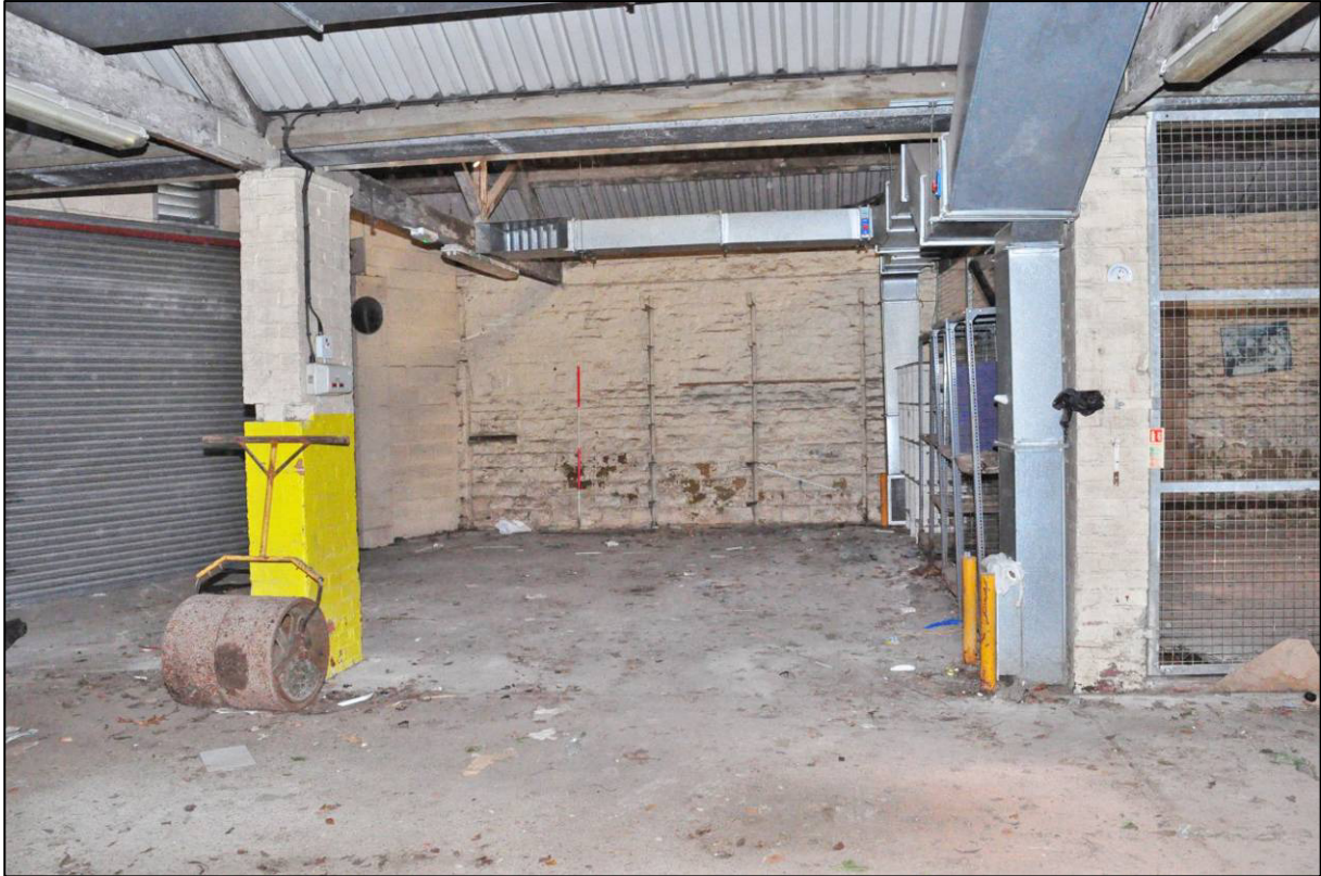
Plate 73: East range, eastern extension, room G22, showing earlier boundary wall, looking E (photo 1/2896).
