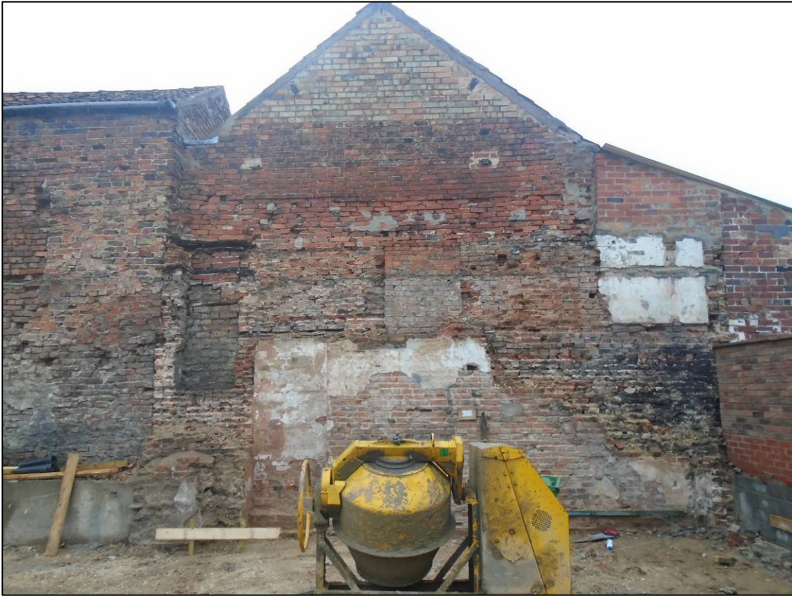
Plate 5: Gable end of Nos. 1-6 Lockwood Court, showing blocked openings, after demolition of cottage, looking NE.
