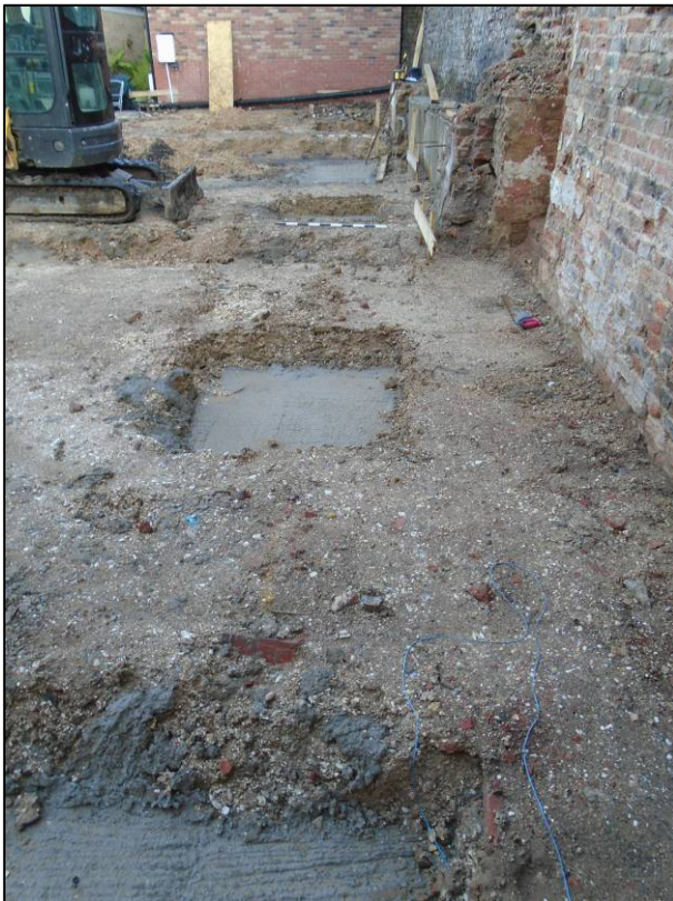
Plate 10: Piecemeal development of back wall foundation, looking N.
