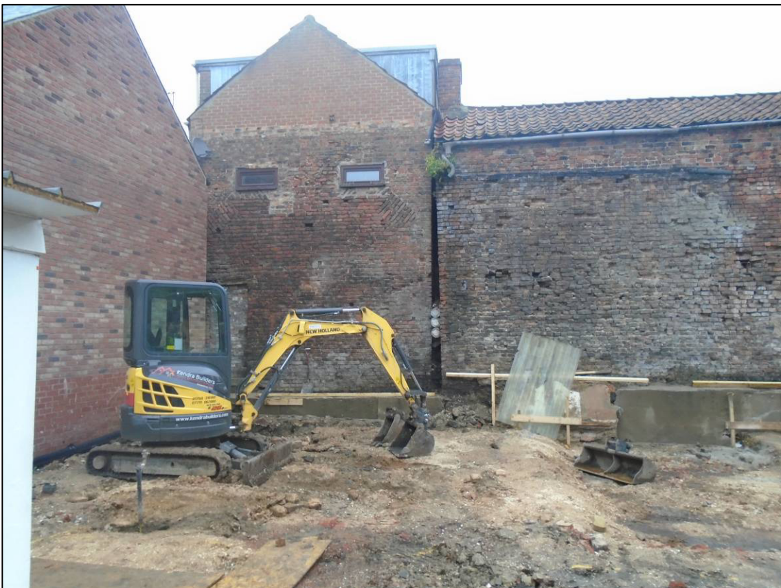
Plate 4: Gable end of No. 2a Lockwood Court, showing tumbled brickwork of former roof line, after demolition of cottage, looking NE..
