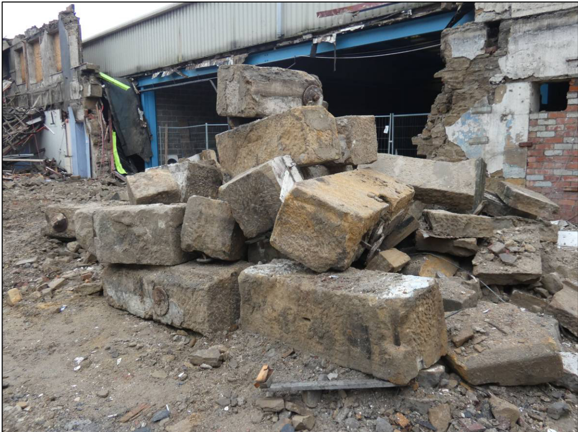
Plate 56: Ilkley Road frontage during demolition, ashlar band from c.1857 original part (Unit G), looking NW (photo 3648).
