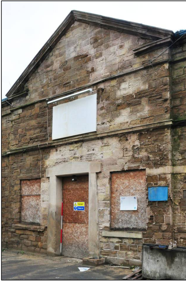
Plate 43: Ilkley Road frontage, c.1857 original part (Unit G), central entrance and pediment, looking N (photo 11737).
