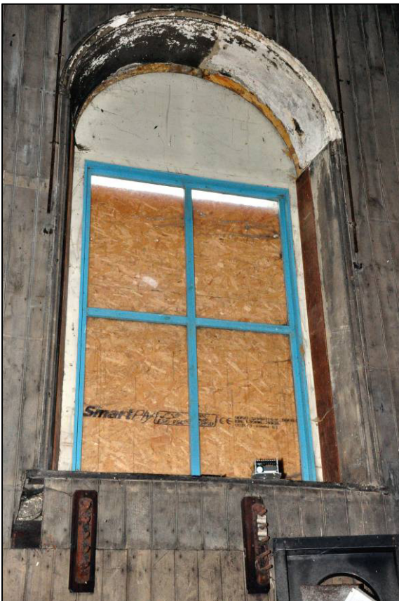
Plate 22: Southern engine house, ground floor, western window in south wall, looking S (photo 11840).
