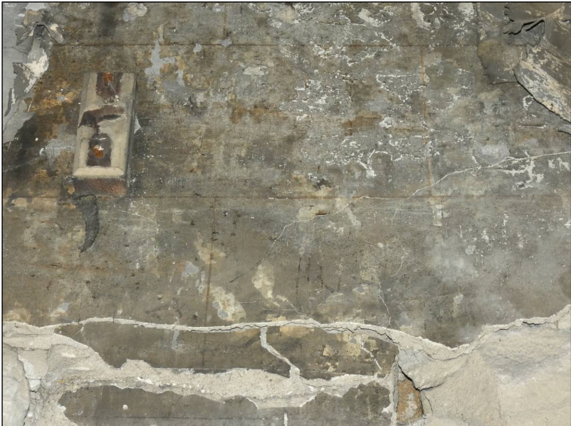
Plate 31: Southern engine house, ground floor after stripping out, painted decoration at upper level of north wall, looking N (photo 2394).
