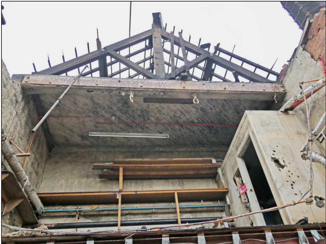
Plate 53: Northern engine house during demolition, southernmost roof truss with lifting rings, looking S (photo 3640).
