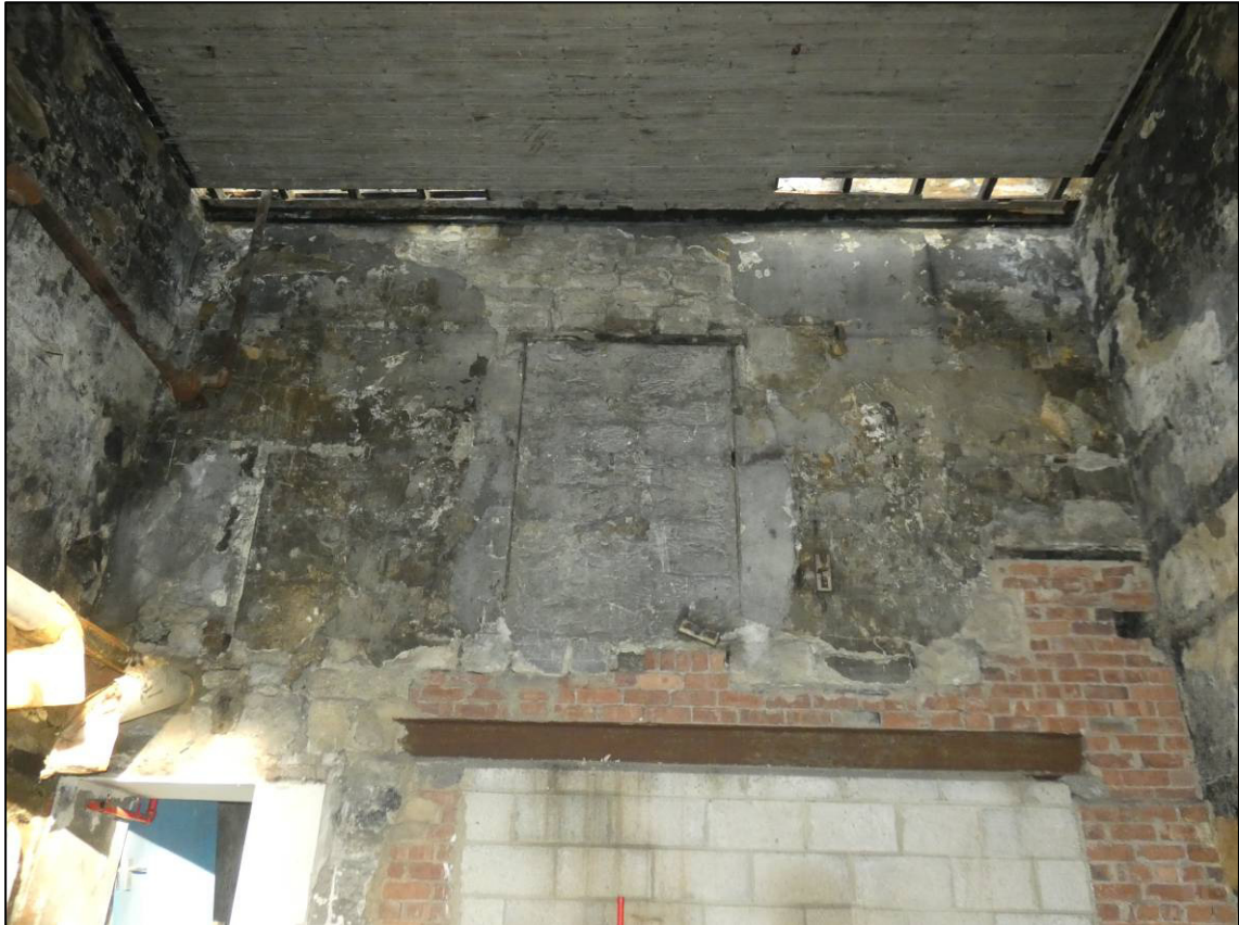
Plate 30: Southern engine house, ground floor after stripping out, blocked window in north wall, looking N (photo 2352).
