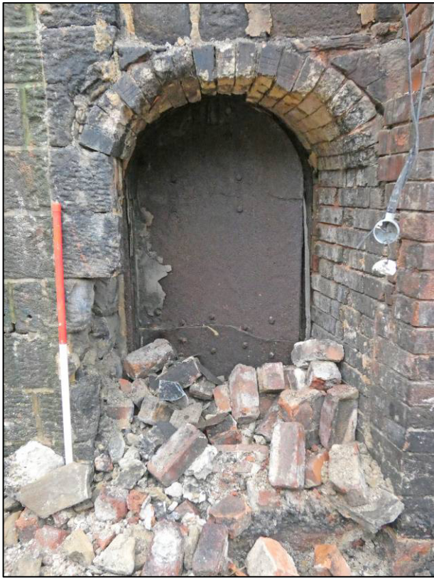
Plate 50: Boiler house, ground floor opening at east end of north gable, revealed after demolition of economiser house, looking S (photo 3632).
