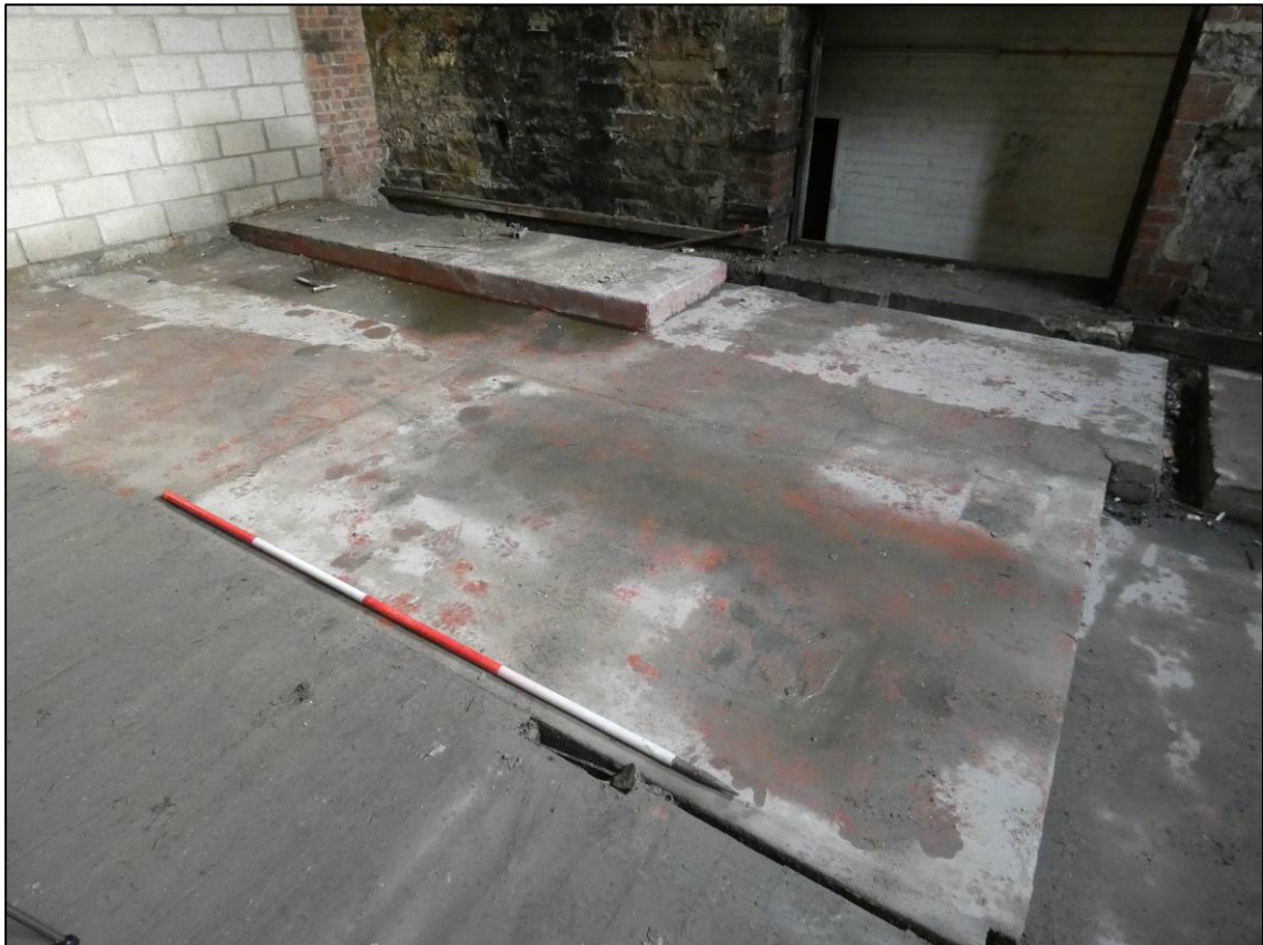
Plate 26: Southern engine house, ground floor after stripping out, secondary bed, looking NE (photo 2382).
