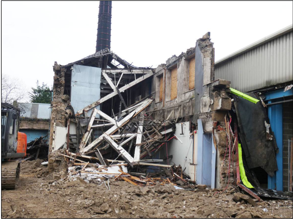
Plate 55: Ilkley Road frontage during demolition, c.1857 original part (Unit G), looking W (photo 3645).
