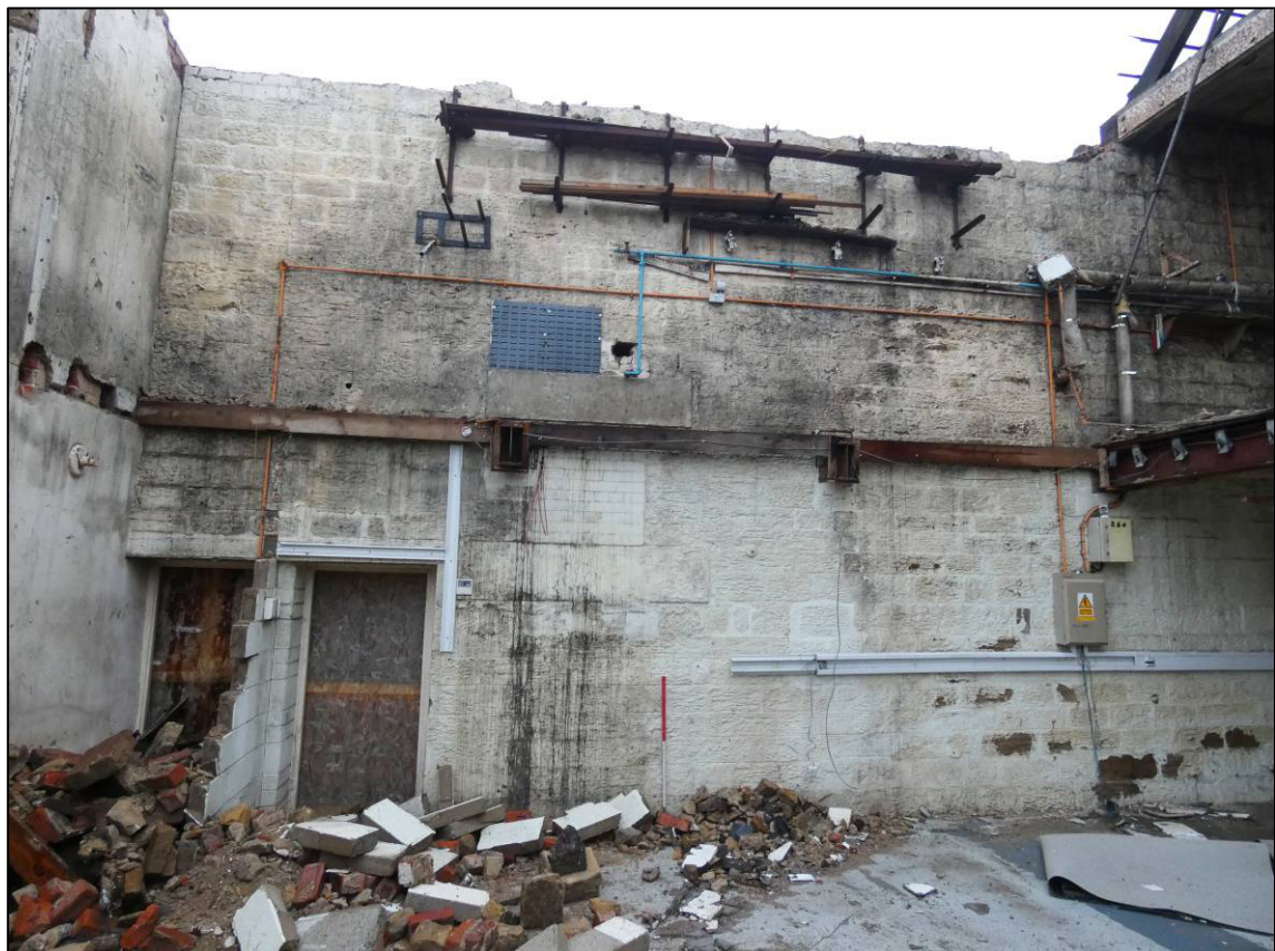
Plate 52: Northern engine house during demolition, north end of east wall, looking E (photo 3638).
