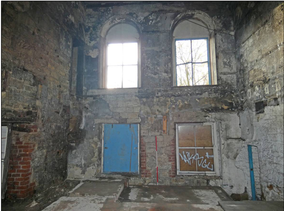
Plate 29: Southern engine house, ground floor after stripping out, south wall, looking S (photo 2369).
