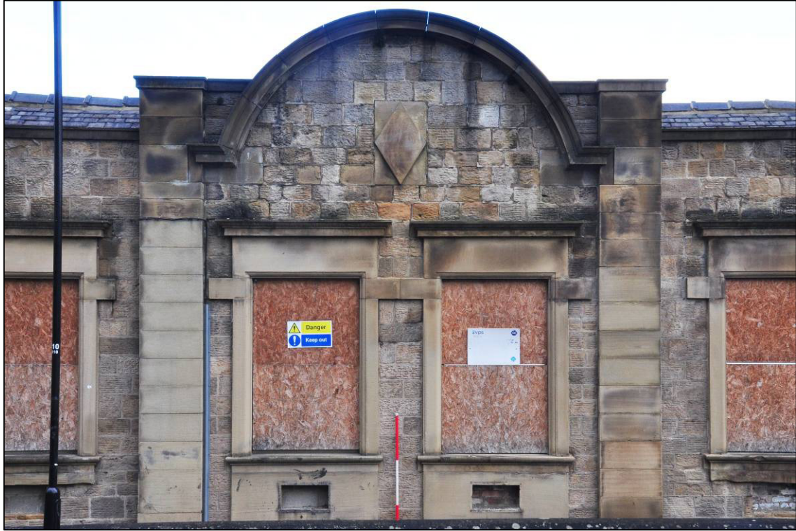
Plate 46: Ilkley Road frontage, 1891-1908 extension (Unit D), detail of central pediment, looking N (photo 11726).
