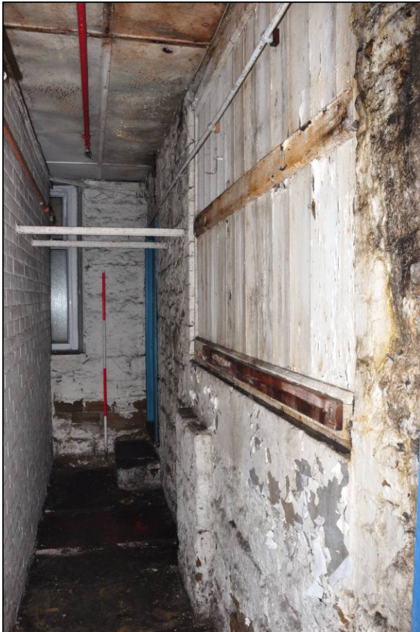
Plate 18: Southern engine house, lower east elevation revealed in north-south passage, looking S (photo 11808).
