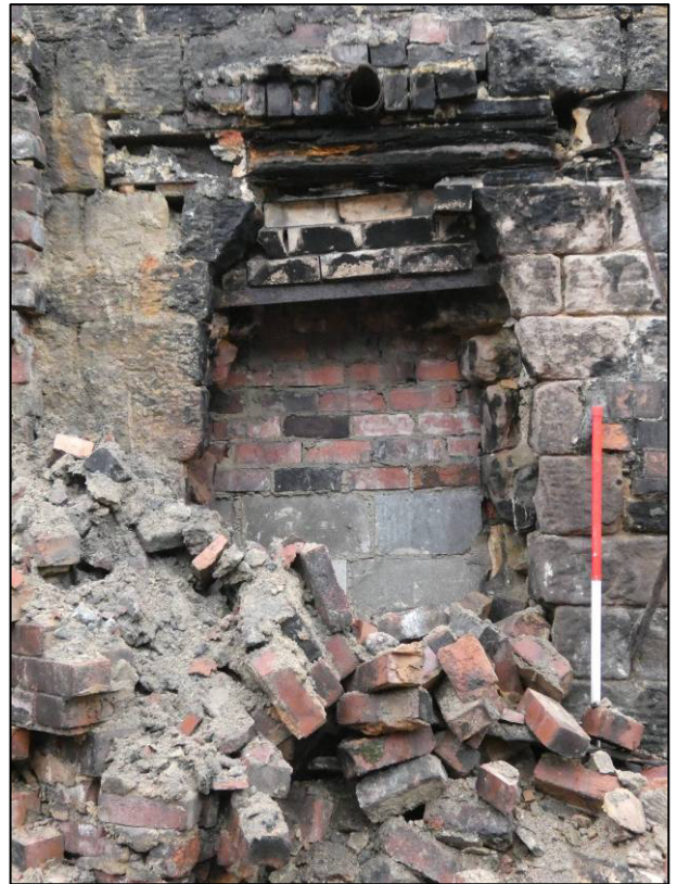
Plate 51: Boiler house, ground floor opening at west end of north gable, revealed after demolition of economiser house, looking S (photo 3629).
