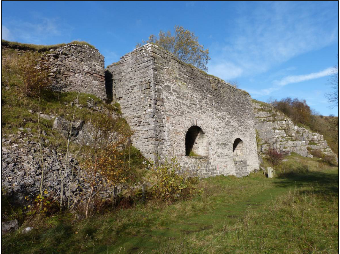
Plate 1: East elevation of Smardale kilns with railway track bed, looking NW (photo 1/004).
