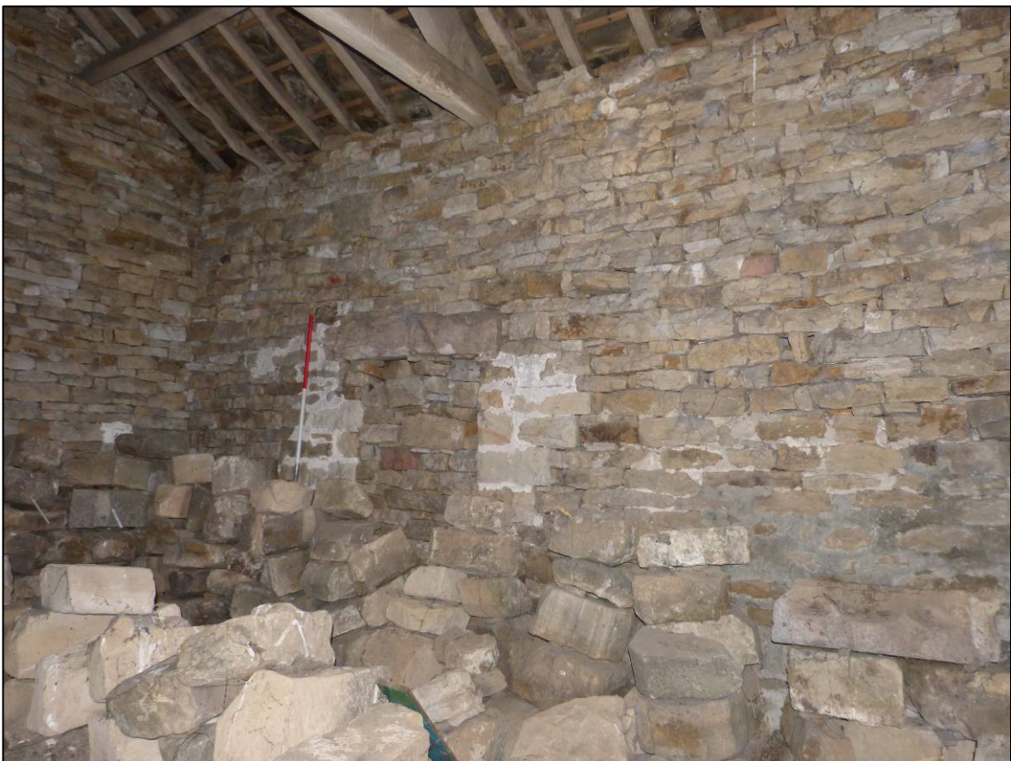
Plate 70: Pendragon Castle barn, interior showing east wall and stored stonework, looking NE (photo 4/228).
