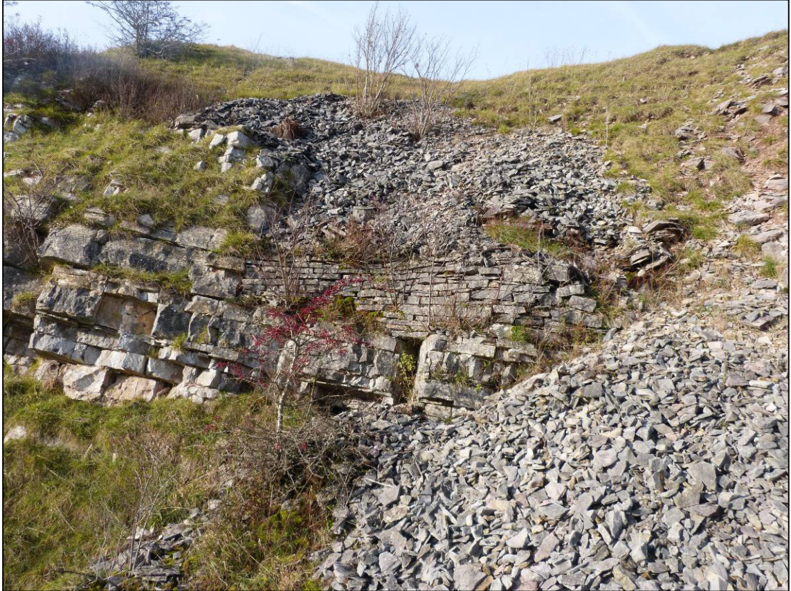
Plate 20: Smardale quarry, retaining wall at north end of quarry (Site 103), looking W (photo 2/120).
