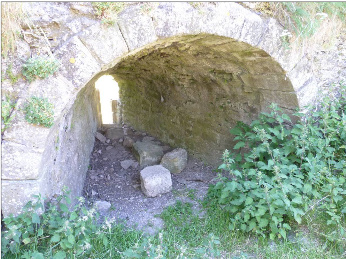
Plate 85: Pendragon Castle, interior, rubble in south window of west wall, looking W (photo 10/180).
