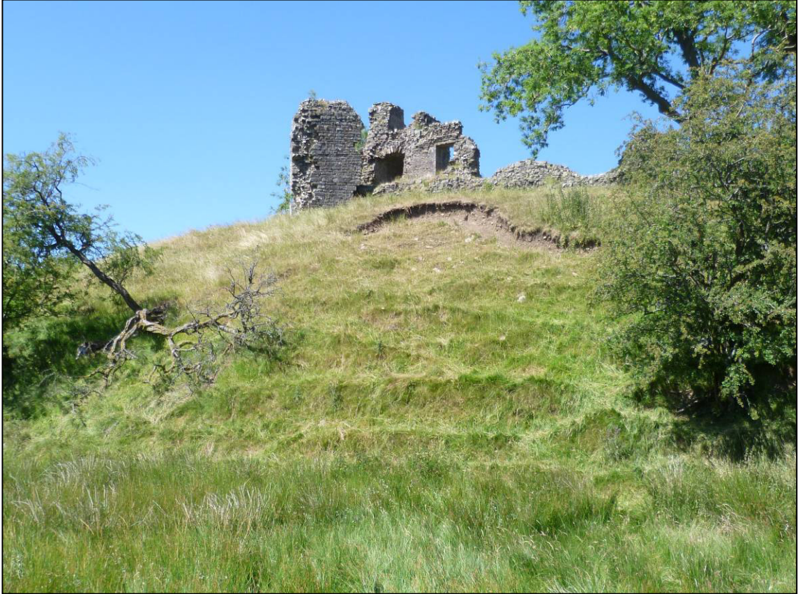
Plate 75: Pendragon Castle, slumping scar and slippage below (Areas 7 and 9) on south side of castle mound (201), looking NW (photo 10/174).
