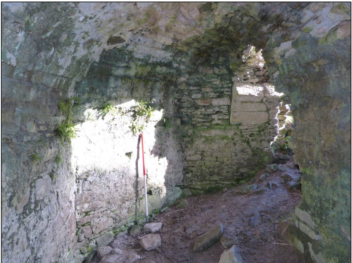
Plate 59: Pendragon Castle, interior of north-west chamber showing angled wall, looking E (photo 9/584).
