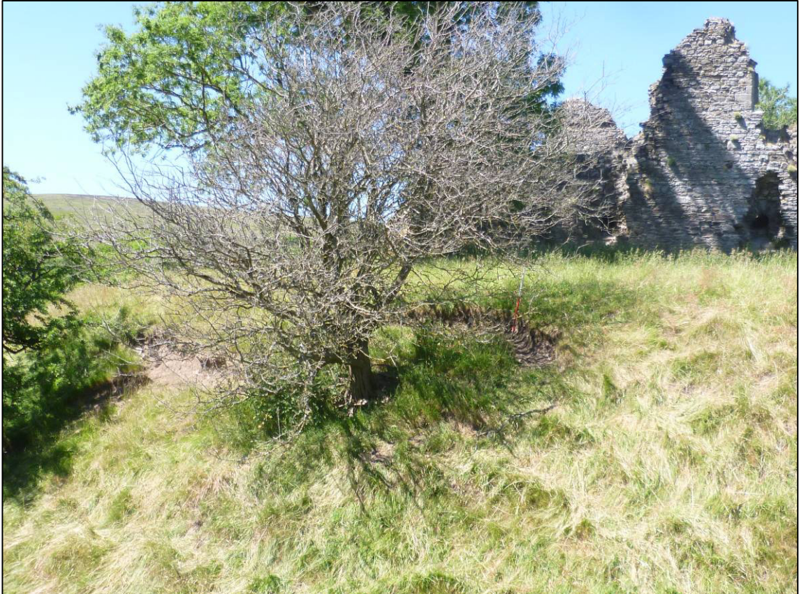
Plate 77: Pendragon Castle, slumping scars (Areas 1 and 2) on south-east side of castle mound (201), looking NW (photo 10/114).
