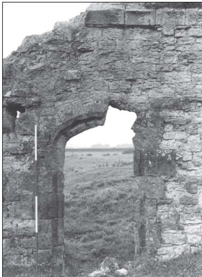
Plate 2: Detail of doorway in east elevation, prior to consolidation, looking W (photo 1/18).
