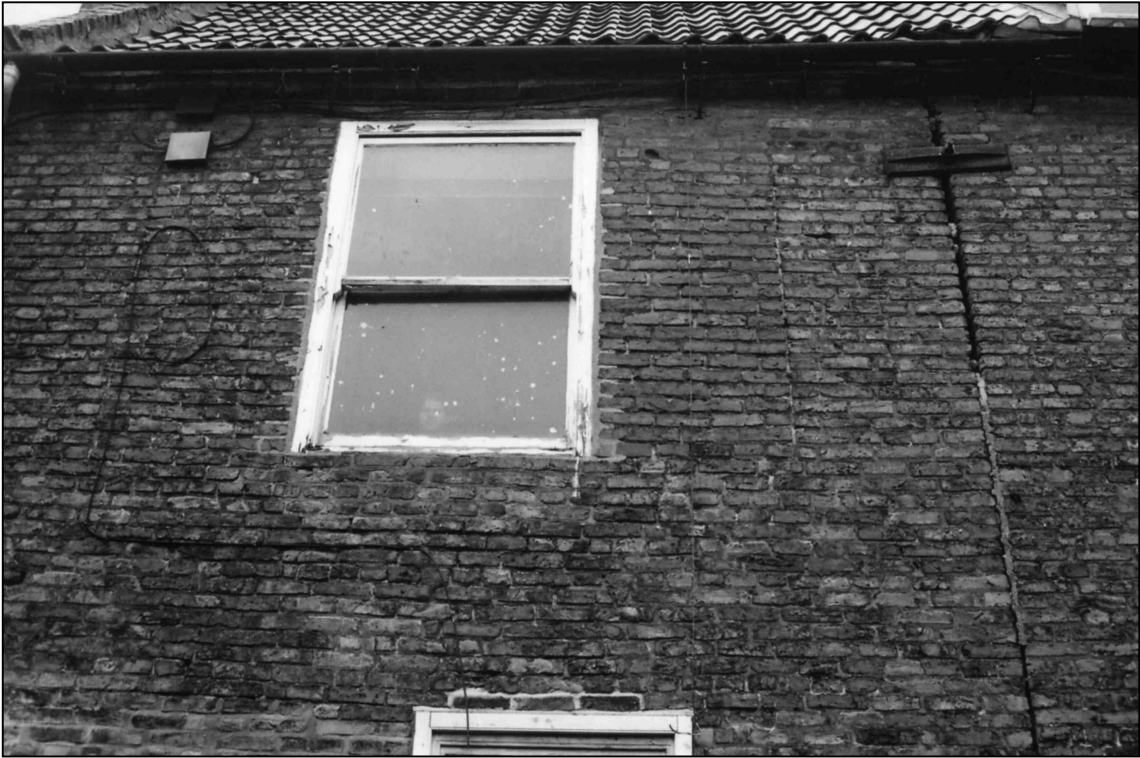
Plate 4: Blocking to first floor window, south elevation of Building B, looking N (photo 2/5).
