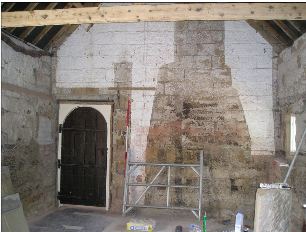
Plate 8: North side of south range (B1) showing scarring of former flue and altered doorway (photo 83).
