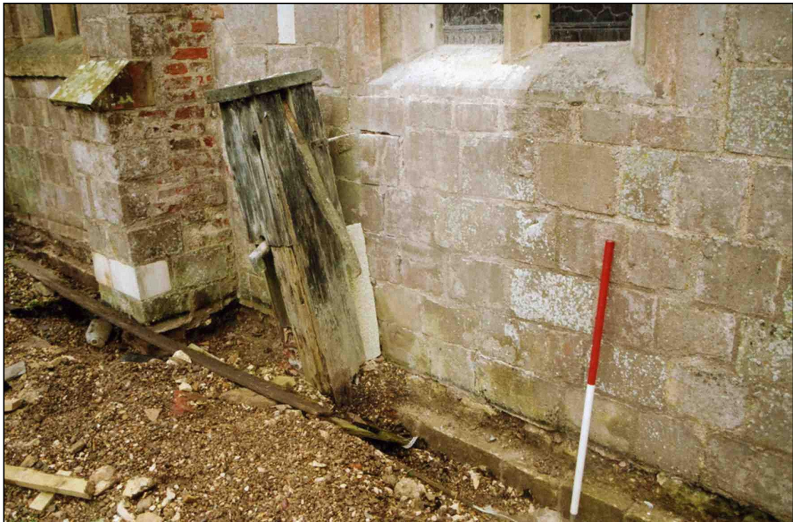
Plate 3: Central part of north aisle showing old pump and cleaned out French drain, looking SE.
