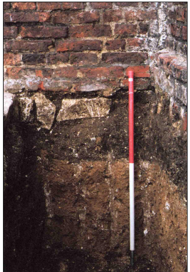
Plate 4: Chalk foundation (013) at SE corner of house, with plinth and foundation (024) of east garden wall to right, looking N.
