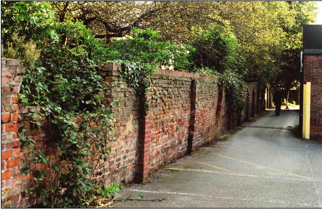
Plate 1: General view of wall 012 prior to demolition, from car park looking north-east.
