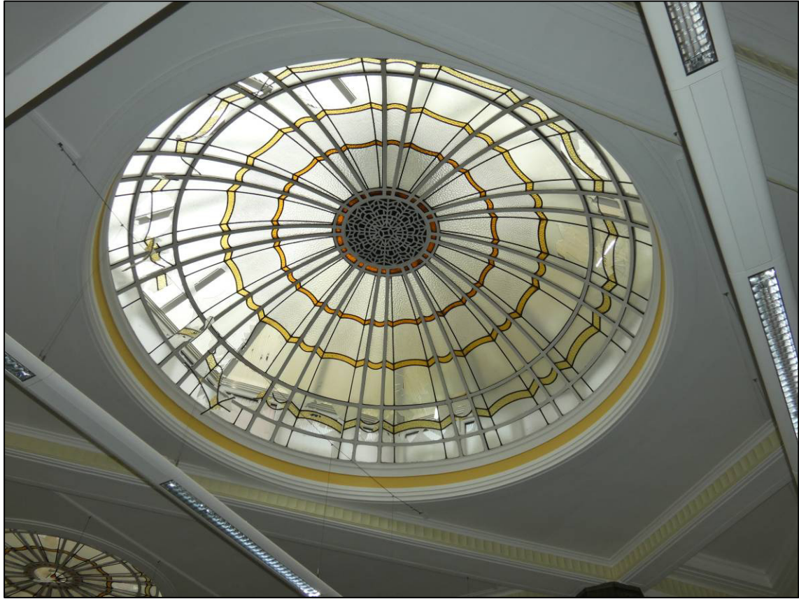
Plate 37: Banking hall and general office (GF2), domed central skylight, looking NW (photo 882).
