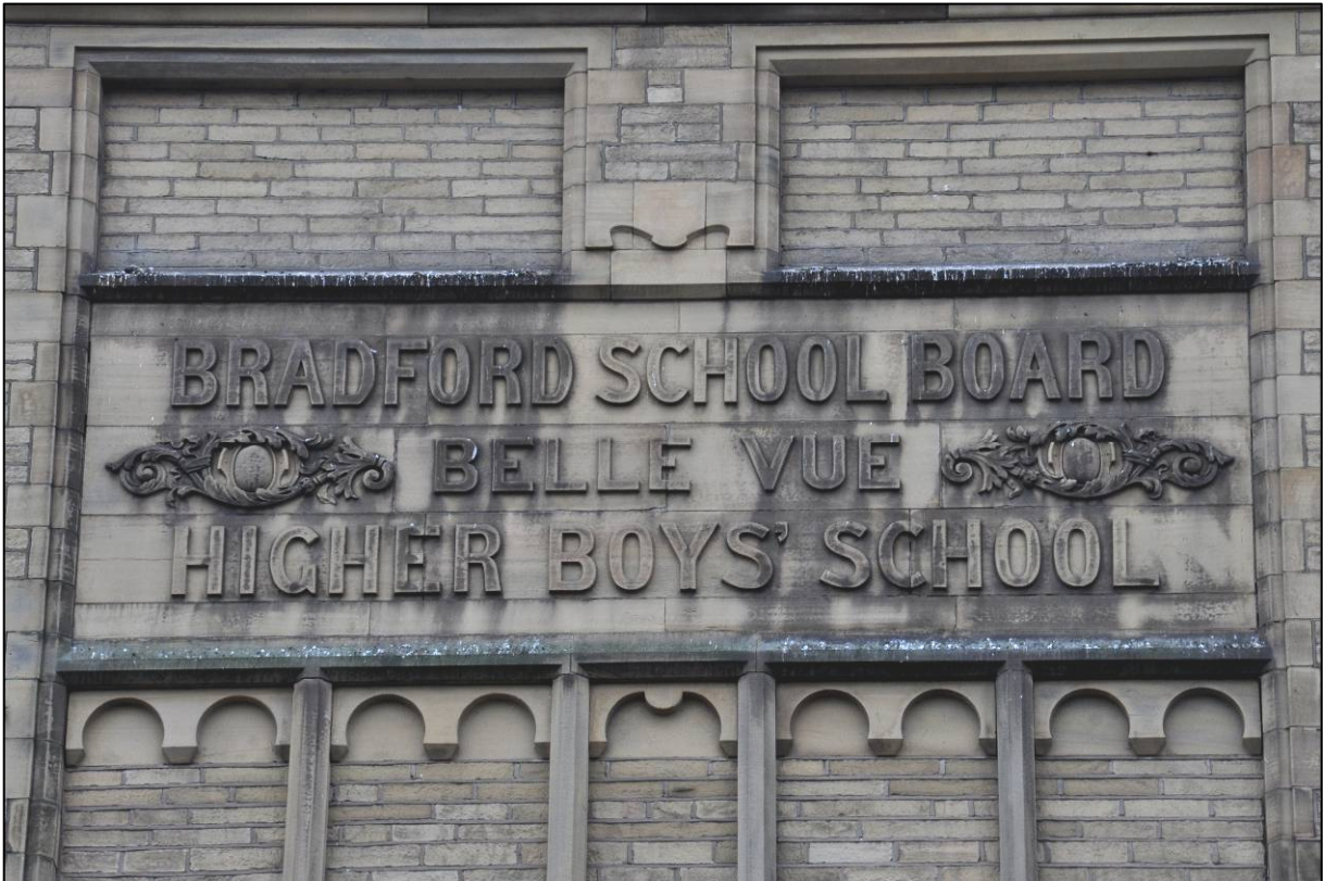
Plate 54: 1895 Higher Grade Boys' School, east elevation, plaque/panel to southern two bays, looking W (photo 2118).
