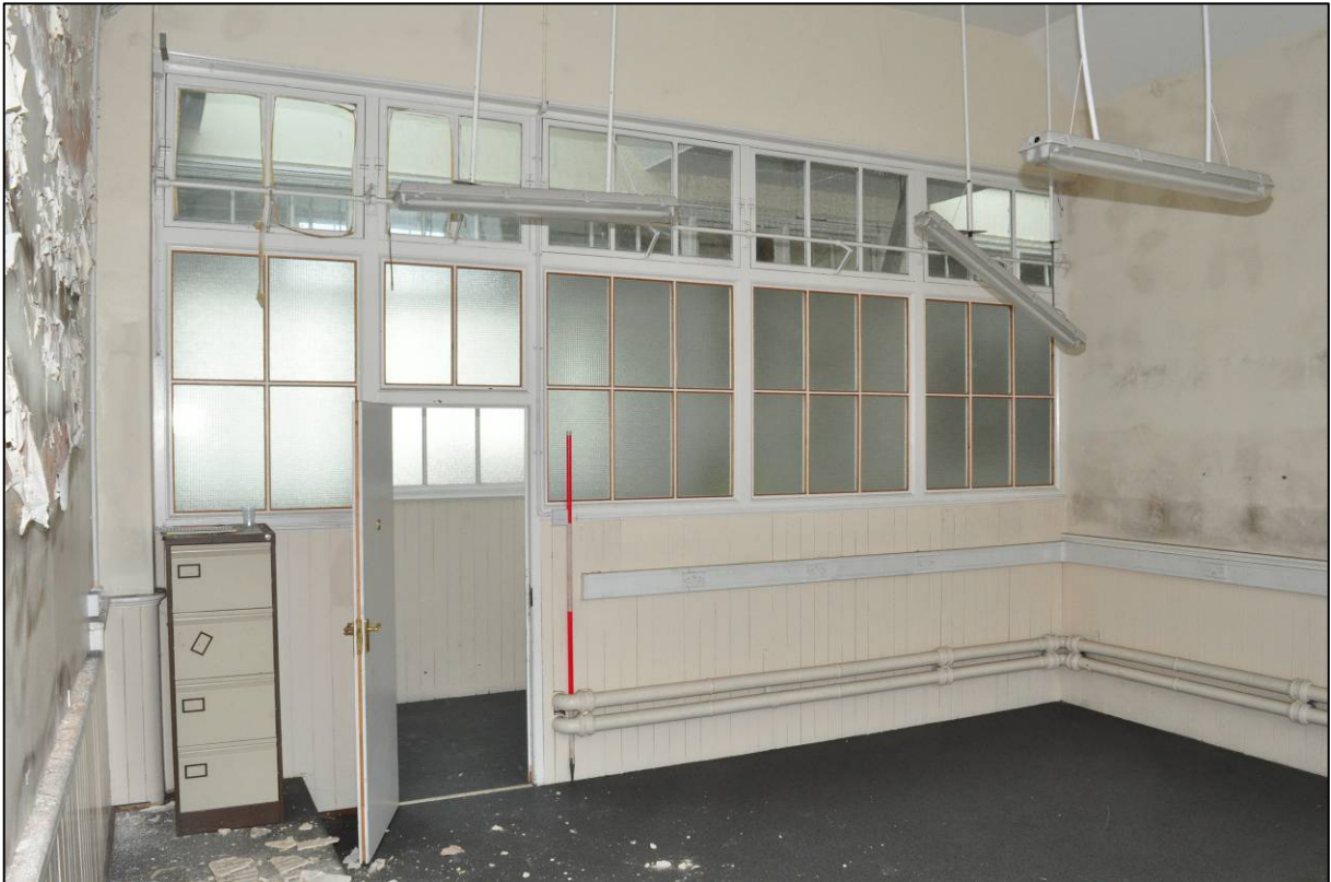
Plate 118: 1908 Higher Grade Girls' School, classroom (2F19), windows to north wall, looking S (photo 2493).
