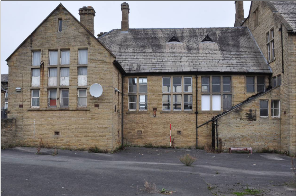
Plate 12: 1879 Board School, south elevation of girls' block, with later external pentice-type stair, looking N (photo 2180).
