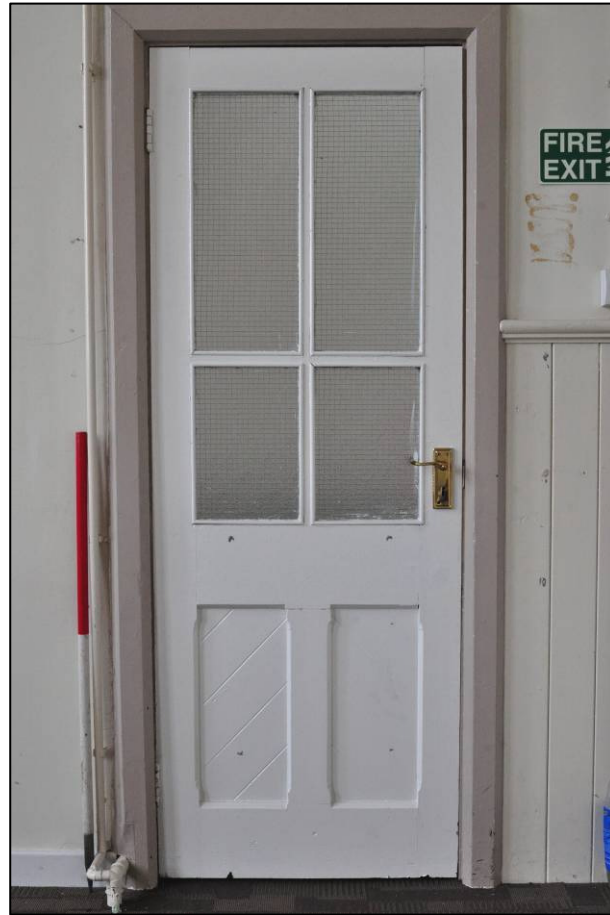
Plate 94: 1895 Higher Grade Boys' School, prep room (2F6), door to north wall, looking N (photo 2319).
