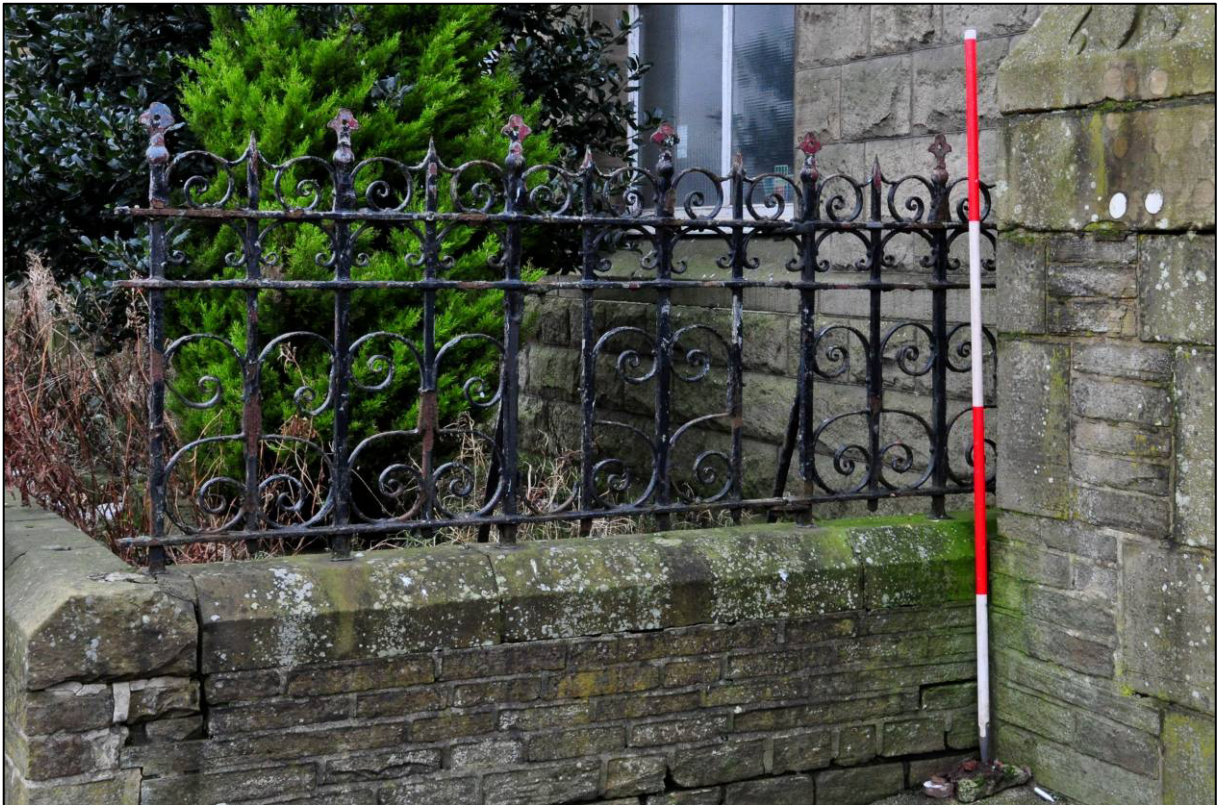
Plate 3: 1895 Higher Grade Boys' School, east elevation, original cast-iron railings adjacent to north yard gates, looking S (photo 2141).
