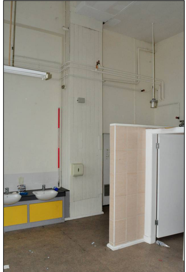
Plate 72: 1895 Higher Board Boys' School, changing room (1F12), heating vent to north wall, looking NE (photo 2237).
