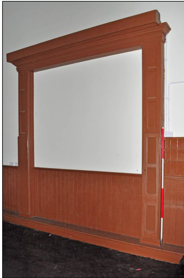
Plate 90: 1895 Higher Grade Boys' School, lecture theatre (2F5), blackboard surround to west wall, looking SW (photo 2312).
