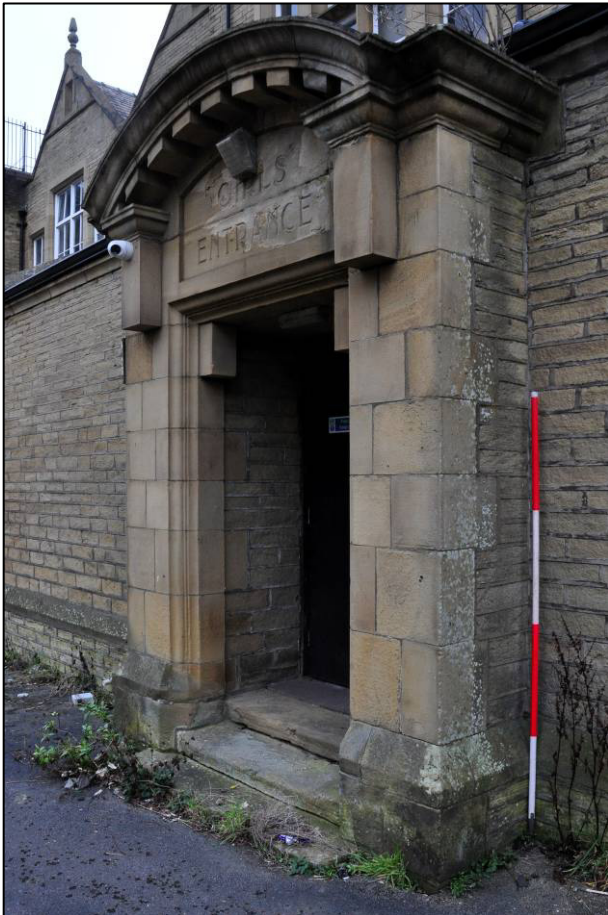
Plate 8: 1908 extension to Higher Grade Girls' School, girls' entrance to north elevation, looking SE (photo 2188).
