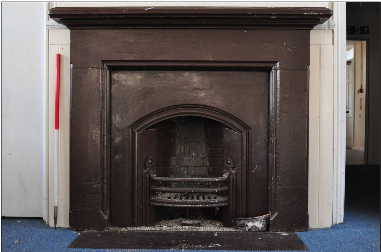
Plate 33: 1879 Board School, girls' hall (GF4), fireplace to west wall, looking W (photo 2456).
