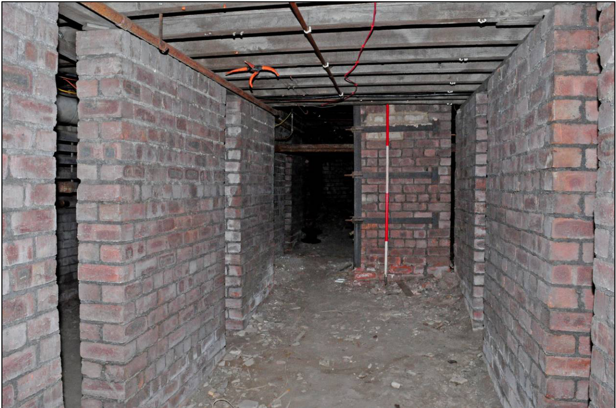
Plate 18: 1879 Board School, basement, typical underfloor void to north of B4, looking W (photo 2376).
