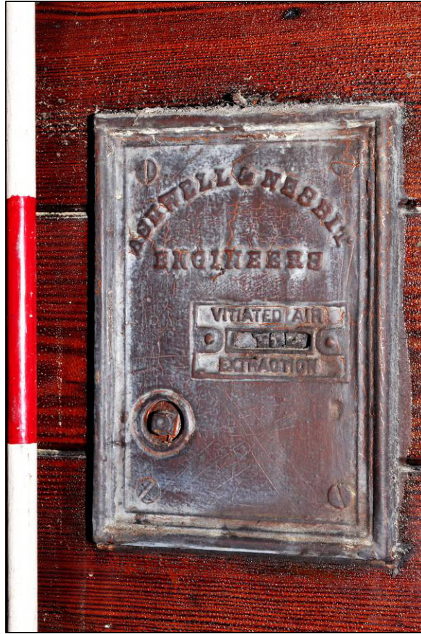
Plate 84: 1895 Higher Grade Boys' School, classroom (2F8), maker's plate on southern ventilation duct to east wall, looking E (photo 2344).
