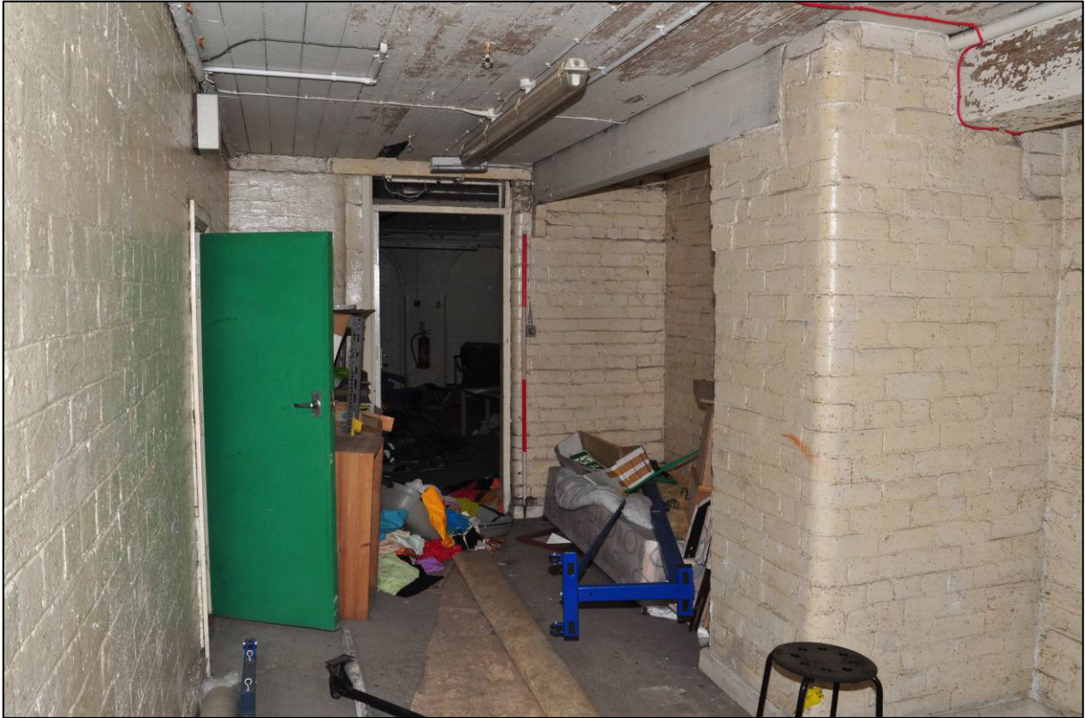
Plate 16: 1879 Board School, former boys' covered playground (B4), now store, looking E (photo 2375).
