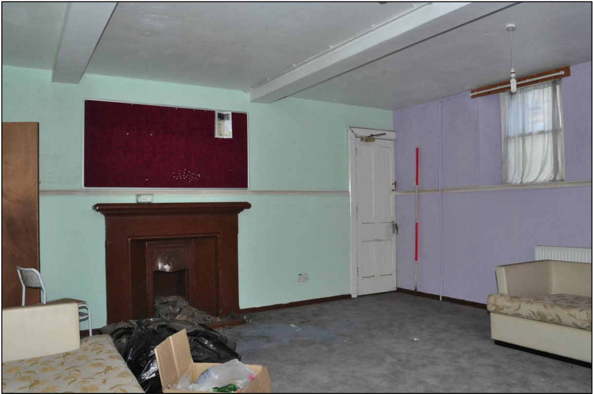
Plate 39: 1879 Board School, girls' classroom (GF1), fireplace, dado rail and door to south wall, looking SW (photo 2460).
