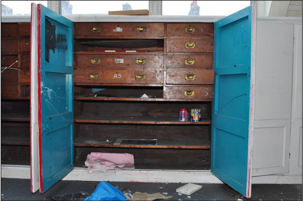
Plate 120: 1908 Higher Grade Girls' School, classroom (2F23), cupboard to north wall, looking N (photo 2503).
