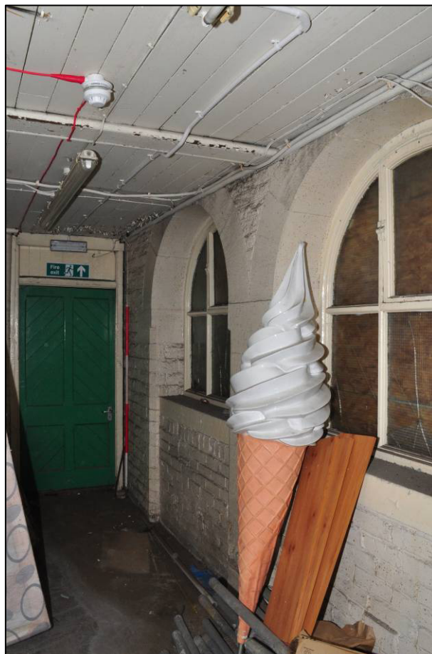
Plate 17: 1879 Board School, former boys' covered playground (B5), now store, looking E (photo 2377).
