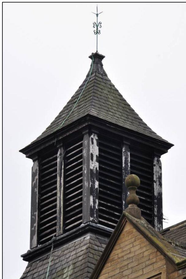
Plate 55: 1895 Higher Grade Boys' School, east elevation, timber roof vent, looking SW (photo 2124).
