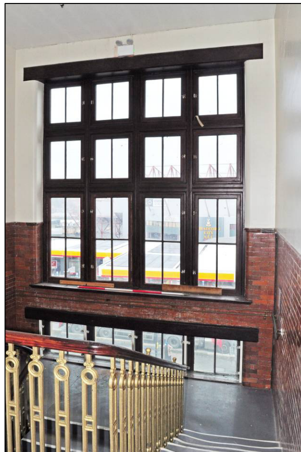
Plate 80: 1895 Higher Grade Boys' School, stair hall (2F1), window to east wall, looking E (photo 2288).
