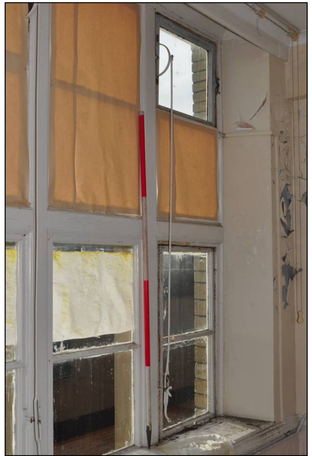
Plate 110: c.1897-99 Higher Grade Girls' School, classroom/cookery room (1F25), opening mechanism to window in south wall, looking SW (photo 2396).
