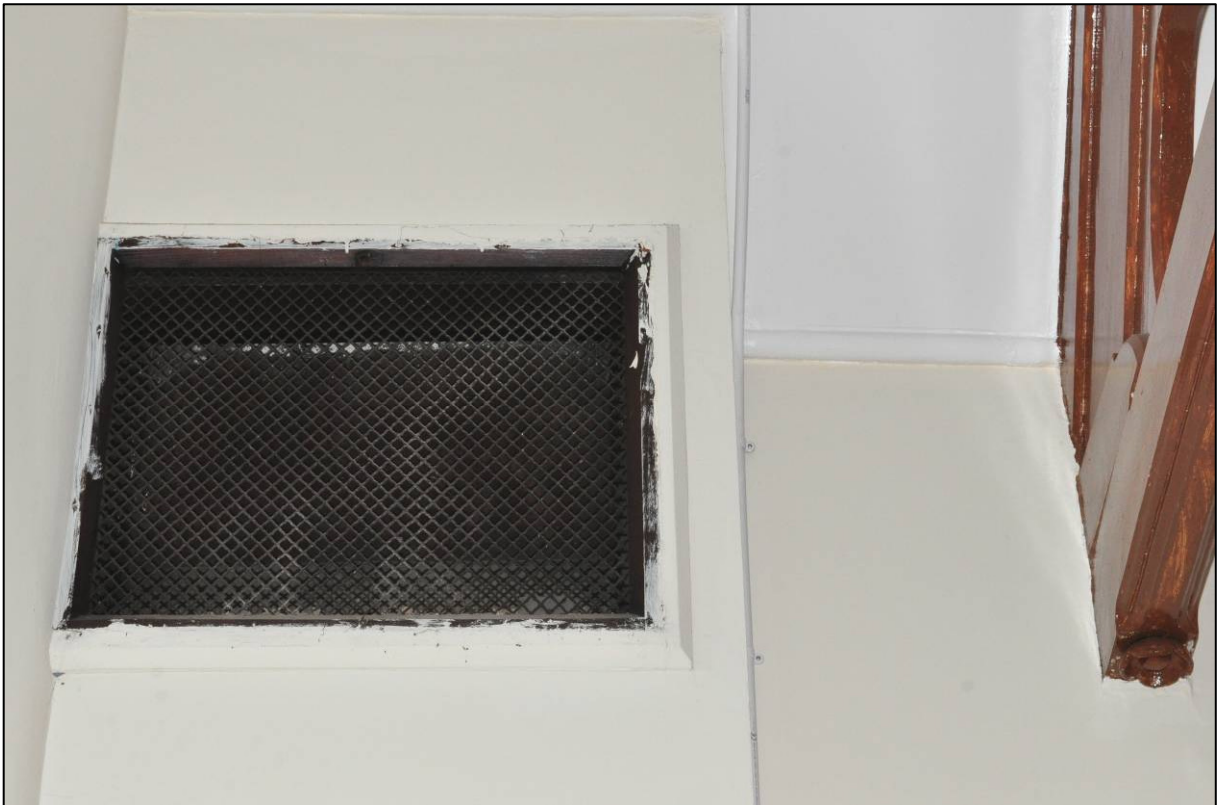
Plate 97: 1895 Higher Grade Boys' School, classroom (2F13), vent grille to south wall, looking S (photo 2350).
