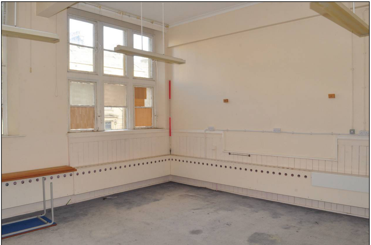
Plate 106: c.1897-99 Higher Grade Girls' School, classroom (1F19), original features, looking NE (photo 2400).
