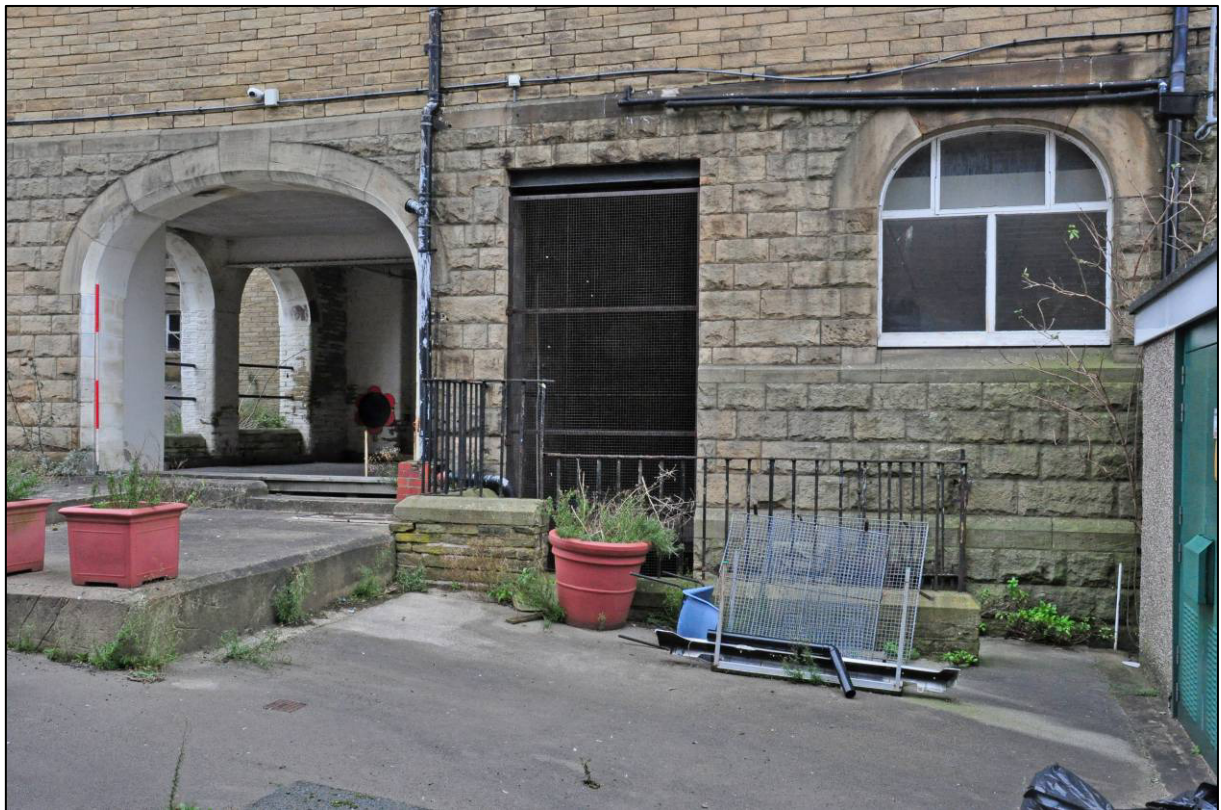
Plate 57: 1895 Higher Grade Boys' School, south elevation, entrance to basement, looking NW (photo 2197).
