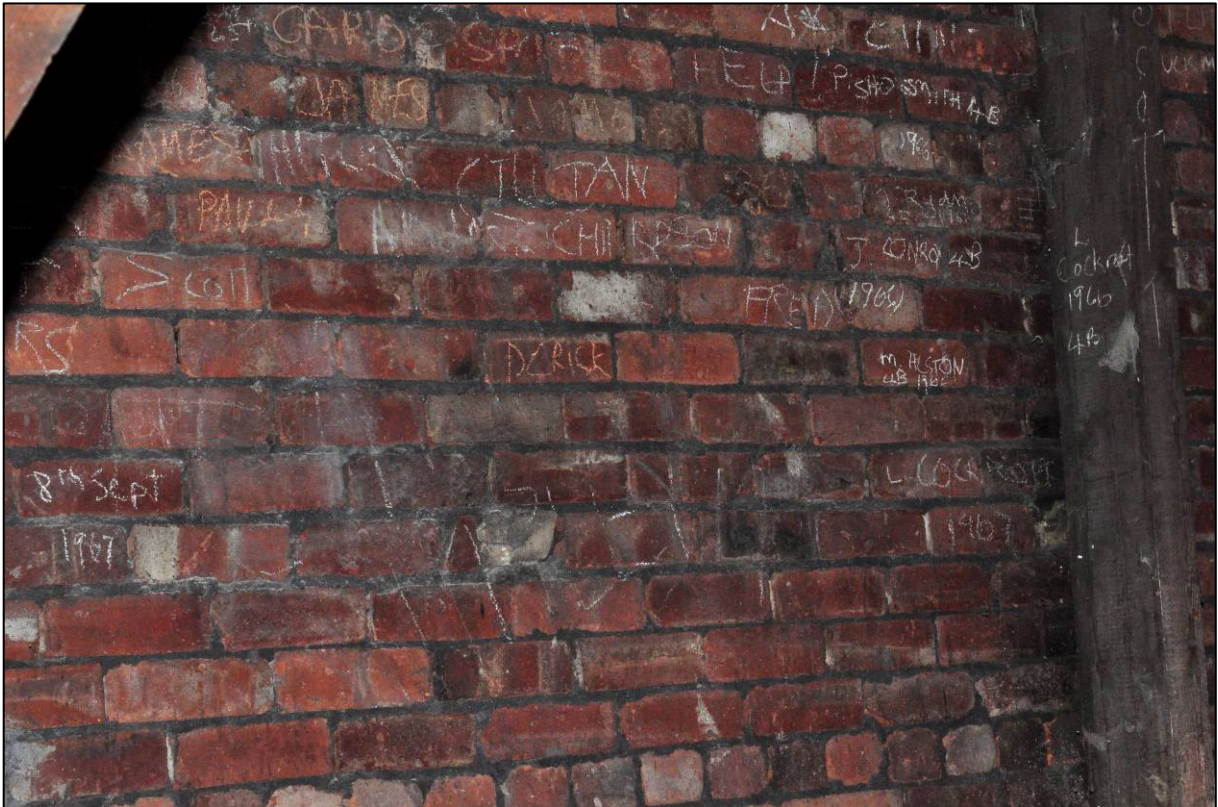
Plate 86: 1895 Higher Grade Boys' School, lecture theatre (2F5), chalked graffiti to space under seating, looking SE (photo 2324).
