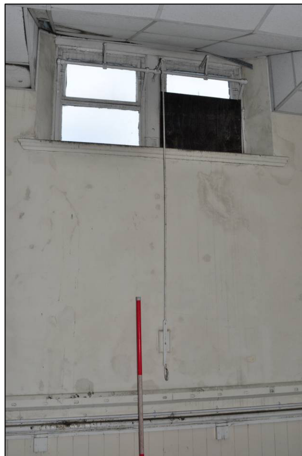
Plate 42: 1879 Board School, science classroom (1F5), opening mechanism to window in west wall, looking W (photo 2474).
