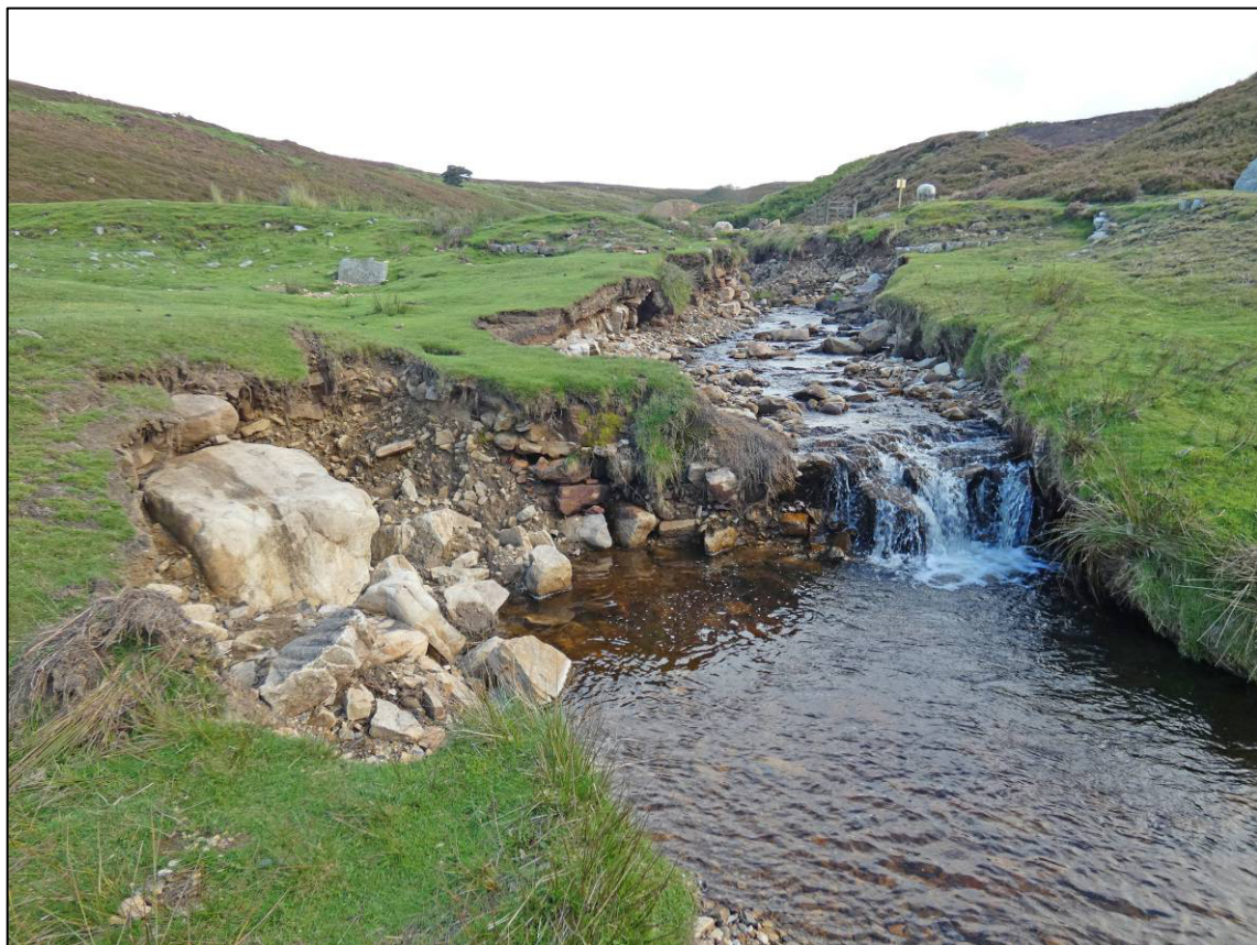
Plate 17: Flood damage to beck between dam and smelt mill, looking S (photo 2/895).
