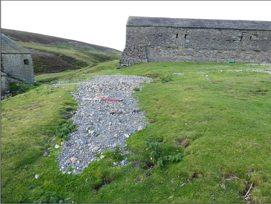
Plate 9: Gravel washed into line of head race off south-west corner of peat house, looking N (photo 2/888).
