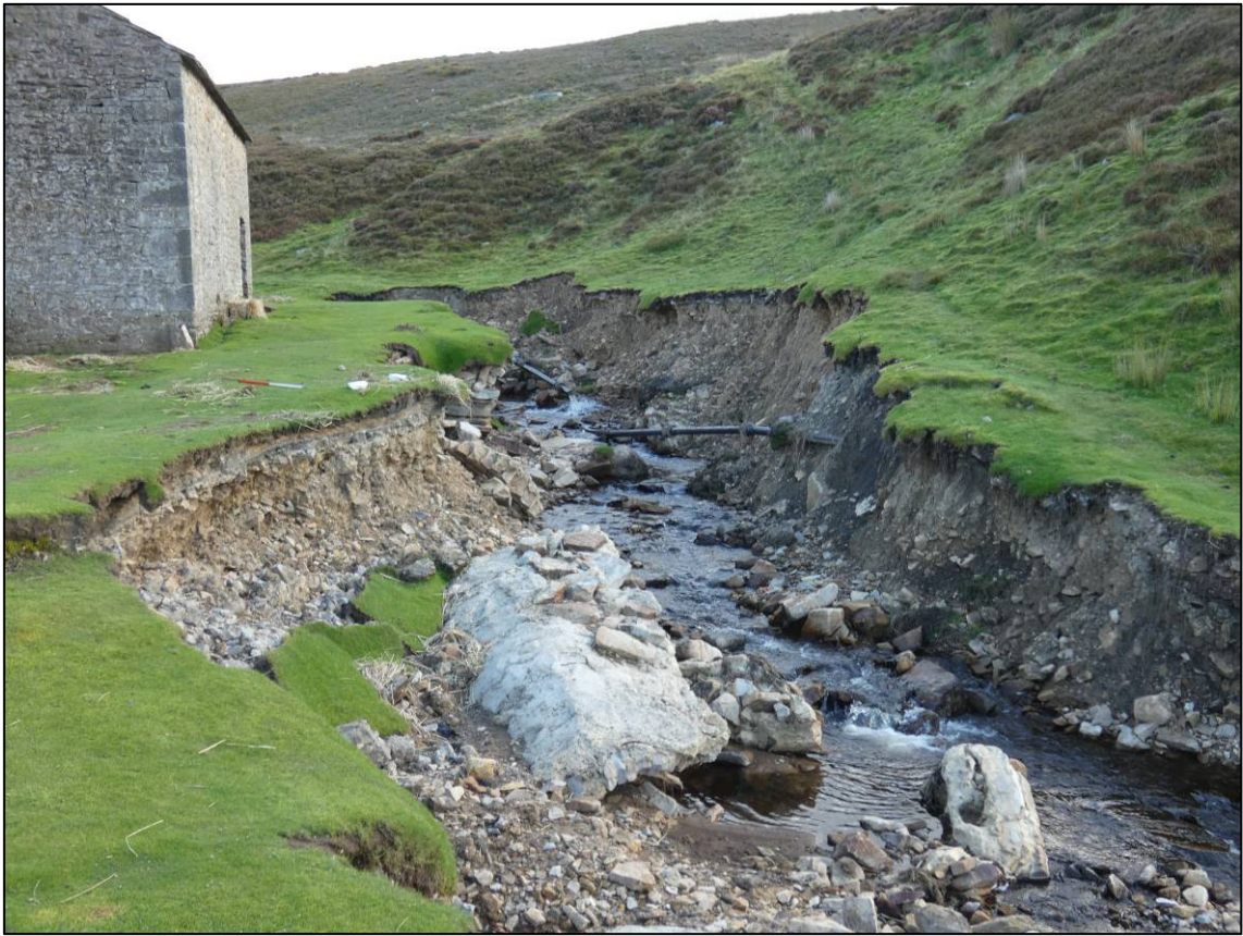
Plate 20: Damage to beck, north-west of smelt mill, looking S (photo 2/859).
