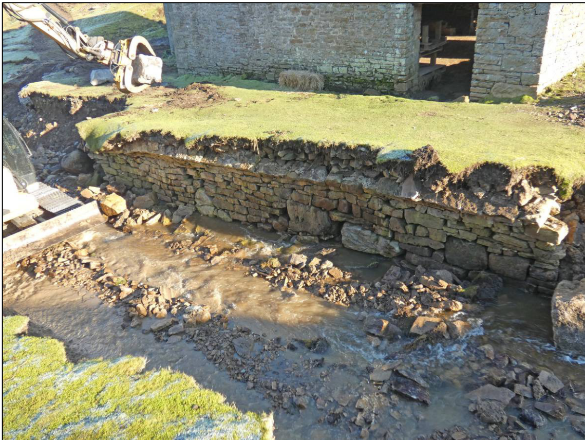
Plate 21: Remains of culvert east wall, adjacent to smelt mill, looking E (photo 3/818).
