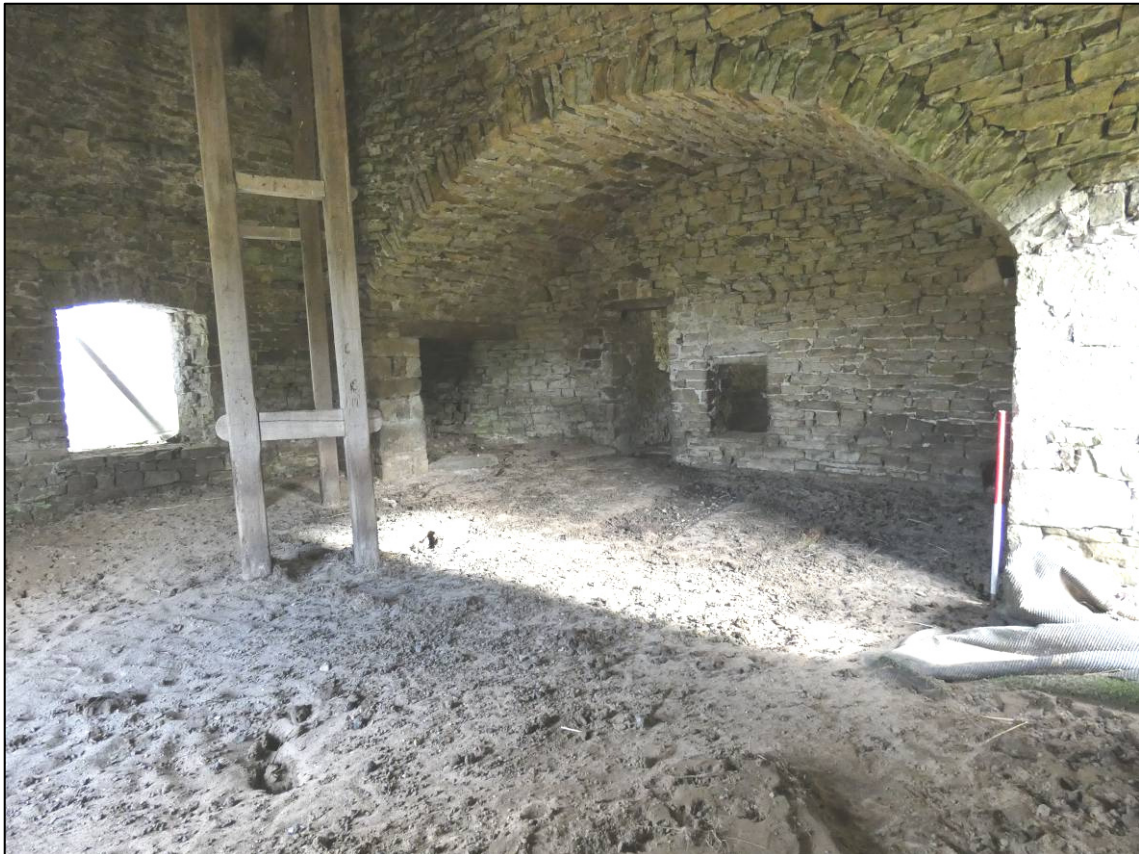
Plate 14: Flood debris in bellows room of smelt mill, looking SE (photo 2/924).
