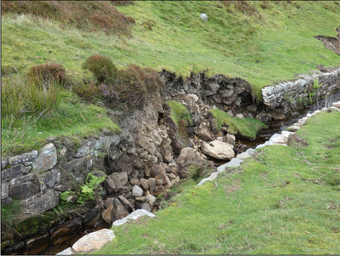
Plate 18: Localised collapse to retaining wall, west side of beck, looking NW (photo 2/905).
