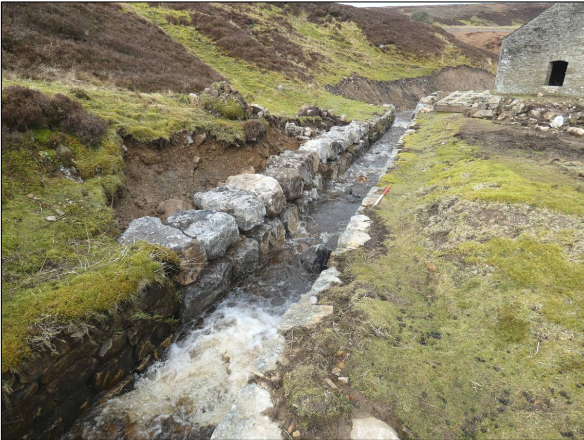
Plate 39: New retaining wall to west side of beck, prior to infilling, south of smelt mill, looking N (photo 4/141).
