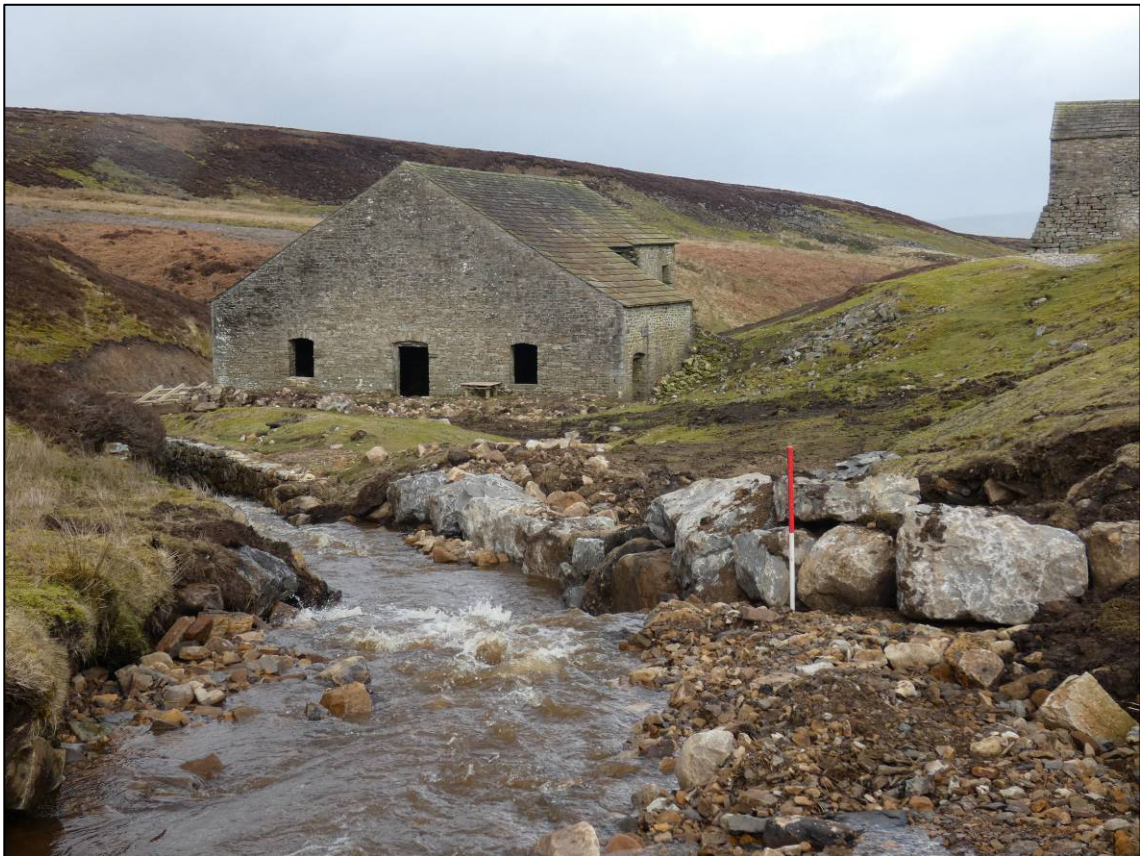
Plate 37: New beck retaining wall to east side of beck, north of reservoir dam, looking NW (plate 4/134).
