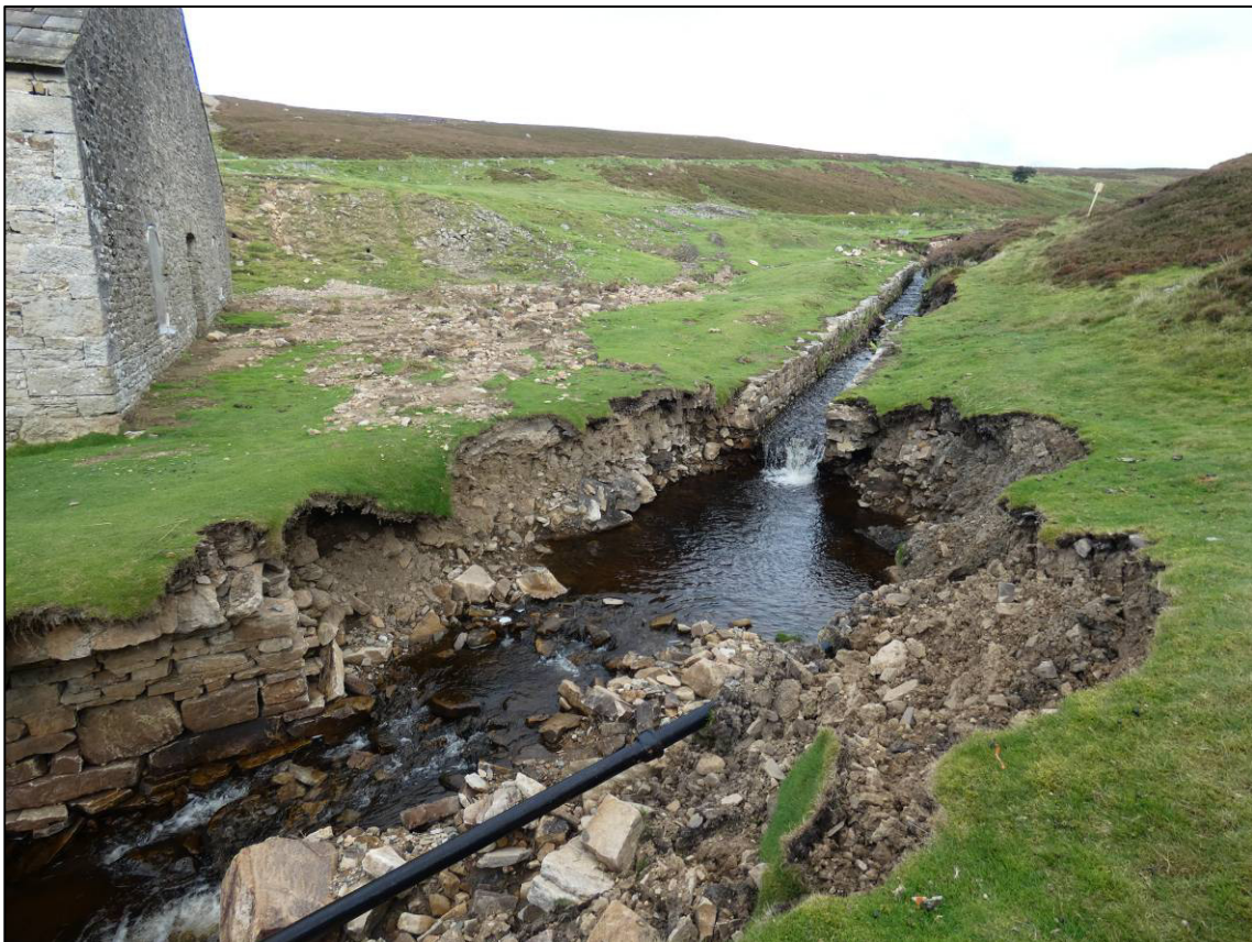
Plate 19: Flood damage off south-west corner of smelt mill, at site of south end of former culvert, looking S (photo 2/878).
