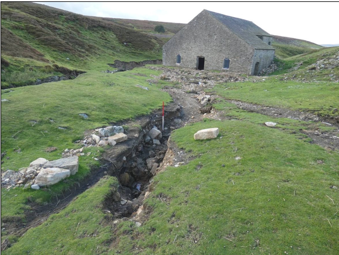
Plate 10: Erosion channel to south of smelt mill, looking NW (photo 2/894).
