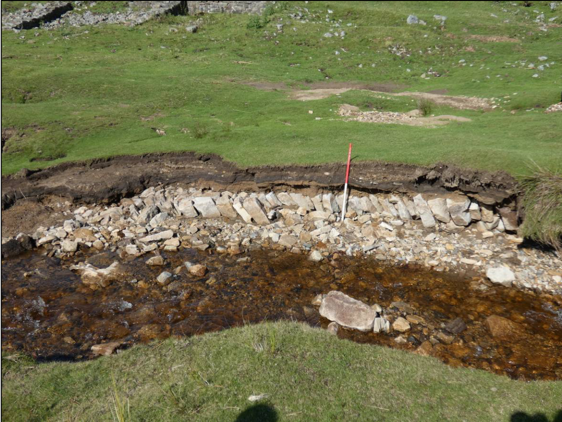
Plate 31: Reservoir dam, west facing section (S2), pitched stone surface (021) of beck/spillway, looking E (photo 1/528).
