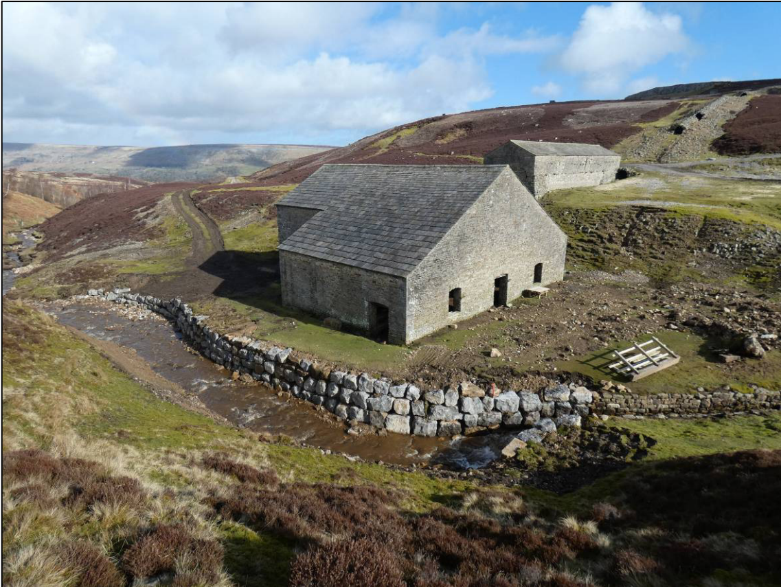
Plate 45: Completed rock-armoured wall to east side of beck, adjacent to smelt mill, looking NE (photo 4/160).
