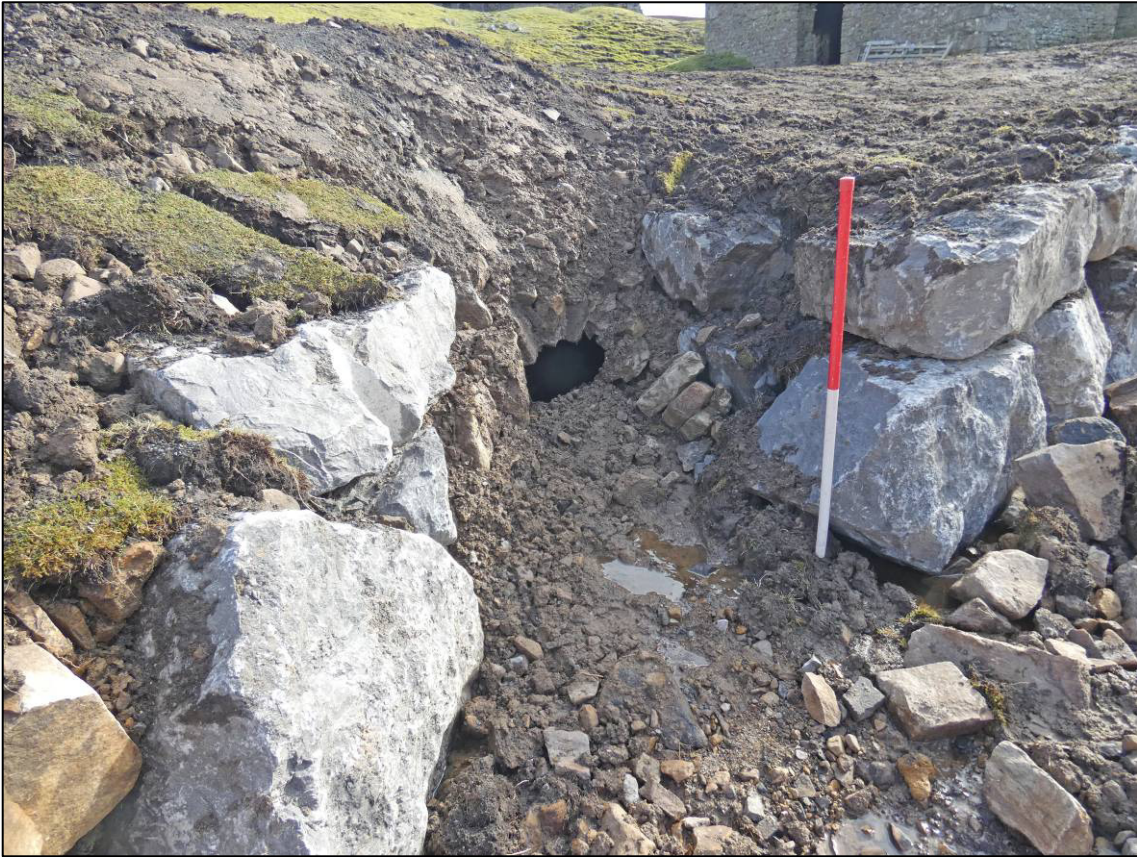
Plate 44: Gap in rock-armoured wall for smelt mill tail race, east side of back, looking SE (photo 4/150).
