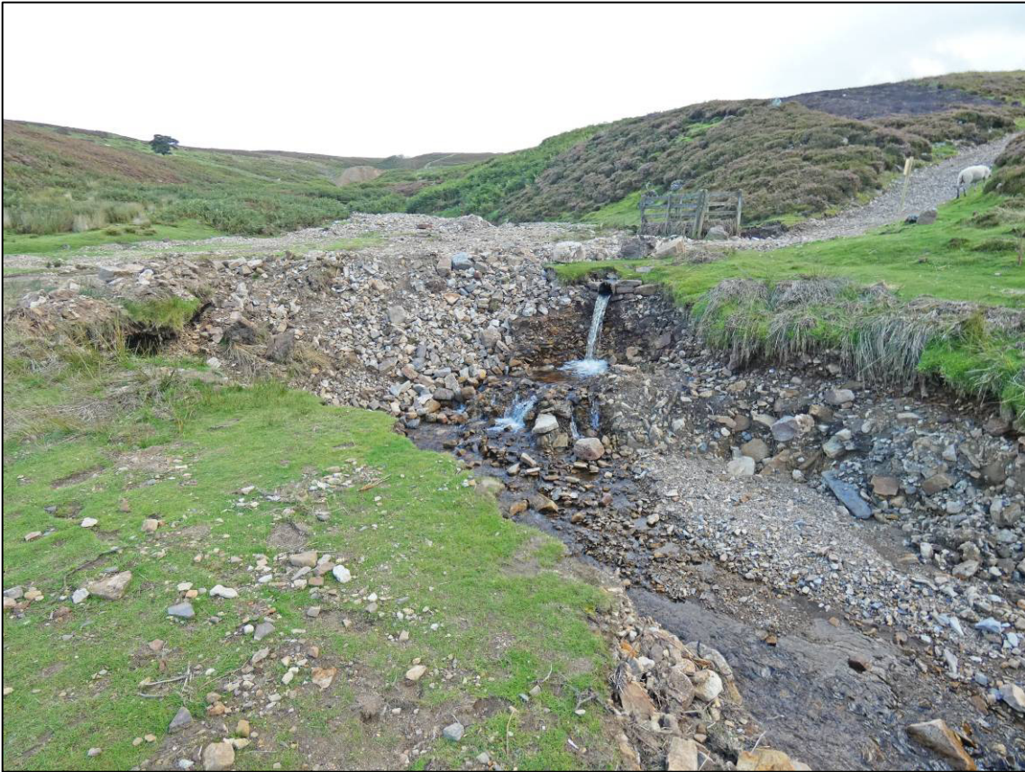
Plate 3: Flood damage adjacent to spring outfall, with reinstated track across gully, looking S (photo 2/900).
