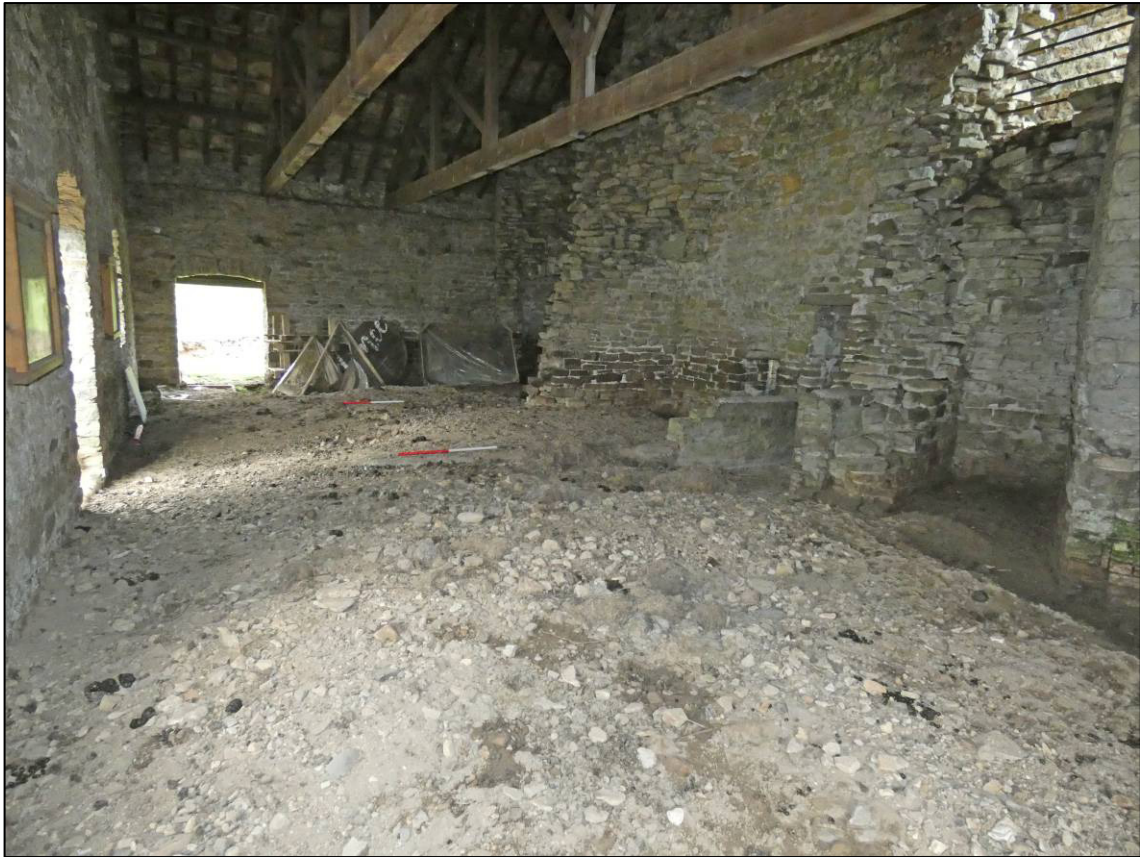
Plate 13: Flood debris in furnace room of smelt mill, looking W (photo 2/907).
