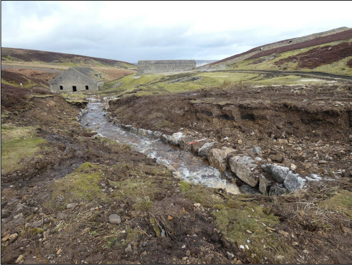
Plate 36: New retaining walls to beck and graded sides through reservoir, looking N (photo 4/130).
