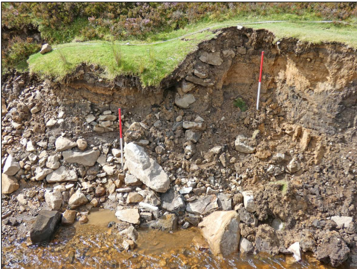
Plate 27: Reservoir dam, east facing section (S1), south part with south retaining wall (014), looking W (photo 1/517).
