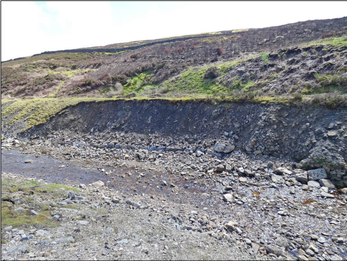
Plate 9: Area 1S, works complete and bedded-in, showing newly-exposed revetment wall at west end, looking SW (photo 3/284).
