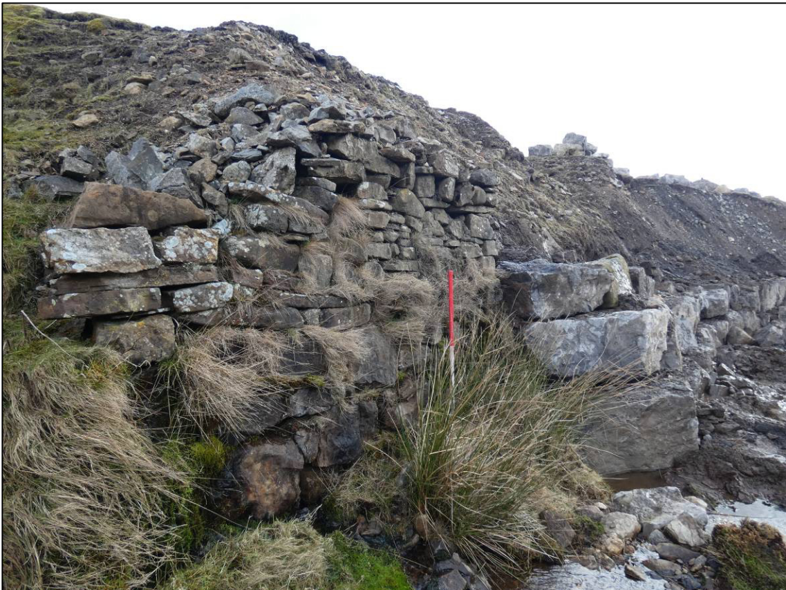
Plate 12: Area 2, existing retaining wall at west end of works, looking E (photo 1/854).
