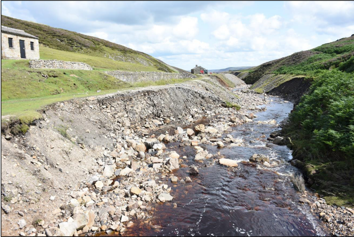
Plate 1: Area 1 erosion to north side of gill, looking SE (photo courtesy YDNPA).
