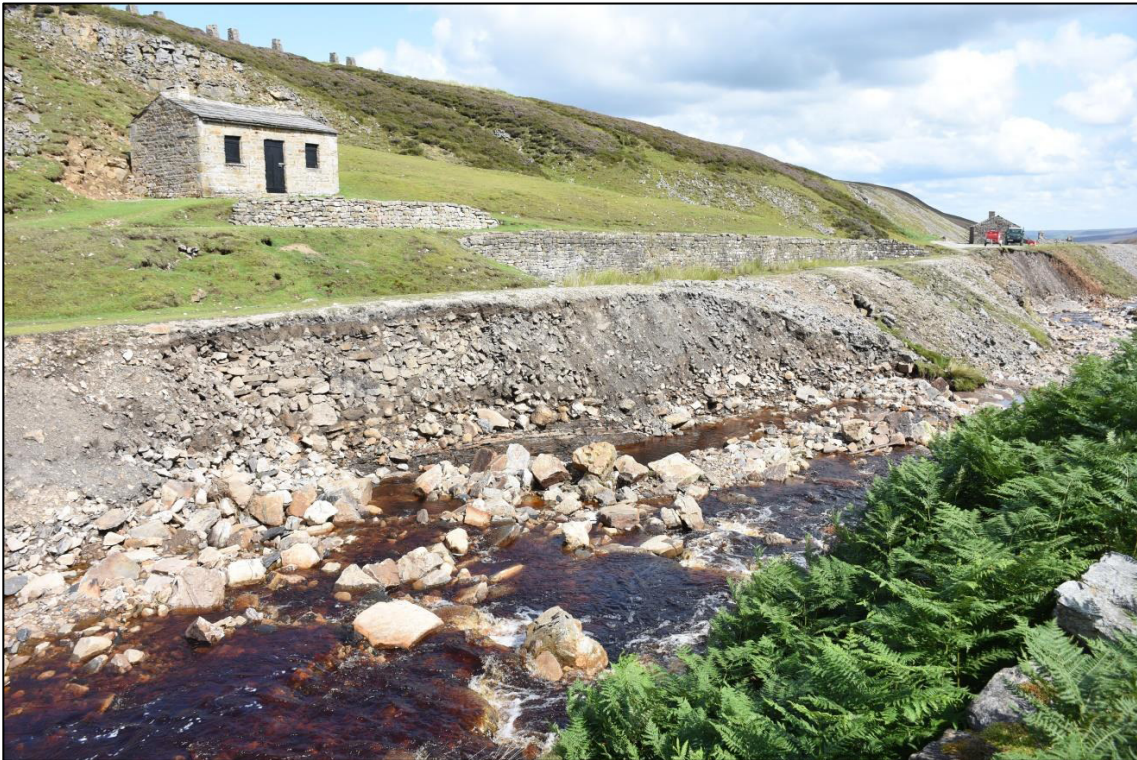
Plate 2: Area 1 erosion to north side of gill, looking E (photo courtesy YDNPA).
