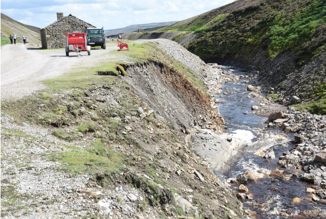
Bank erosion in front of shooting hut (approx. 40m).
