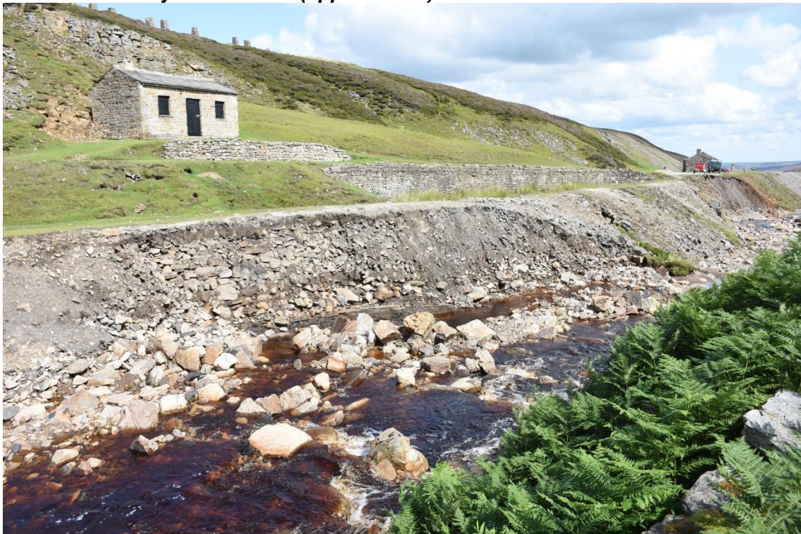
Bank erosion adjacent to dam – area 2 visible in top right
