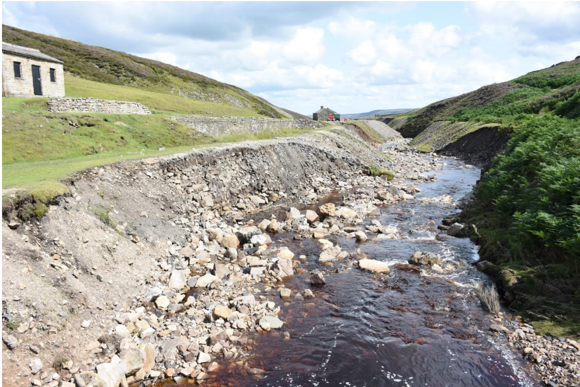
Bank erosion adjacent to dam (approx. 40m)
