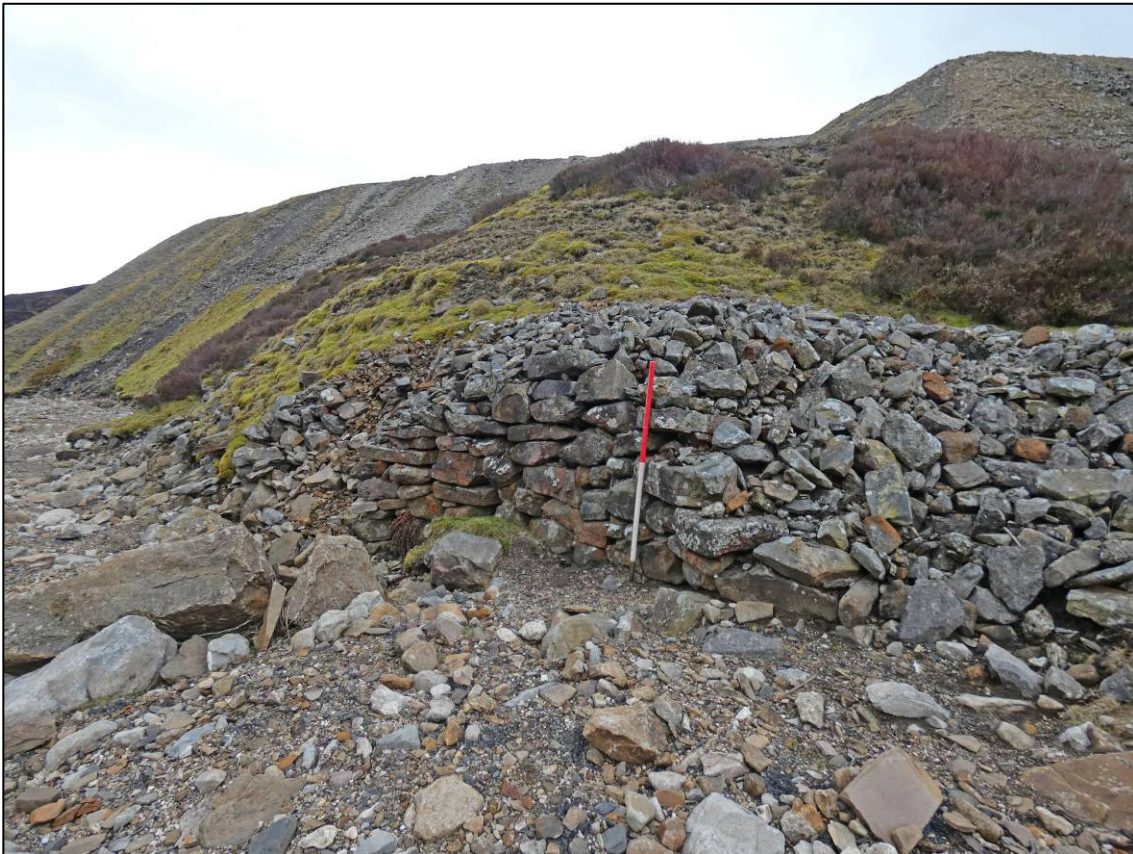
Plate 18: Area 3W, existing revetment wall to small spoil heap, looking S (photo 1/858).
