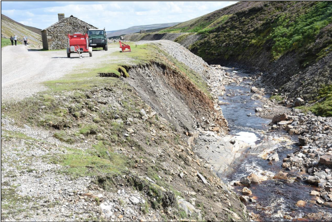
Plate 3: Area 2 erosion to north side of gill, looking SE (photo courtesy YDNPA).
