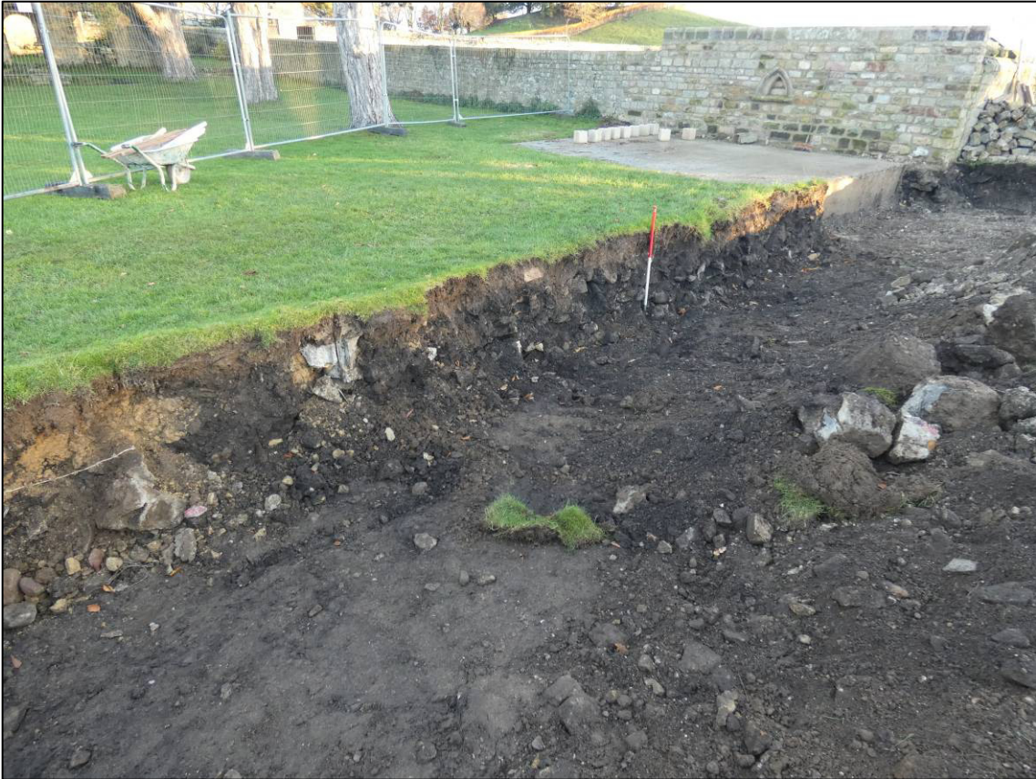
Plate 12: Ha-ha excavation, Section 3, remains of original ha-ha retaining wall (012) being removed, looking NE (photo 3/600).
