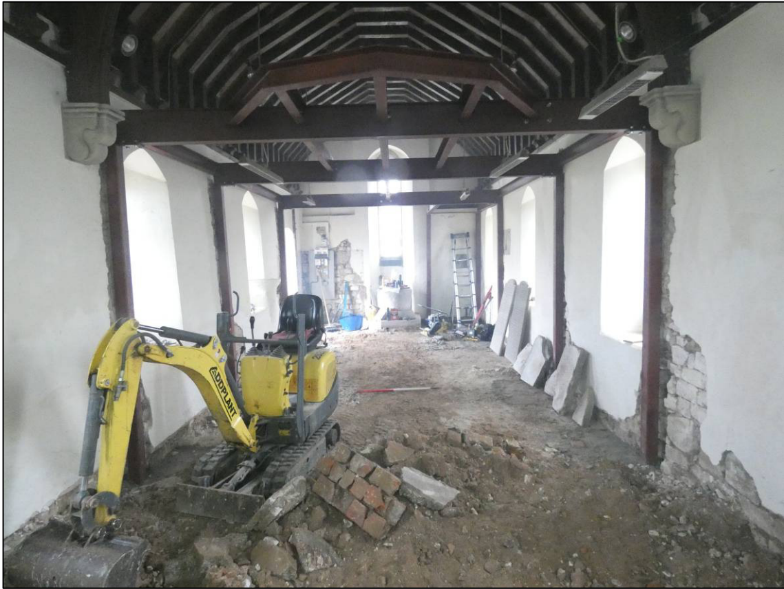
Plate 52: General view of interval excavations, with steelwork for mezzanine floor in position, looking W.
