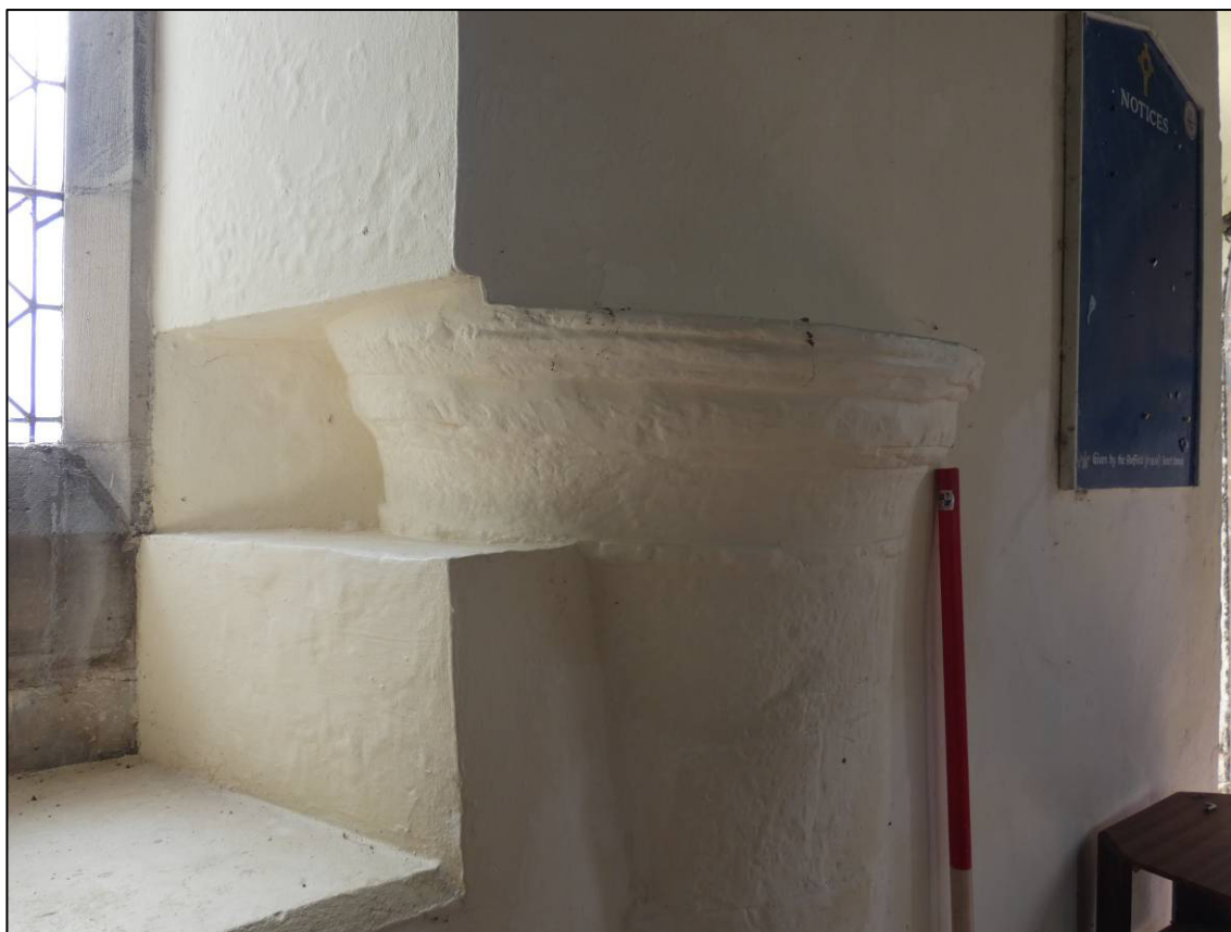
Plate 22: Internal face of south wall, showing pier and window embrasure, looking SW (photo 1/043).
