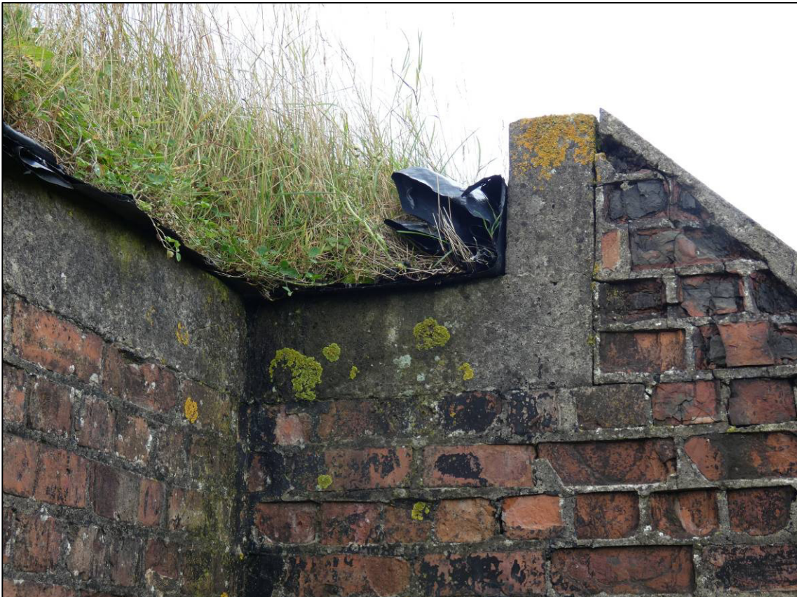
Plate 2: Shelter, detail of raised lip to roof over entrance, looking S (photo 1/081).
