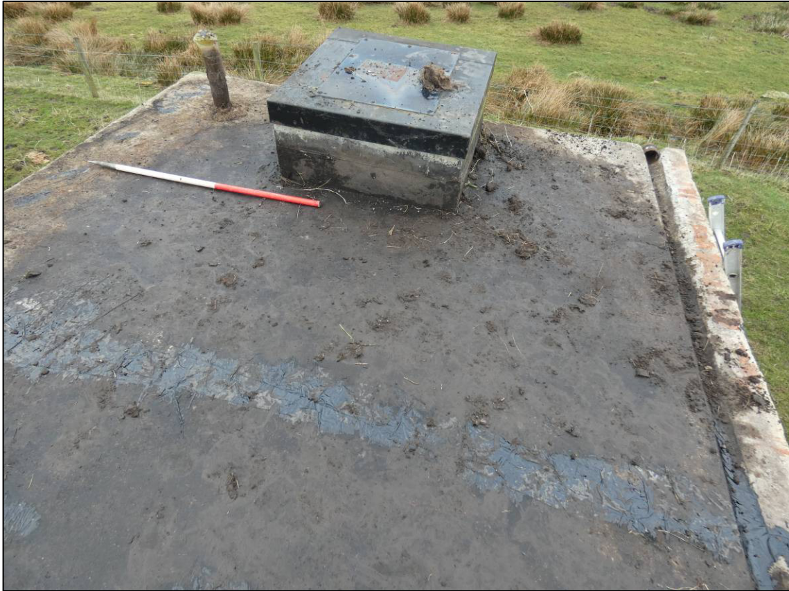
Plate 9: Shelter, roof after removal of turf, showing earlier repairs, drain, hatch and chimney to vent, looking NE (photo 2/413).
