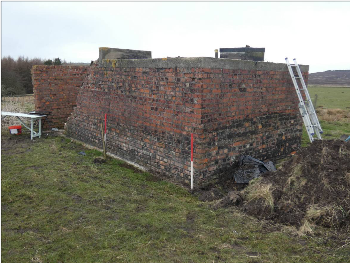
Plate 11: General view of shelter after removal of turf to roof, looking N (photo 2/420).
