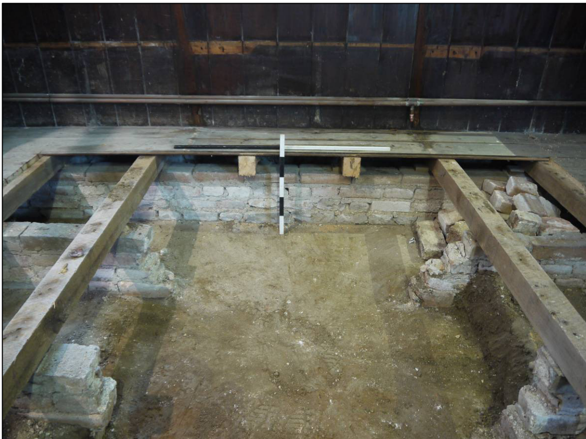
Plate 4: Open trench after completion of excavation, showing structure of pew platform, looking N.
