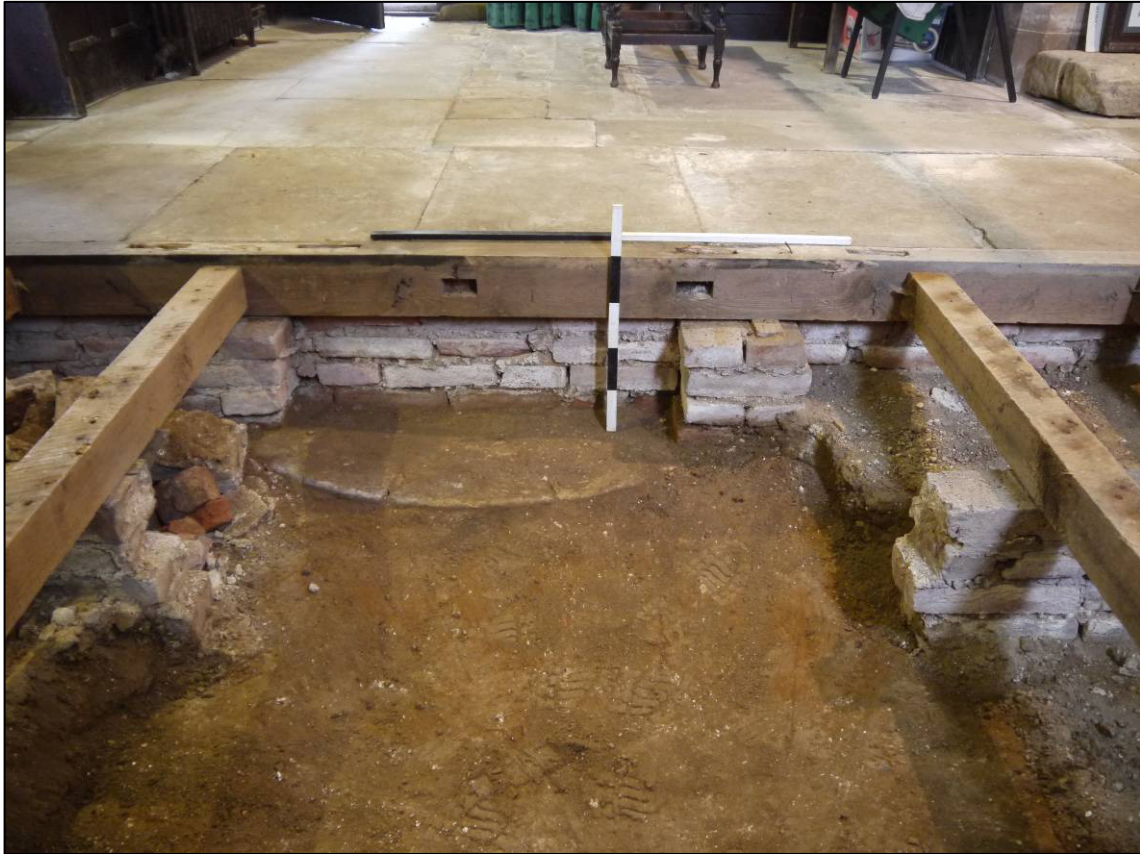
Plate 5: Open trench after completion of excavation, showing structure of pew platform and exposed plinth (109), looking S.
