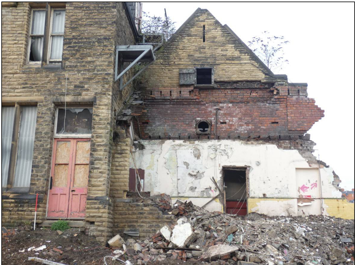
Plate 17: East elevation after demolition, former north wall of corridor (G11) with Operating Theatre (G10) behind, looking N (photo 2/209).
