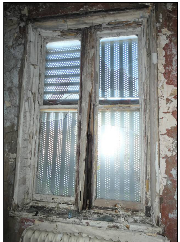
Plate 6: First floor room (1F2), Type 1 window in north wall, looking N (photo 1/741).
