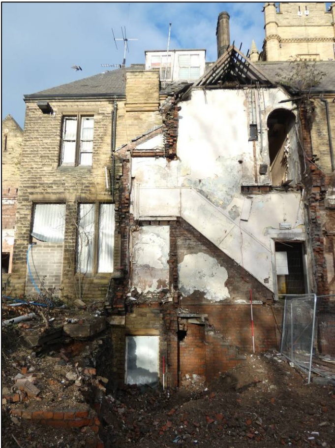
Plate 21: South elevation after demolition, former two storey part of service wing, looking N (photo 2/185).
