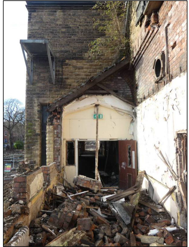
Plate 16: East elevation after demolition, former west wall of corridor (G11), looking W (photo 2/168).
