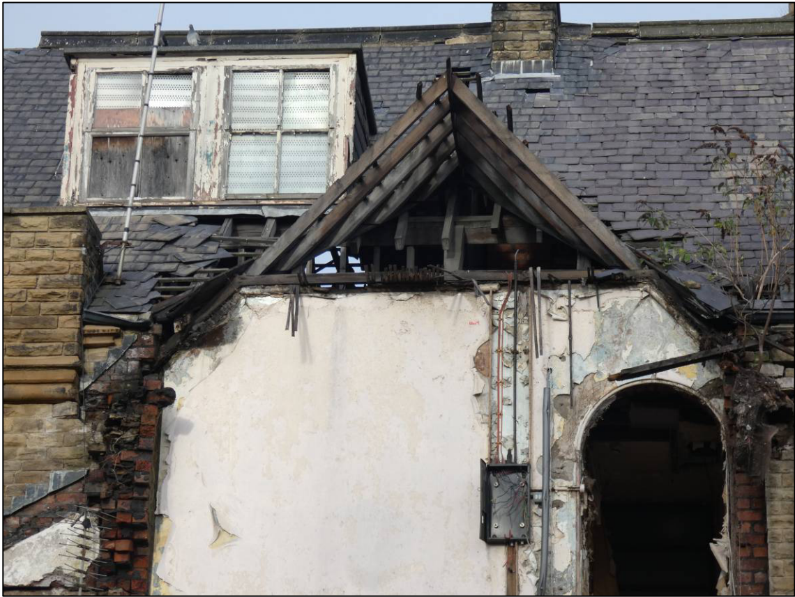
Plate 23: South elevation after demolition, former two storey part of service wing, attic, looking N (photo 2/198).
