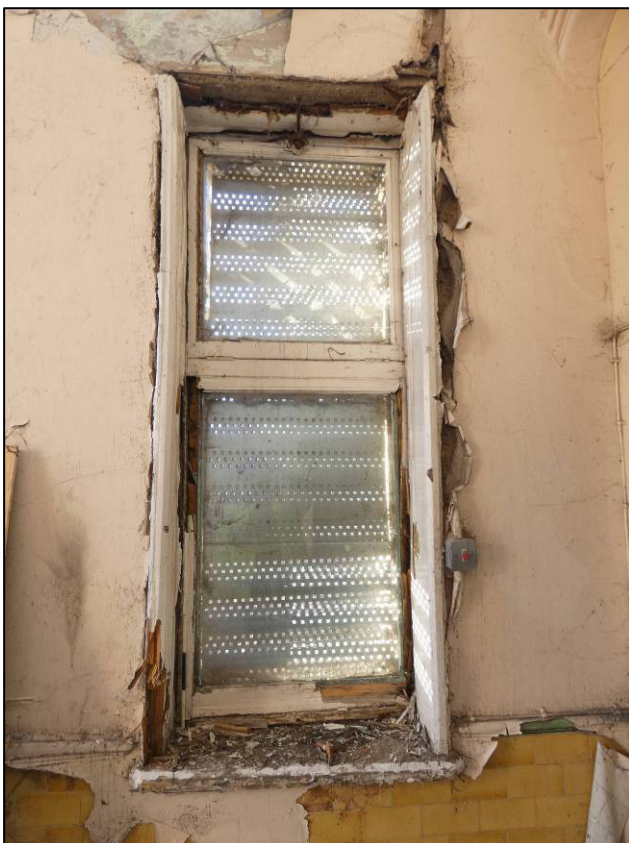
Plate 5: Ground floor room (G11), Type 2 window (G11/1) in south wall, looking S (photo 1/725).
