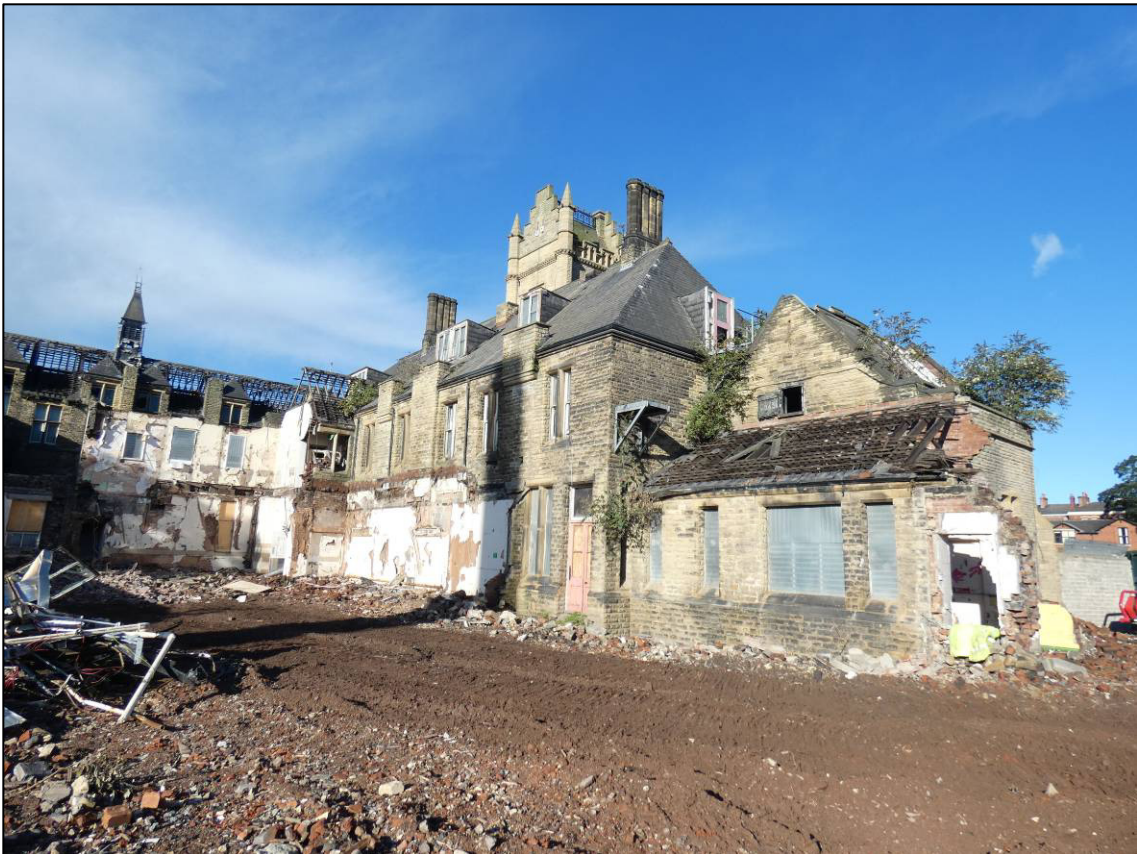
Plate 2: Rear (south) elevation of retained building, with demolition of adjacent structures on going, looking NW (photo 1/758).
