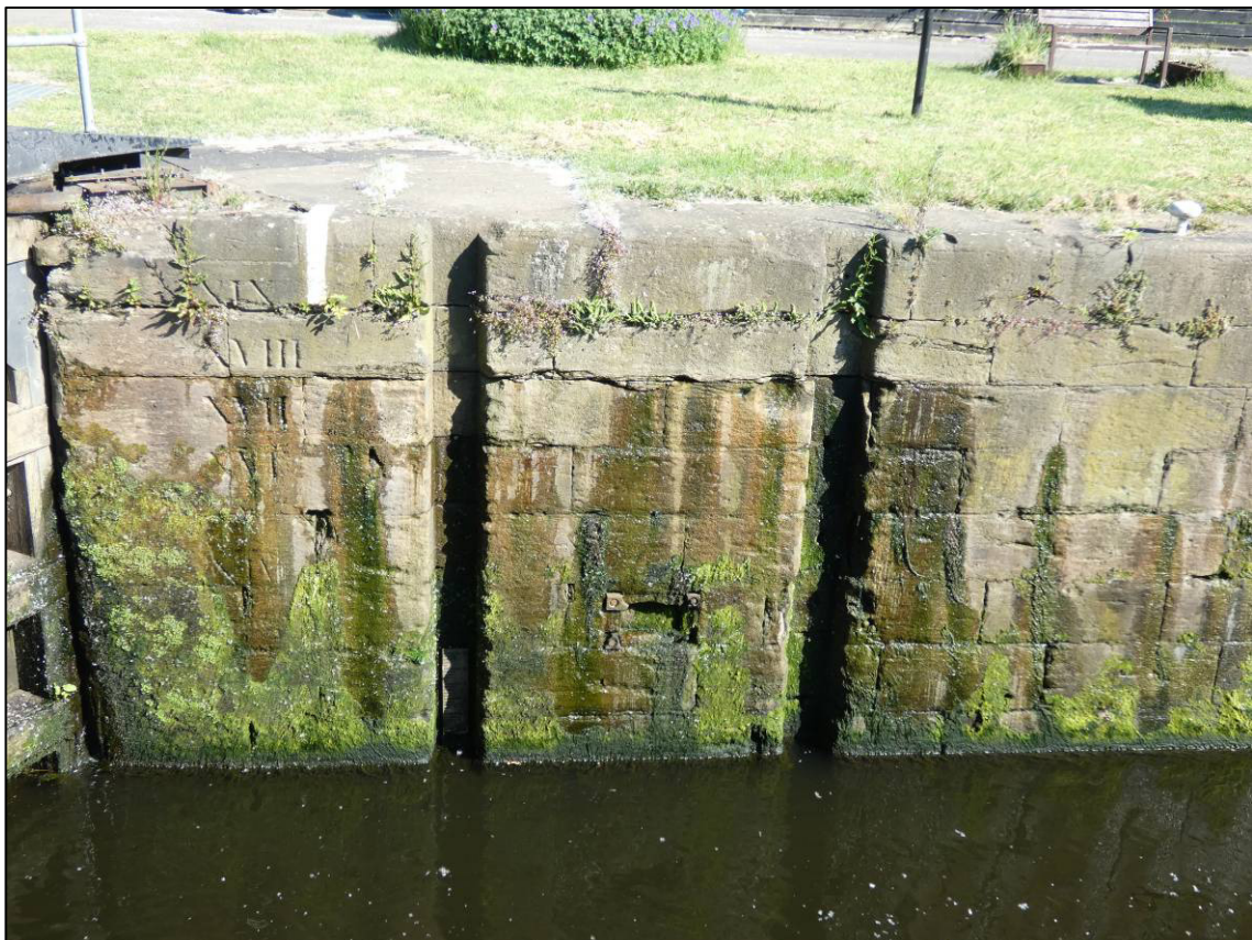
Plate 14: East approach, north wall showing stop plank grooves etc, looking N (photo 2/774).
