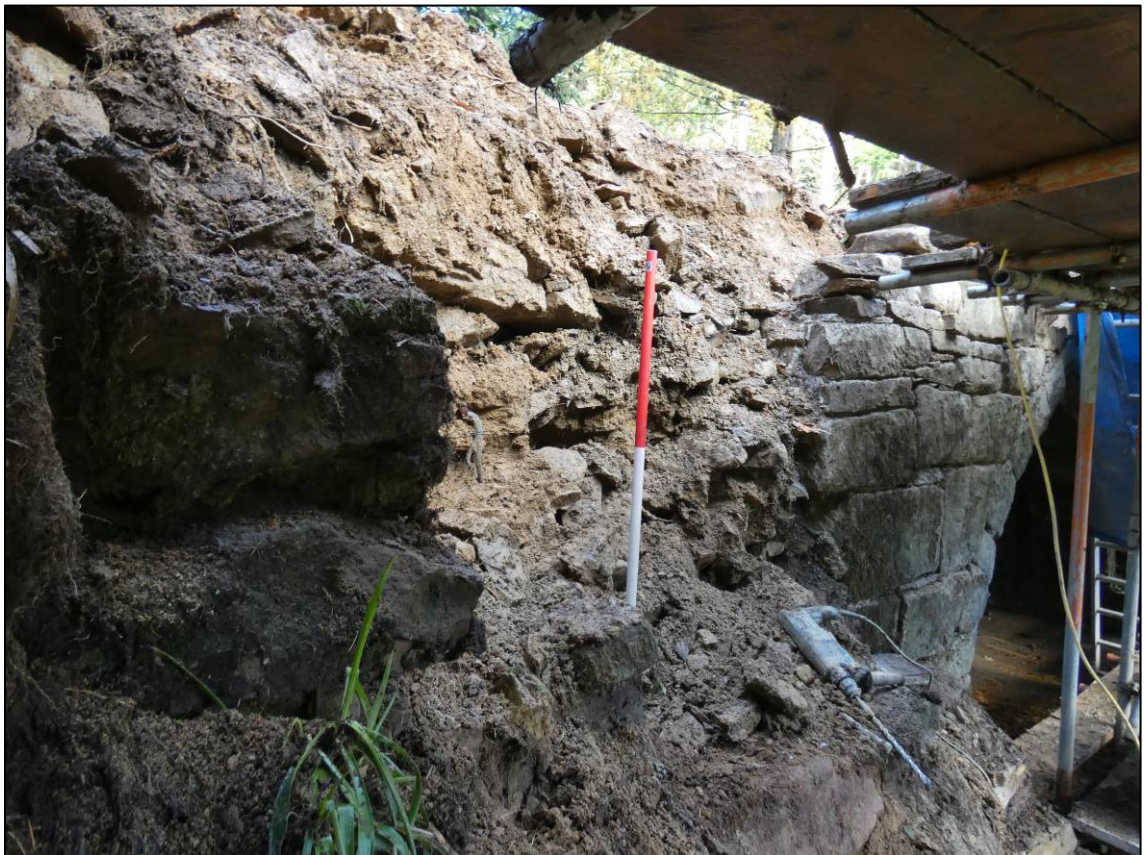
Plate 26: South elevation, area west of arch under repair, showing possible internal faces to core, looking E (photo 4/441).
