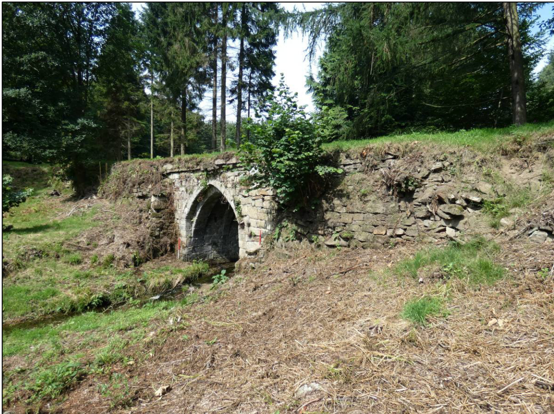
Plate 7: View of south elevation and east abutment, prior to repairs, looking NW (photo 1/885).
