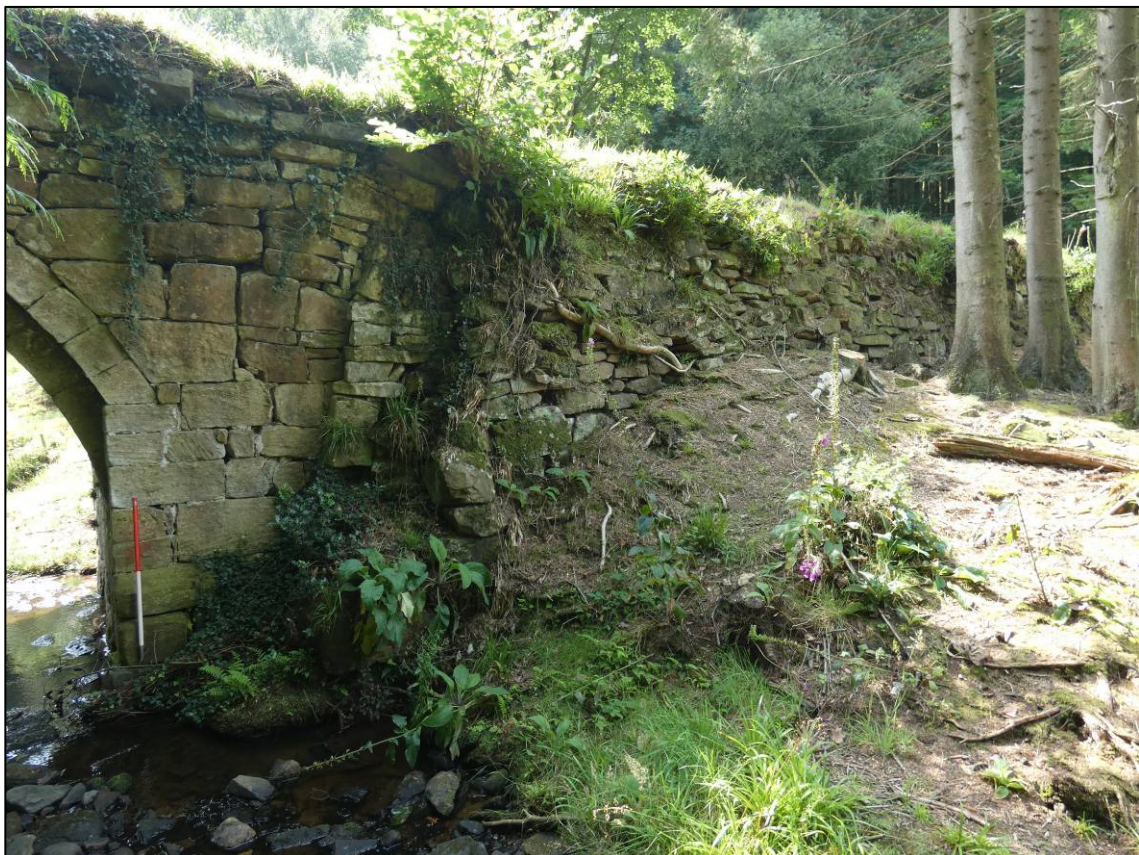
Plate 11: North elevation, west buttress/return and abutment, prior to repairs, looking SW (photo 1/906)
