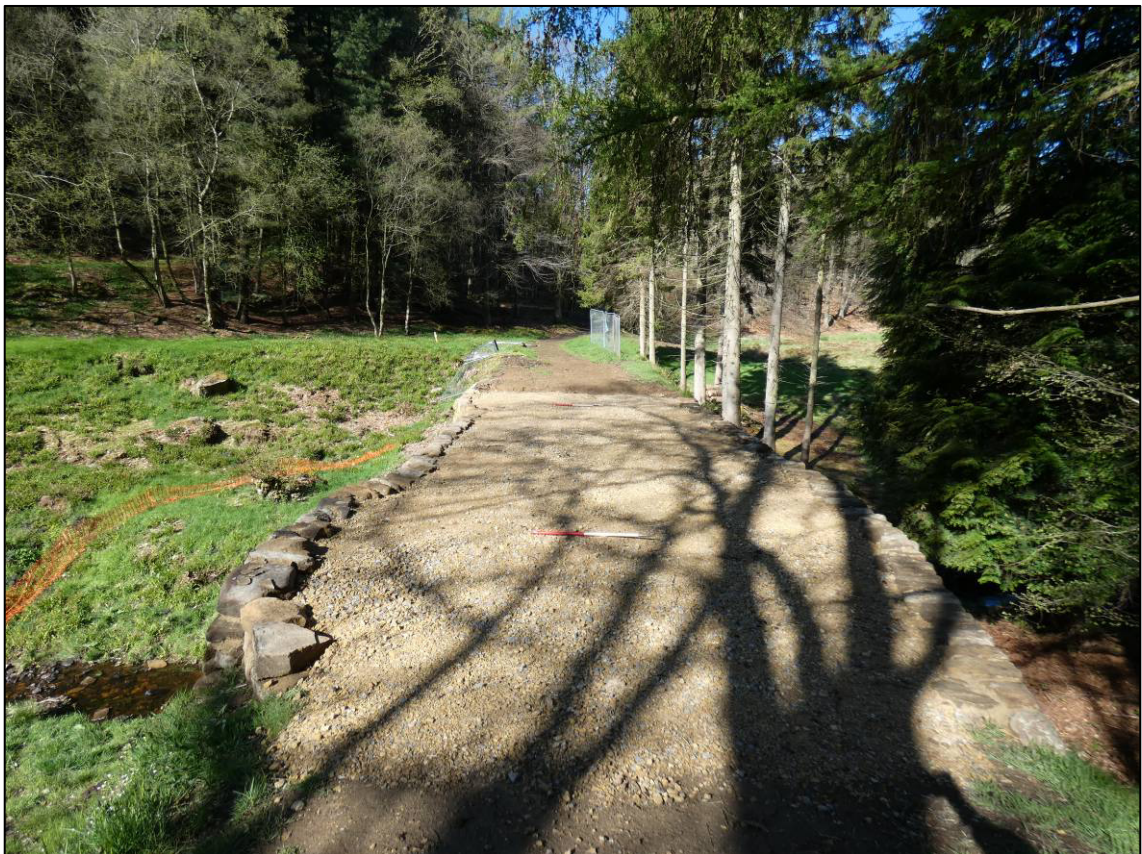
Plate 36: Top of bridge, repairs complete, grass to be sown, looking E (photo 8/562).
