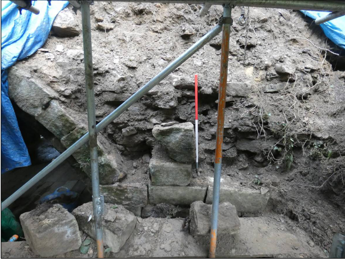
Plate 25: South elevation, area east of arch under repair, showing central core, looking N (photo 3/293).
