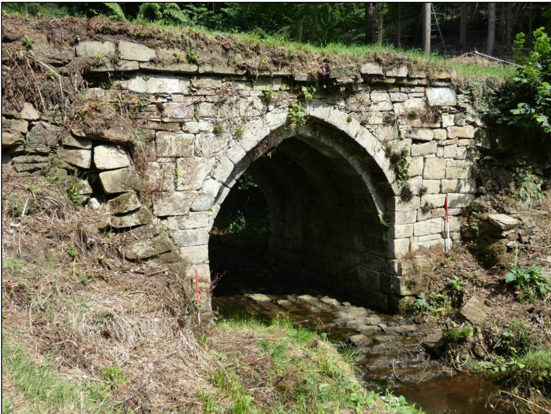
Plate 13: South elevation and west buttress/return, prior to repairs, looking NE (photo 1/893).
