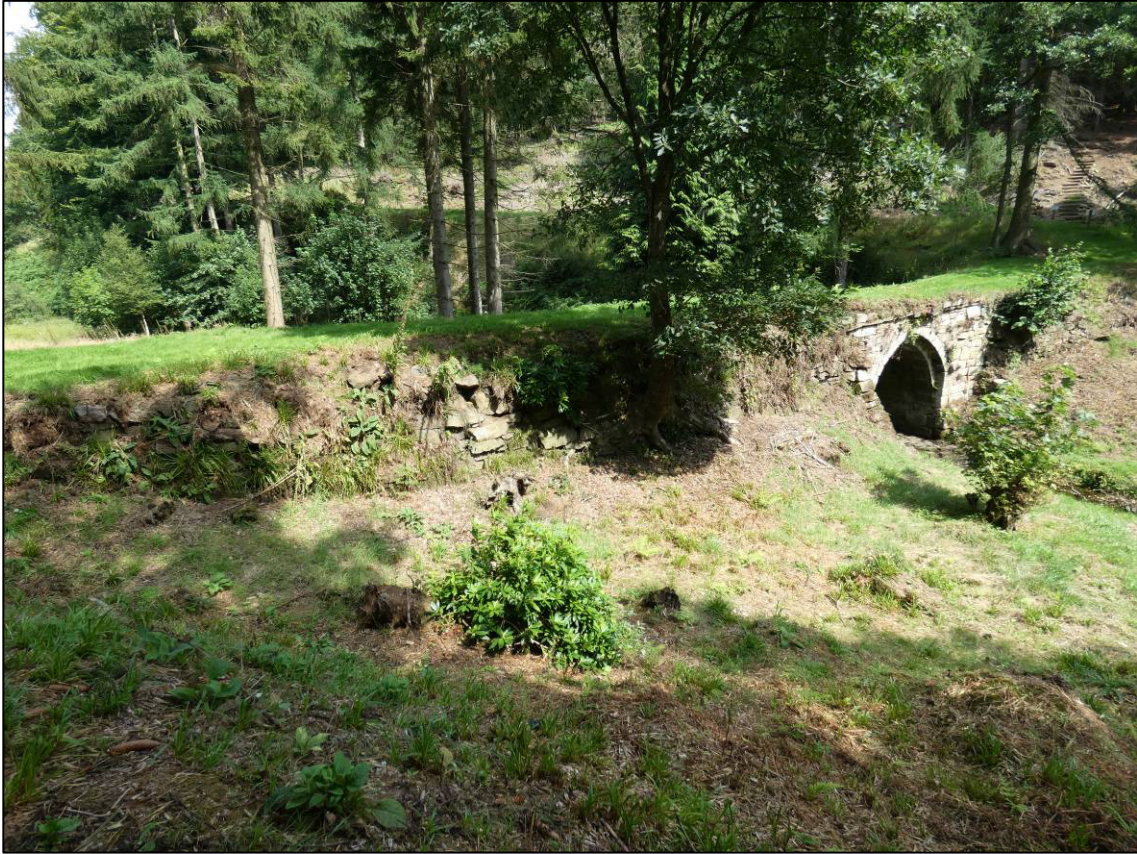
Plate 6: View of south elevation and west abutment, prior to repairs, looking NE (photo 1/896).
