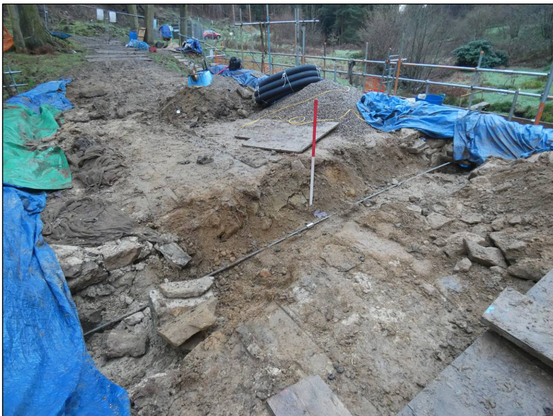
Plate 32: Excavated west trench (Trench B) across bridge top, with tie bar inserted, looking W (photo 6/777).
