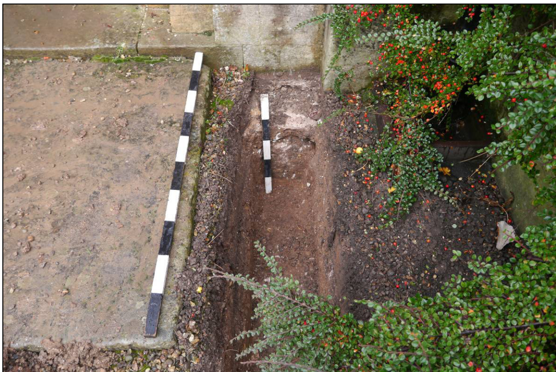
Plate 6: Foundations to south aisle wall (110, 111 and 112) at north end of Trench 1, looking N.
