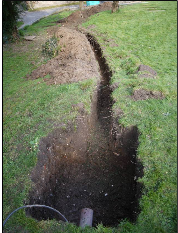
Plate 8: North part of Trench 2, showing curving alignment from central inspection chamber, looking N.
