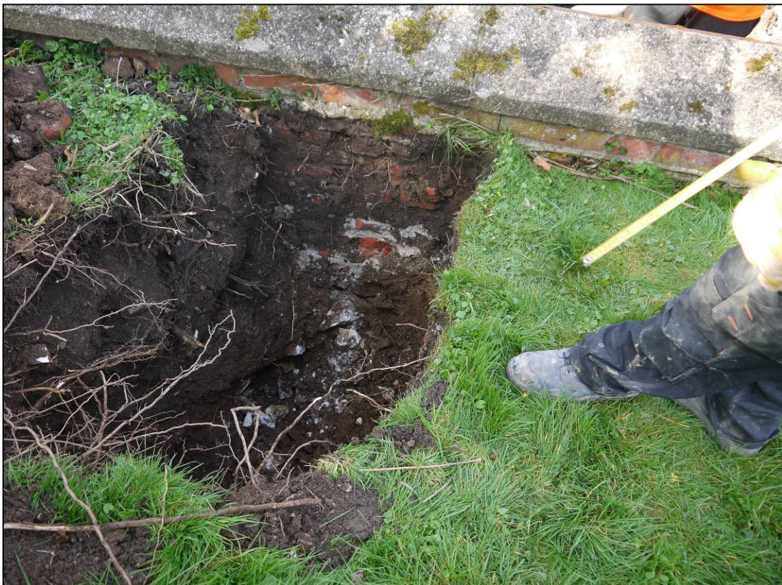
Plate 9: Northern end of Trench 2, inspection chamber against north churchyard boundary wall (115), looking NW.
