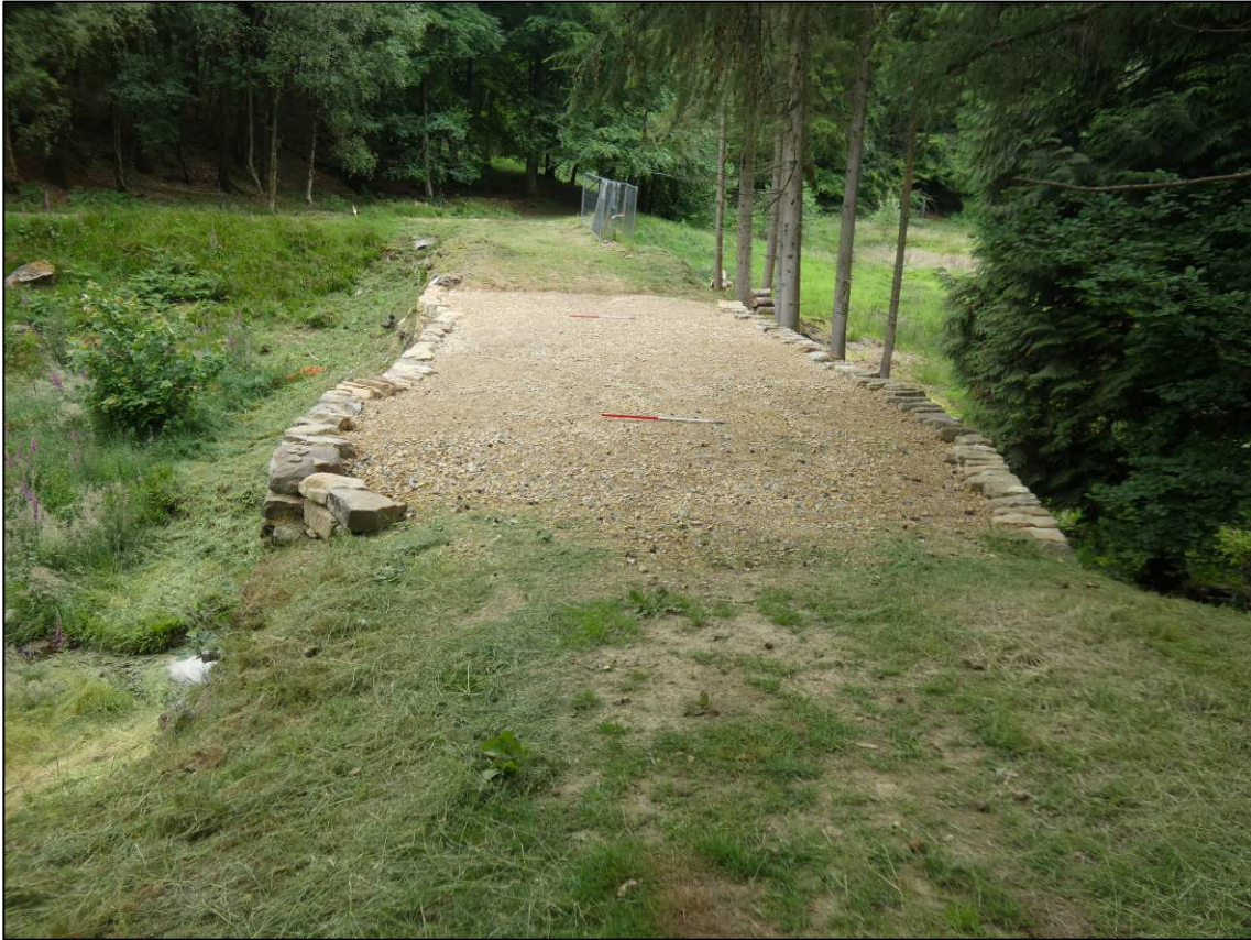
Plate 1: Bridge and abutment surfaces before start of Phase 2 works, looking SW (photo 1/823).
