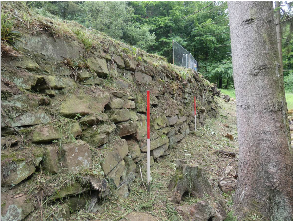
Plate 4: West abutment, north elevation, before start of Phase 2 works, looking SW (photo 1/834).
