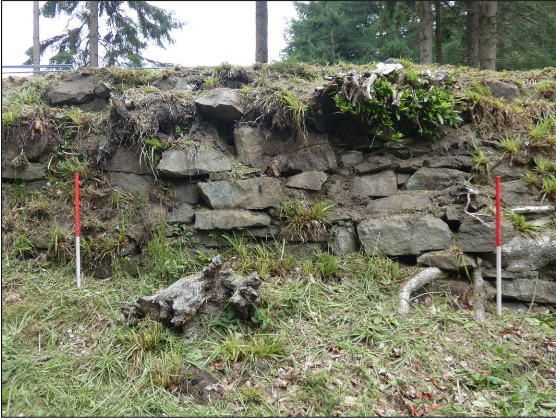
Plate 3: West abutment, south elevation, central section, before start of Phase 2 works, looking NW (photo 1/830).
