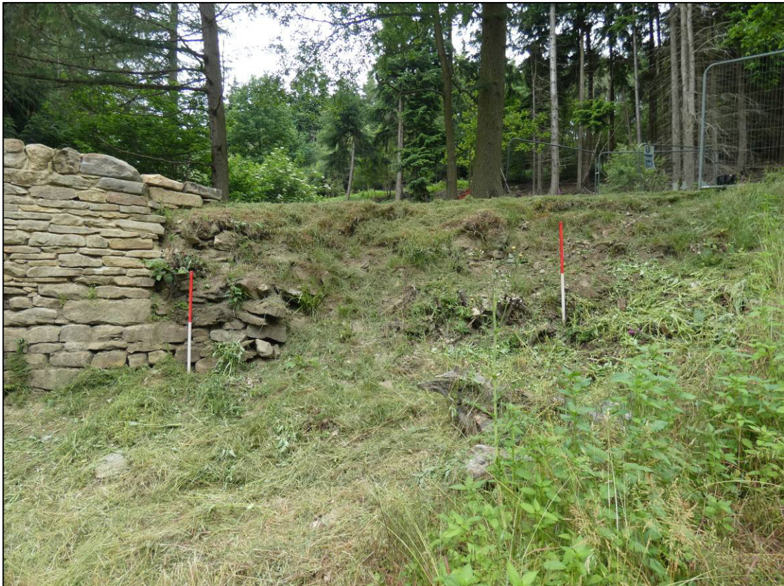
Plate 6: East abutment, south elevation, before start of Phase 2 works, looking N (photo 1/850).
