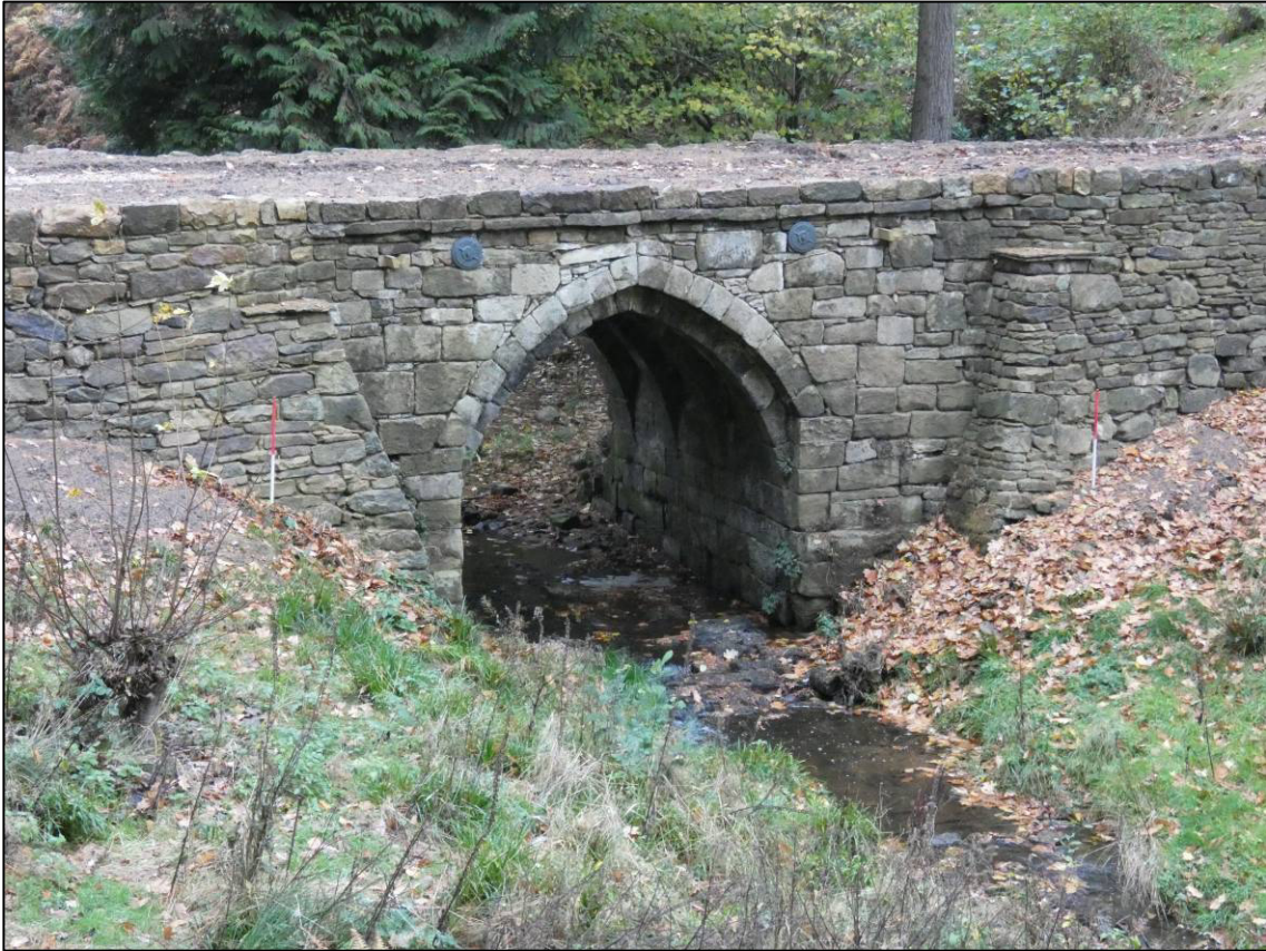
Plate 15: South elevation of main bridge structure, after initial Phase 1 repairs, looking N (photo 6/009).
