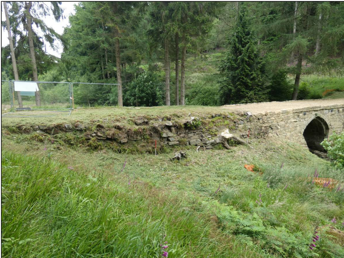
Plate 2: West abutment, south elevation, before start of Phase 2 works, looking N (photo 1/826).
