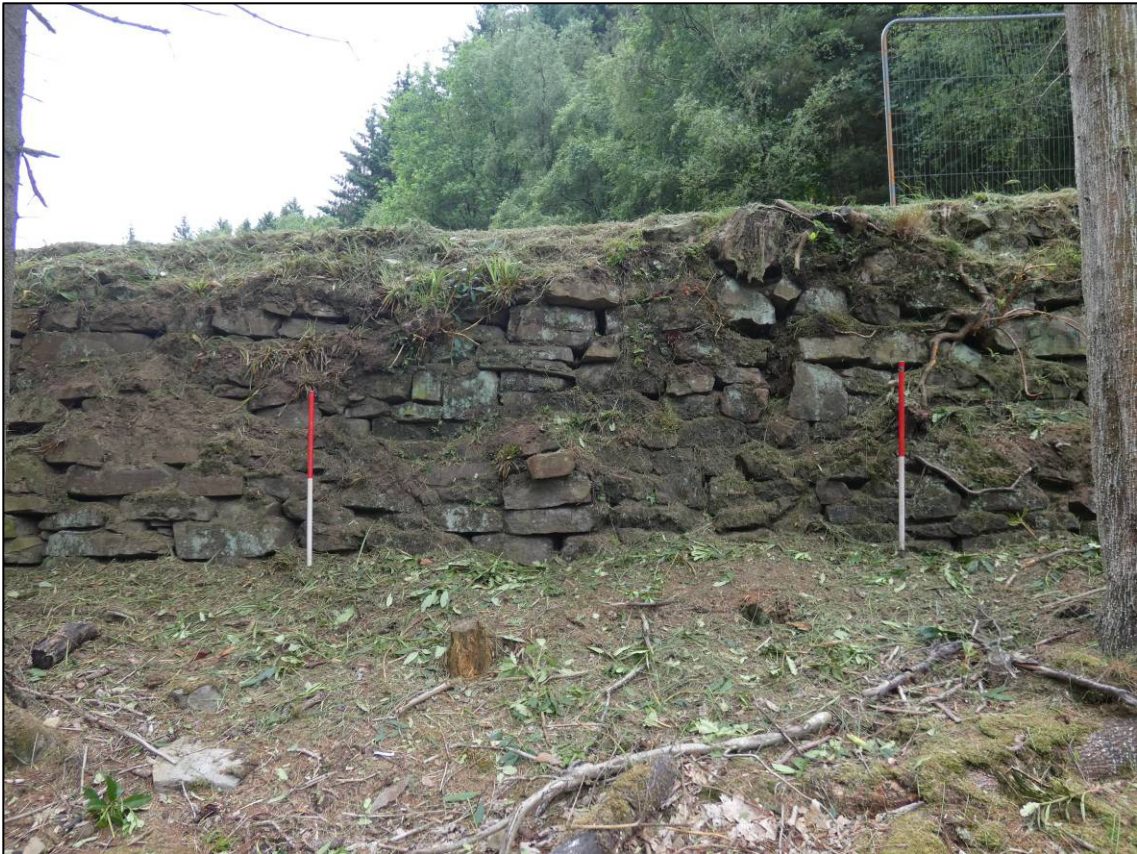
Plate 5: West abutment, north elevation, central section, before start of Phase 2 works, looking SE (photo 1/838).
