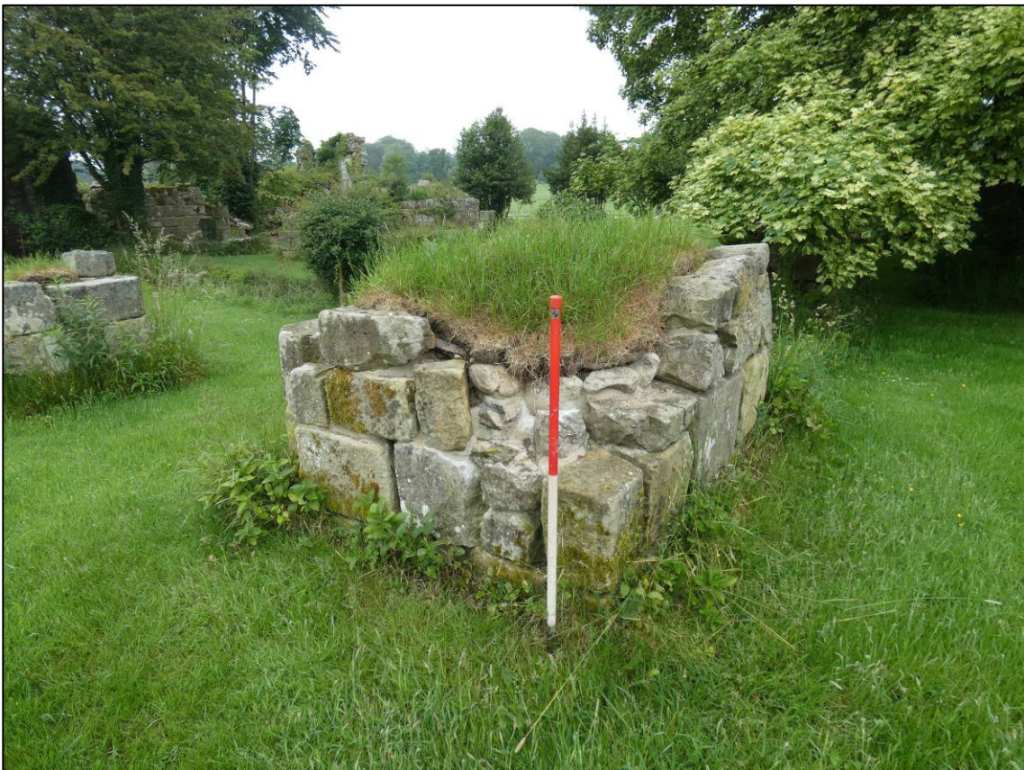
Plate 9: Area 2: Lay brothers' rear-dorter, east return to west wall, after repair, looking SE (photo 6/666).
