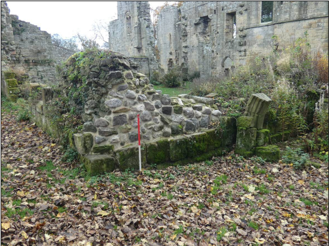
Plate 48: Area 15: Infirmary's lodging, west external elevation of west wall (north end), after repair, looking SE (photo 7/616).
