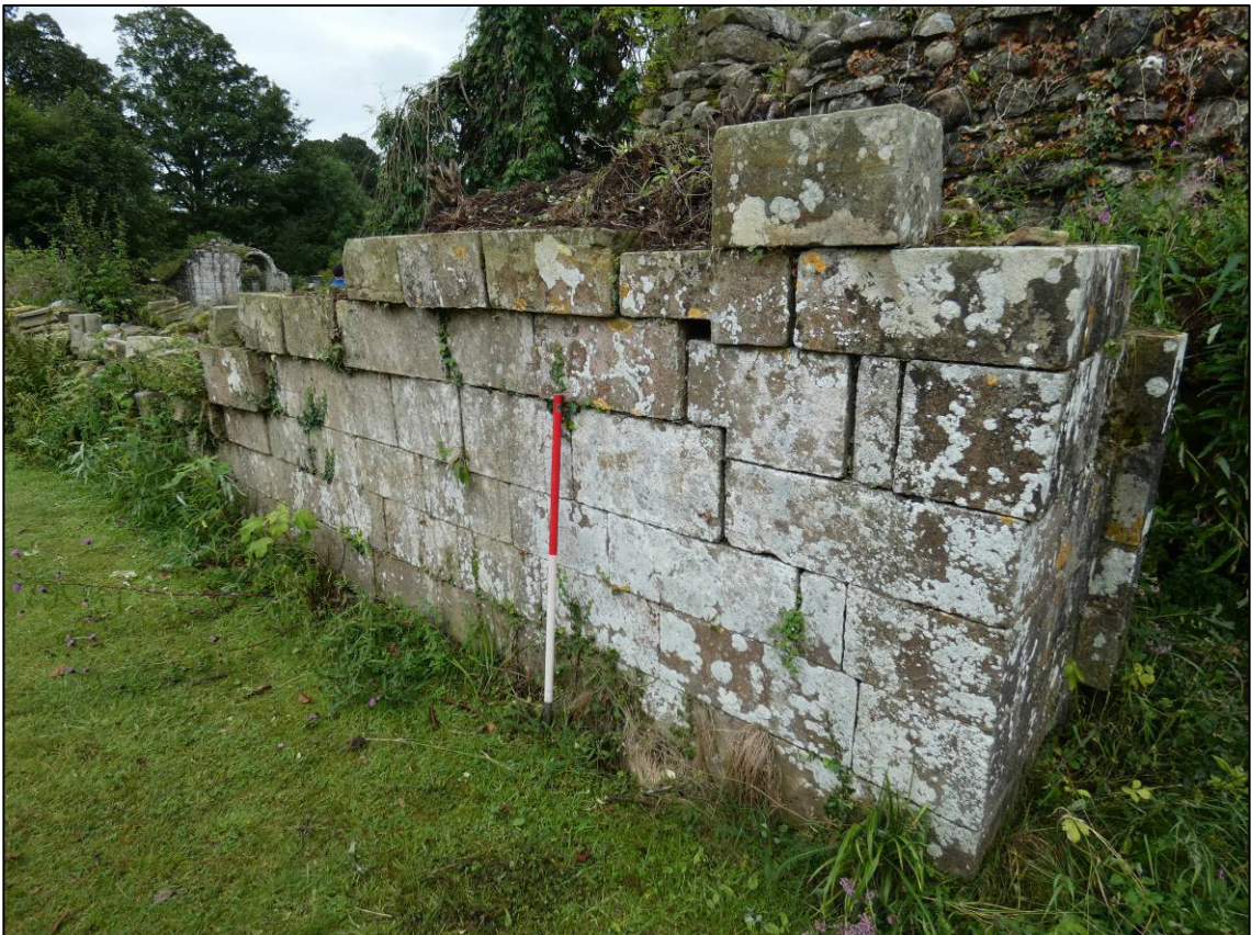
Plate 56: Area 18: Abbey church, lay brothers' quire, north internal elevation of south wall (west part), during clearance showing doorway opening, looking SE (photo 2/475).
