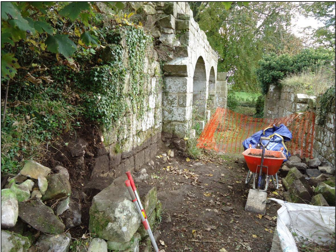
Plate 50: Area 16: Vestry, south internal elevation of north wall, during repair, looking NE (photograph courtesy Peter Pace).
