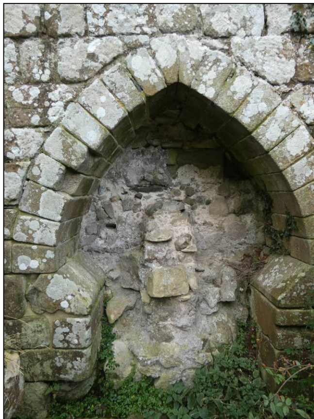
Plate 45: Area 14: Monks' rere-dorter, south internal elevation of drain, western arch after repair, looking S (photo 7/619).
