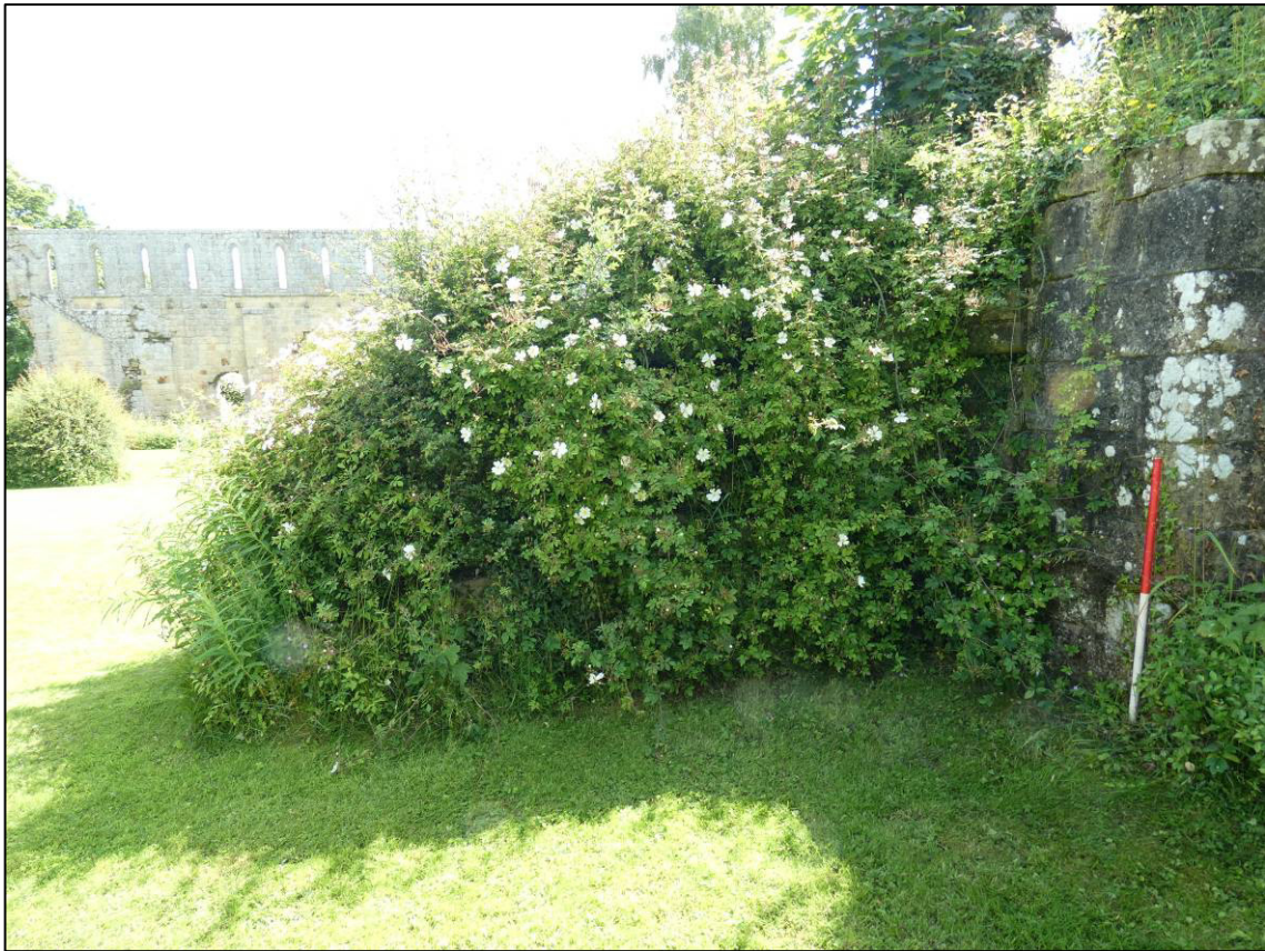
Plate 12: Area 4: Lay brothers' quarters (frater), west internal elevation of east wall (south end), before clearance, looking E (photo 1/278).
