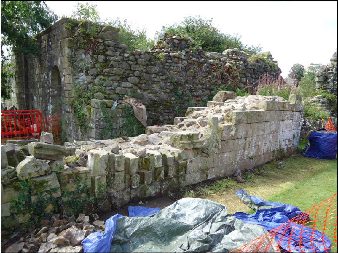
Plate 57: Area 18: Abbey church, lay brothers' quire, north internal elevation of south wall (west part), during repair, looking SW (photograph courtesy Peter Pace).
