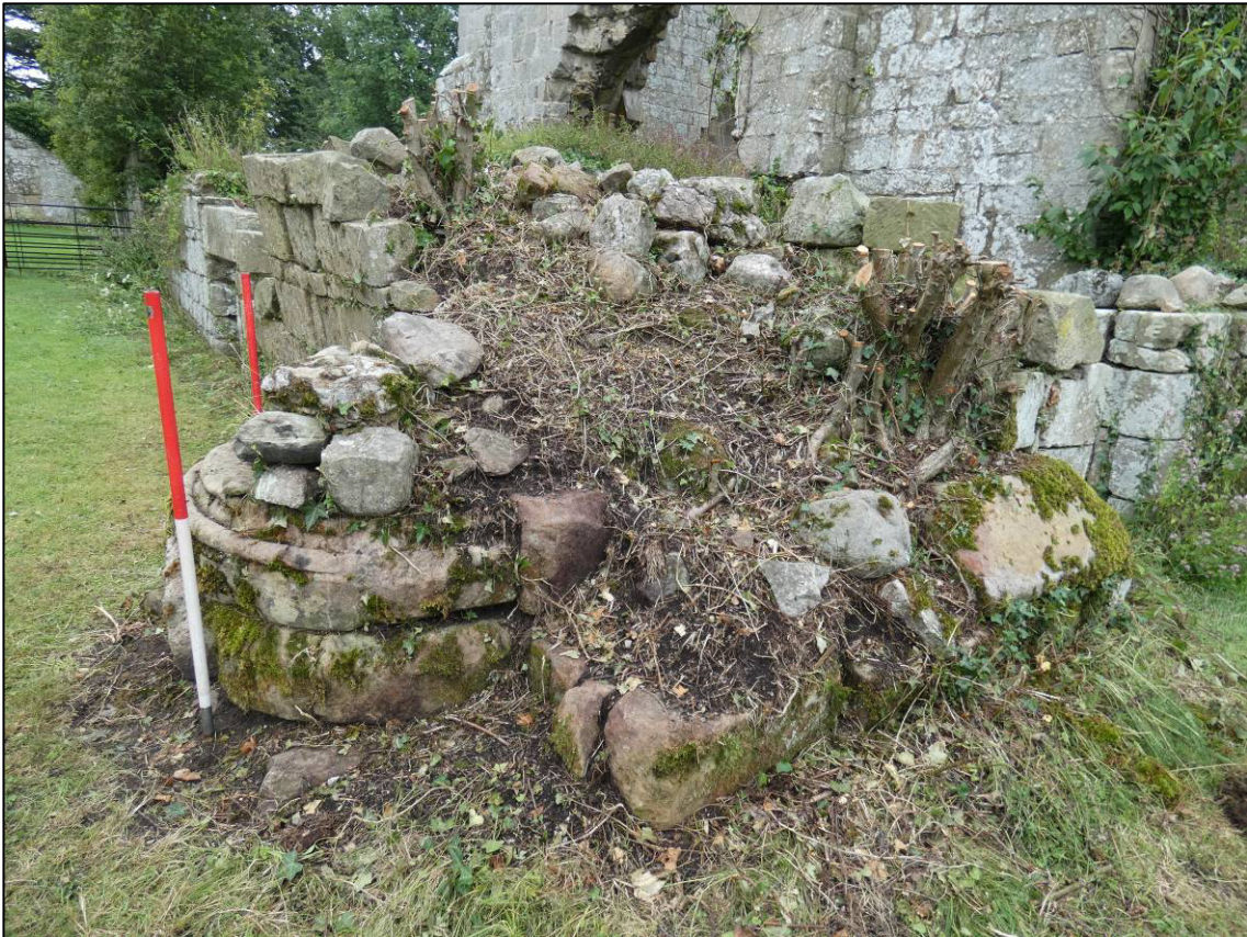
Plate 24: Area 9: Monks' dorter, pier base in west internal elevation of east wall (south end), after clearance, looking N (photo 2/482).
