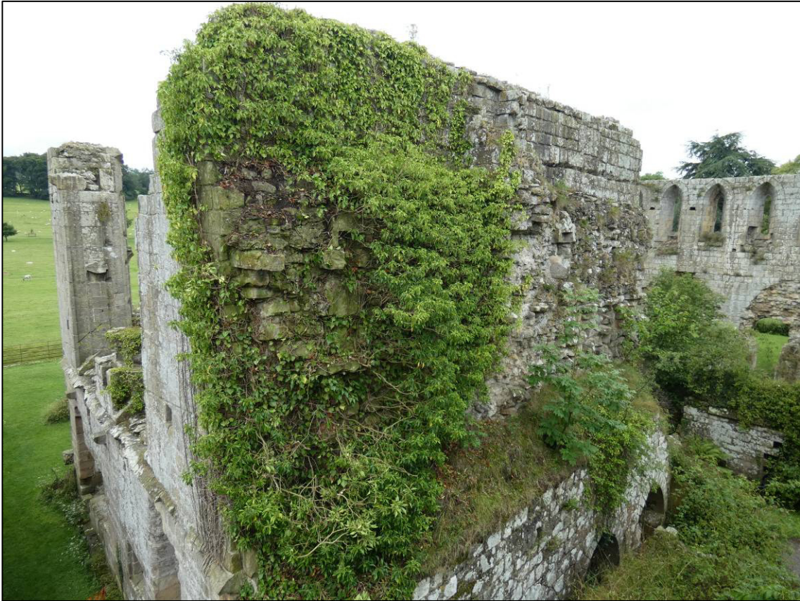
Plate 40: Area 14: Monks' rere-dorter, north internal elevation of south wall (upper level), during clearance, looking SW (photo 2/491).
