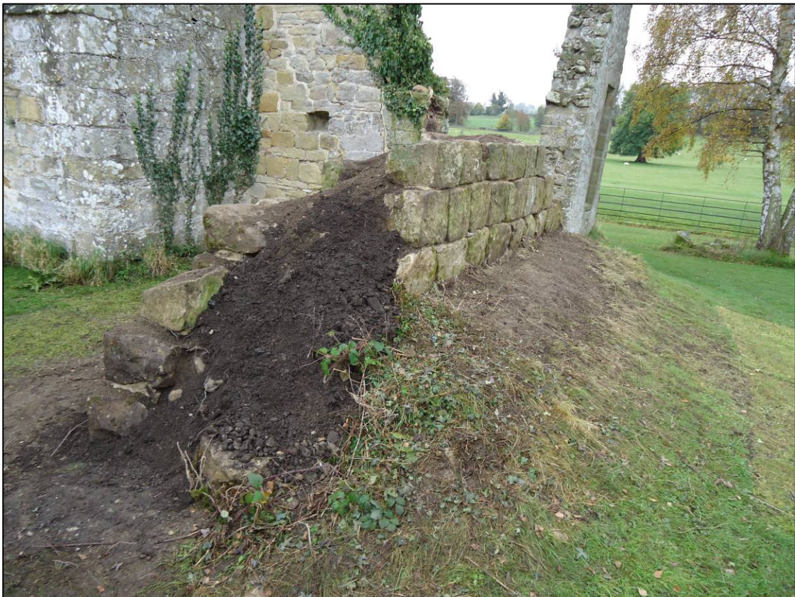
Plate 15: Area 6: Monks' frater, west internal elevation of east wall (south end), after repair, looking SE (photograph courtesy Peter Pace).
