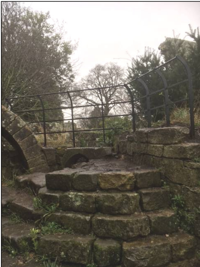
Plate 68: Area 12: Stairs between abbots' lodging and monks' rere-dorter, new fencing to top over drain, looking N (photograph courtesy Historic Property Restoration).
