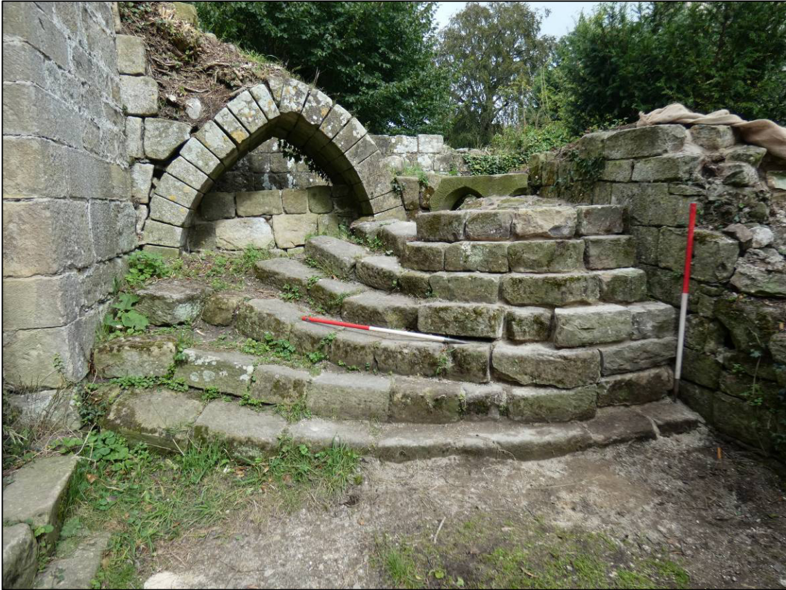
Plate 34: Area 12: Staircase between abbots' lodging and monks' rere-dorter, after repair, looking N (photo 3/557).
