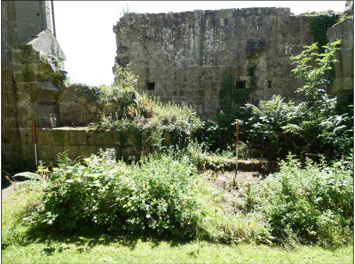
Plate 36: Area 13: Meat kitchen, north internal elevation of south wall, before clearance, looking S (photo 1/330).
