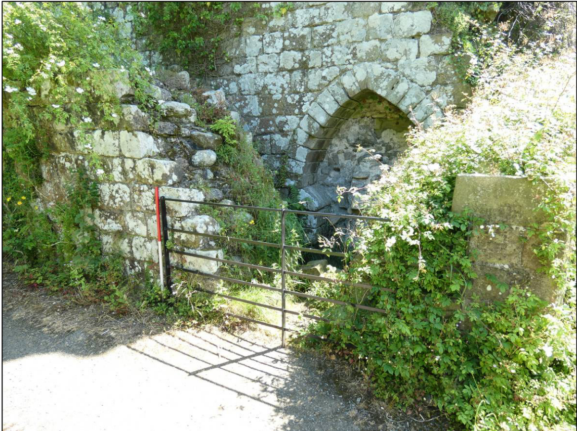
Plate 66: Area 14: Monks' rere-dorter, west end of drain showing older-type fencing, looking SE (photo 1/349).
