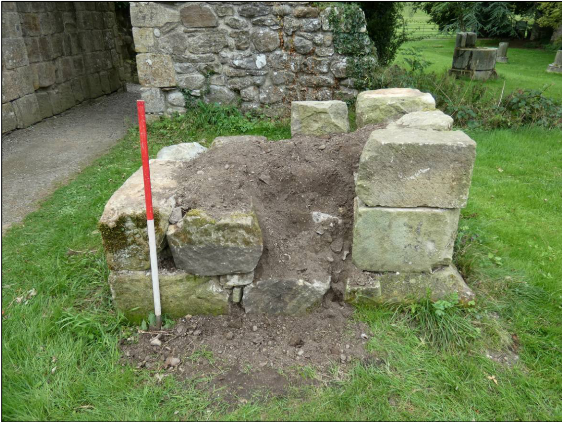
Plate 8: Area 2: Lay brothers' rear-dorter, east end of north wall, during repair, looking E (photo 3/578).
