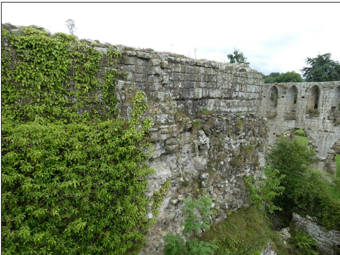
Plate 41: Area 14: Monks' rere-dorter, north internal elevation of south wall (upper level), showing chimney flue from meat kitchen and cut line of former rere-dorter roof, looking SW (photo 2/493).
