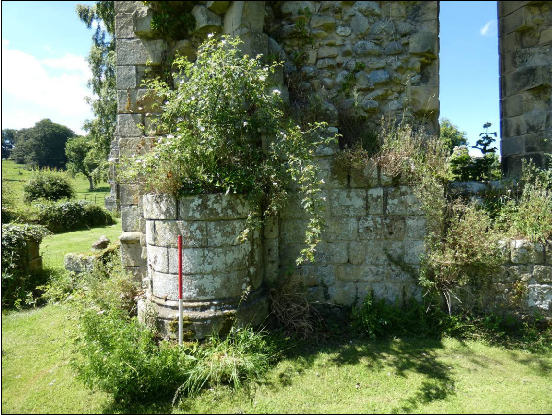
Plate 30: Area 9: Monks' dorter, pier at south end of east internal elevation of west wall, looking W (photo 1/307).
