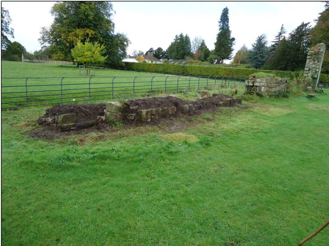
Plate 11: Area 3: Lay brothers' guest house, west wall, during repair, looking NW (photograph courtesy Peter Pace).
