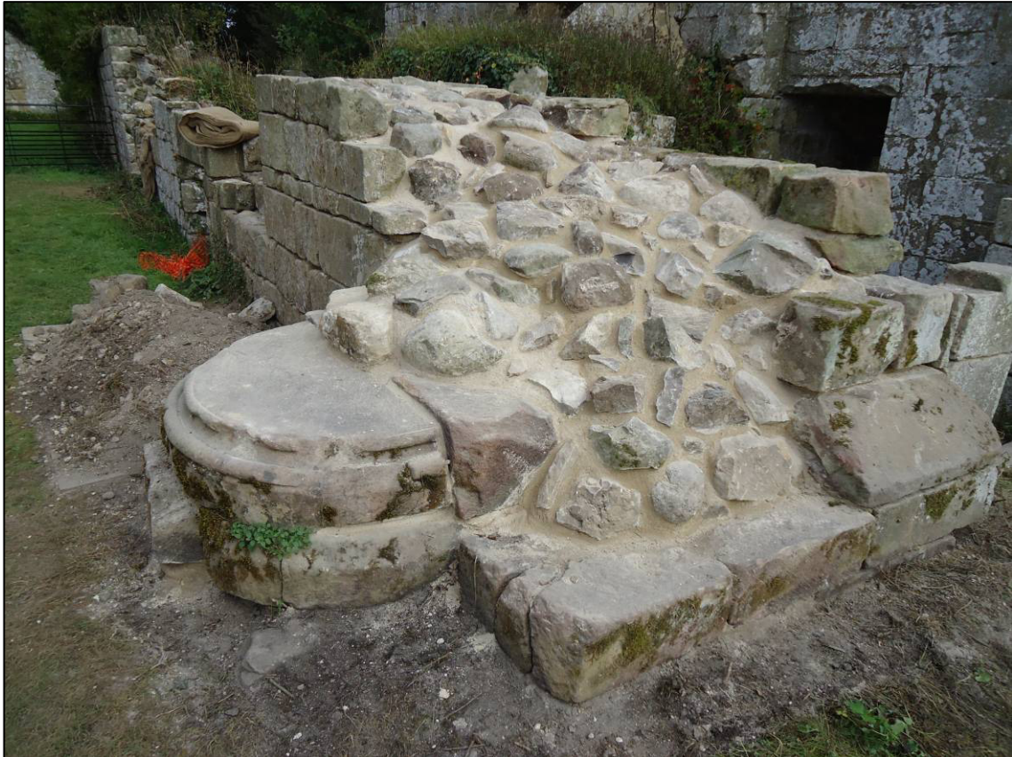
Plate 26: Area 9: Monks' dorter, pier base and west internal elevation of east wall (south end), after consolidation, looking N (photograph courtesy Peter Pace).
