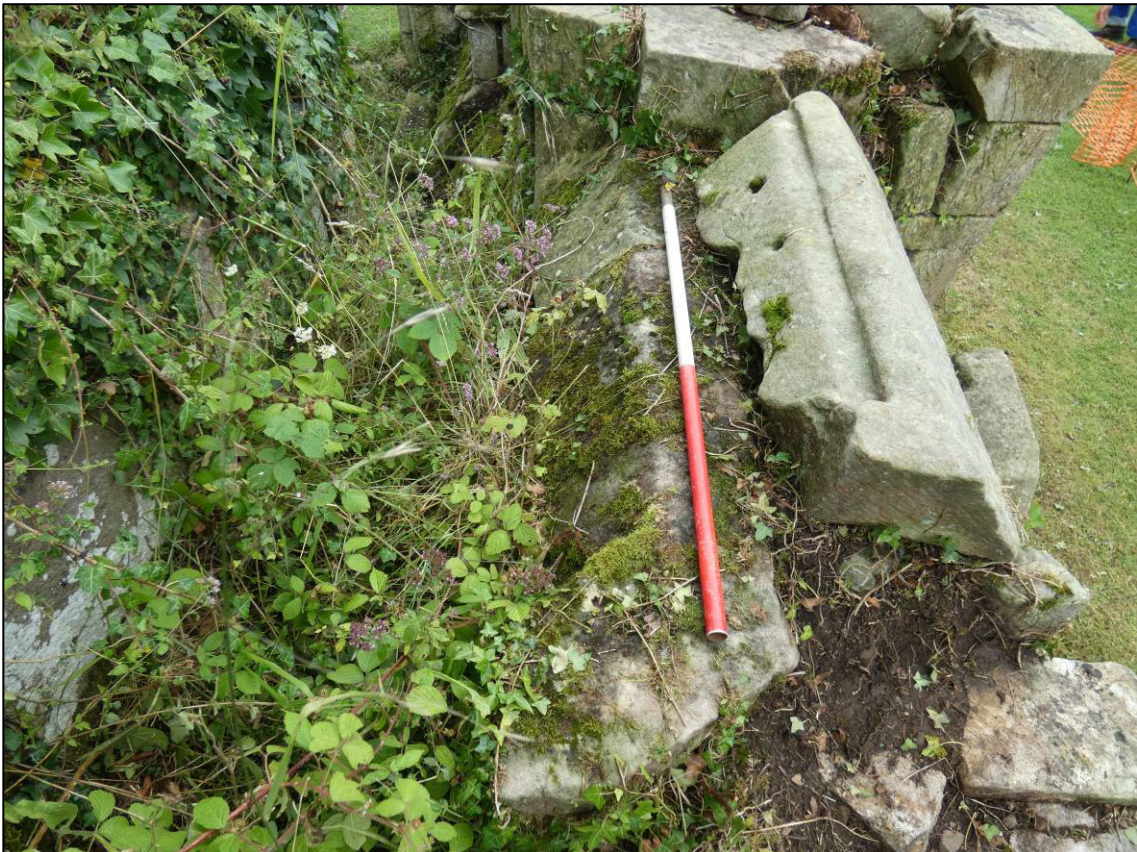
Plate 23: Area 9: Monks' dorter, window sill in west internal elevation of east wall (south part), looking S (photo 2/485).
