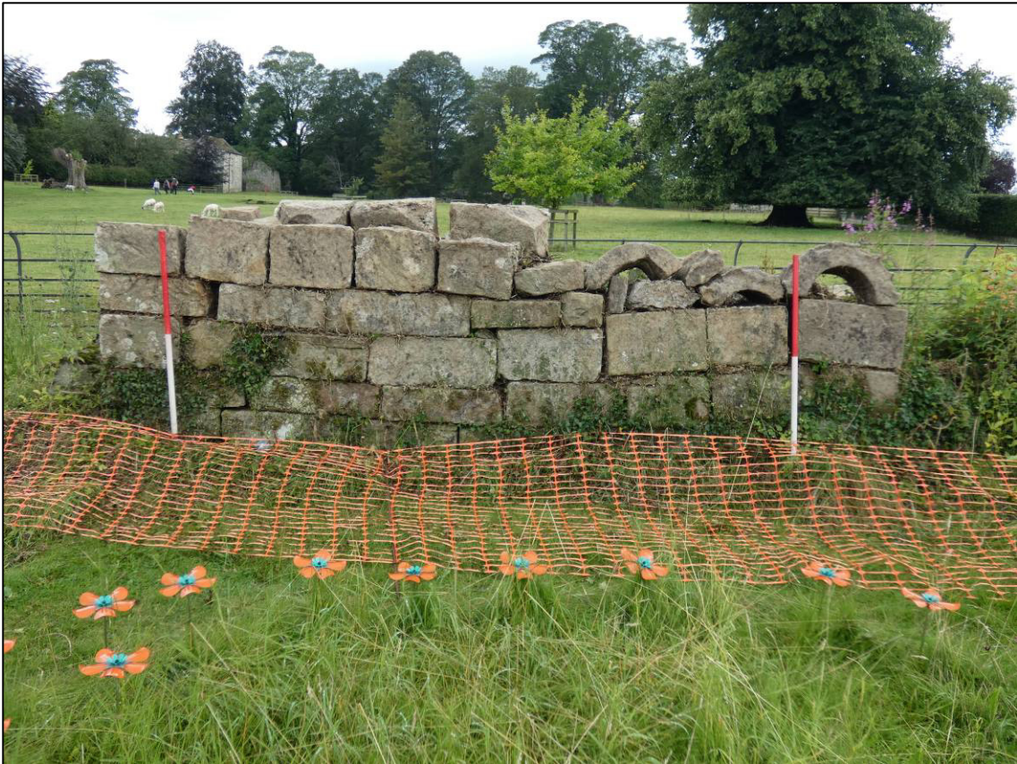
Plate 10: Area 3: Lay brothers' guest house, east internal elevation of west wall (north part), after clearance, looking W (photo 2/466).
