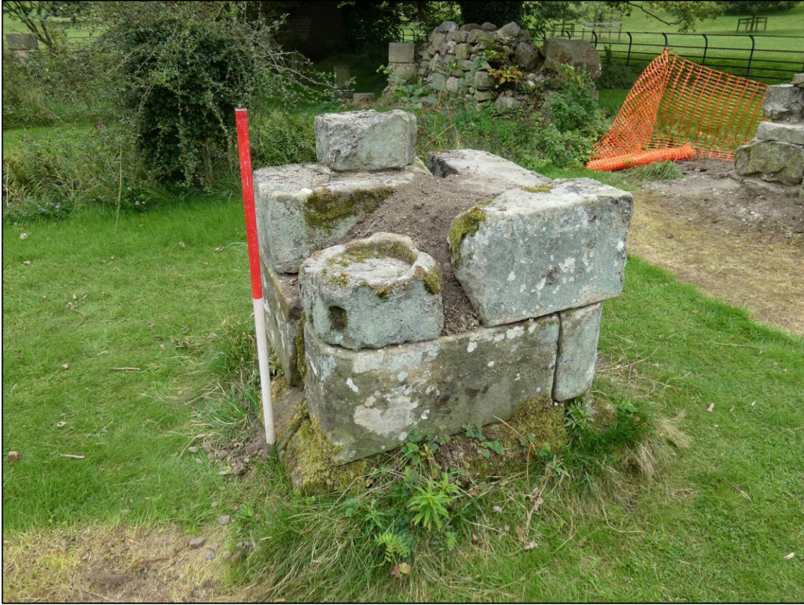
Plate 6: Area 2: Lay brothers' rear-dorter, west pier in north wall, during repair, looking S (photo 3/576).
