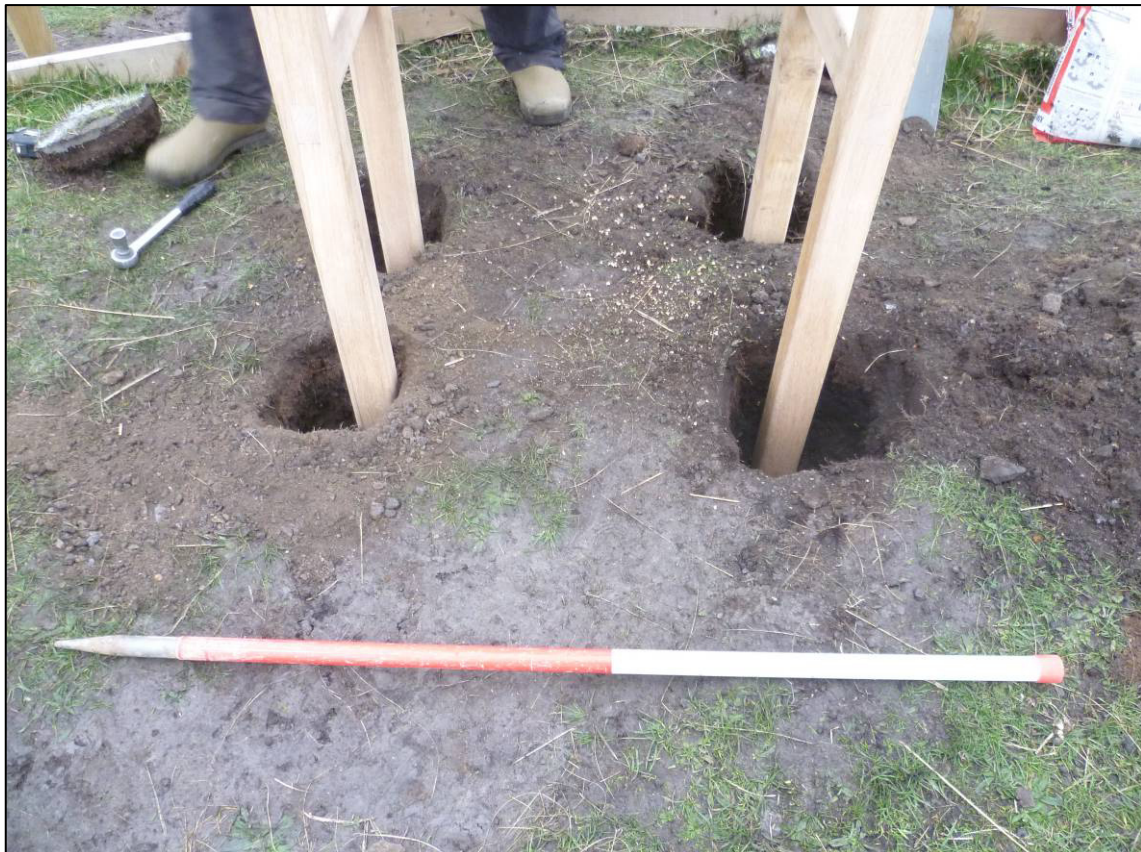
Plate 2: Excavated holes for leg supports, Deep Grove quarry interpretation board, looking W.
