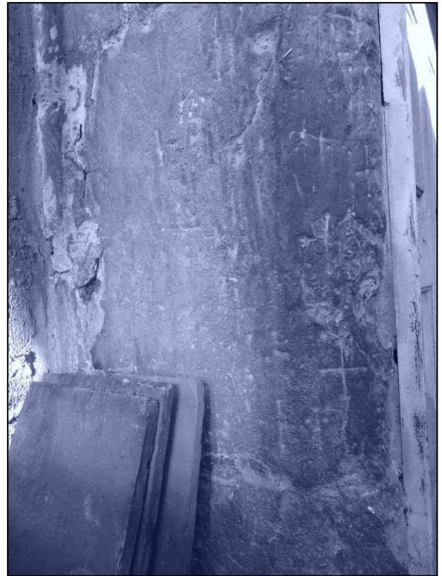
Plate 7: Carved crosses to west jamb of south doorway within porch, looking N.
