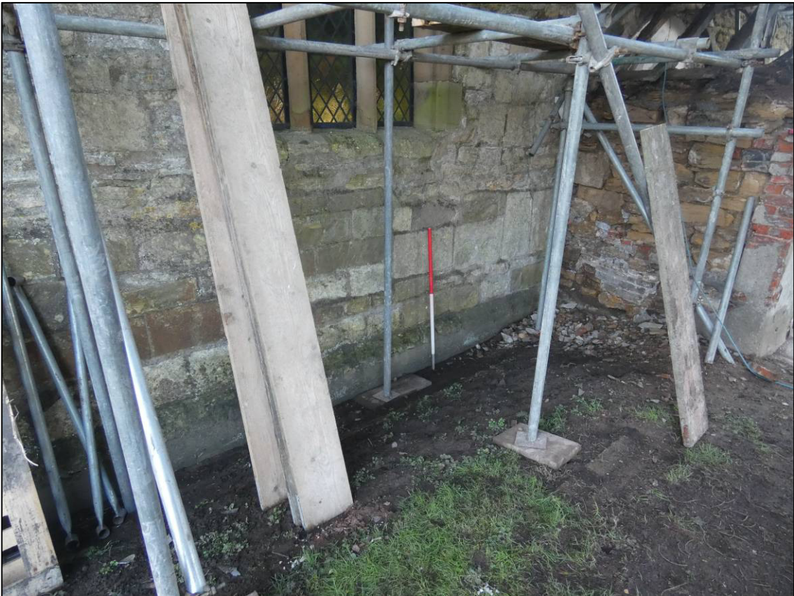
Plate 4: Earlier masonry to north wall of nave, east of the north porch, looking SW.
