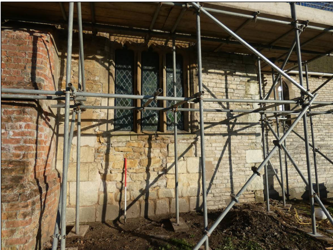
Plate 11: Earlier masonry and blocked opening to south wall of nave, east of brick buttress, looking N.
