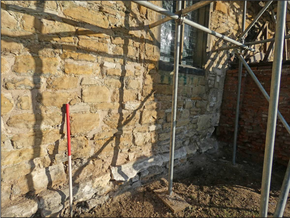
Plate 8: Earlier masonry and blocked opening to south wall of nave, west of south porch, looking NE.
