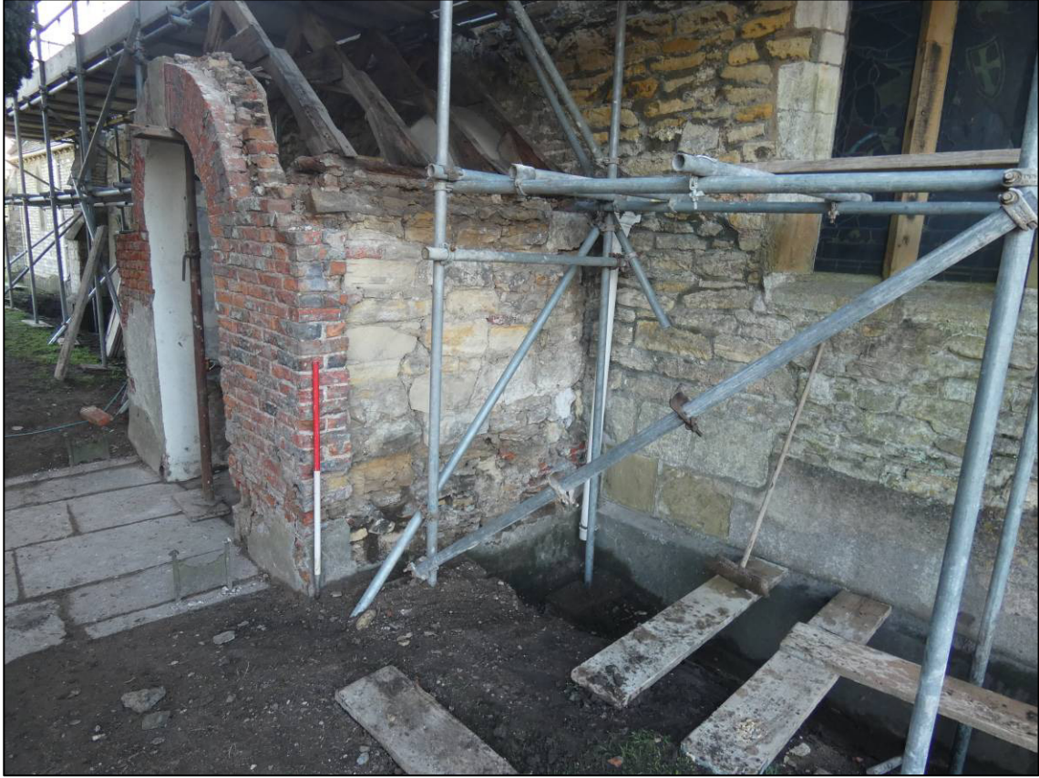
Plate 5: North porch after removal of stucco plaster, showing different fabrics, looking SE.
