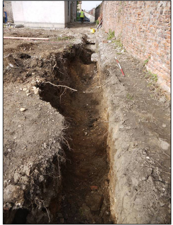
Plate 79: Collapse to south side of Trench 1, looking W.
