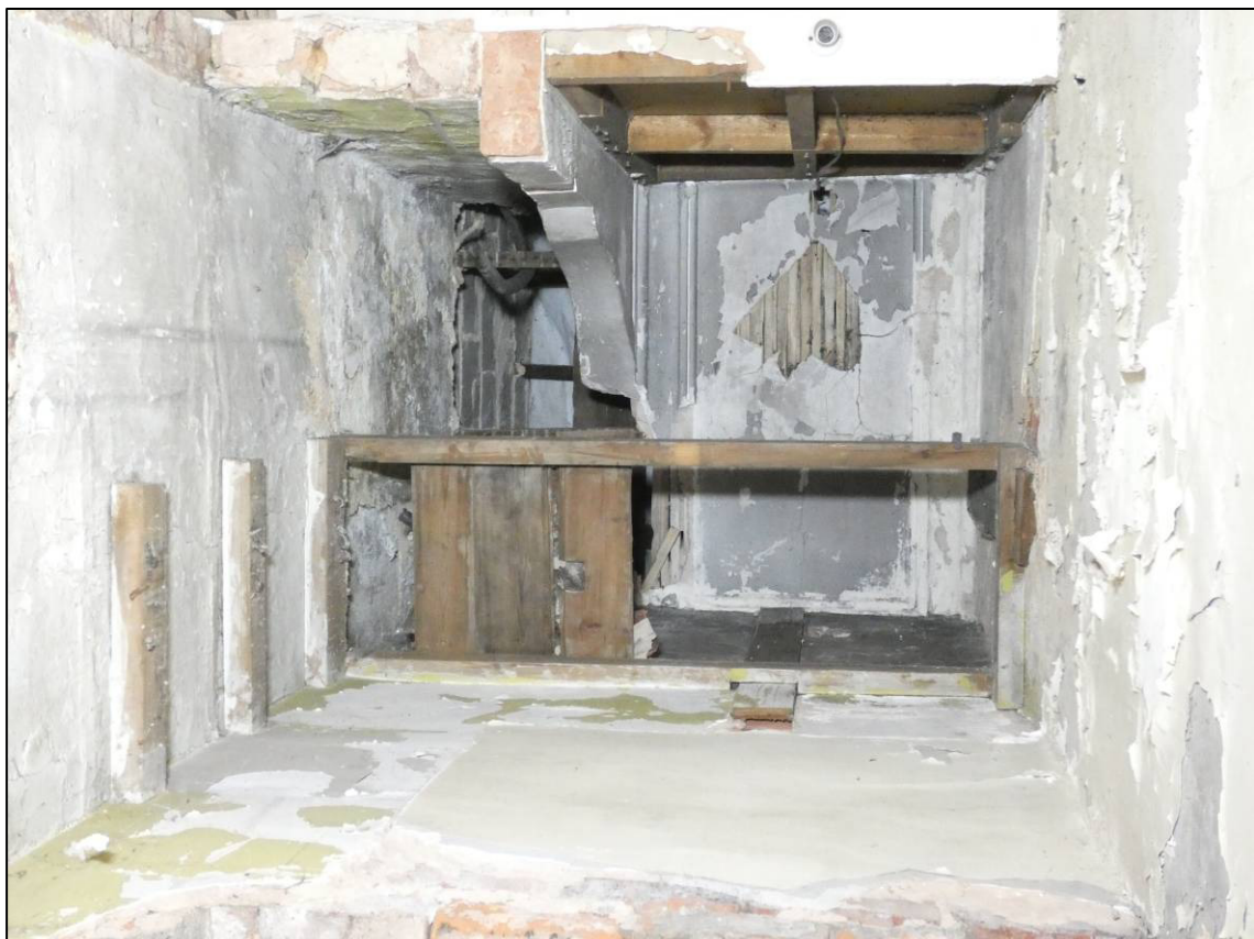
Plate 58: Rear wing first floor, east room (1F8), south-east corner, from GF6, showing remains of ceiling cornice, looking up (photo 2/134).
