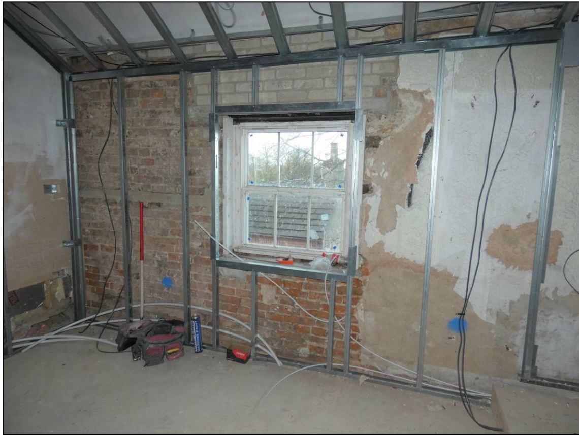
Plate 64: Second floor, south-west room (2F5), west wall after stripping out, looking W (photo 4/491).
