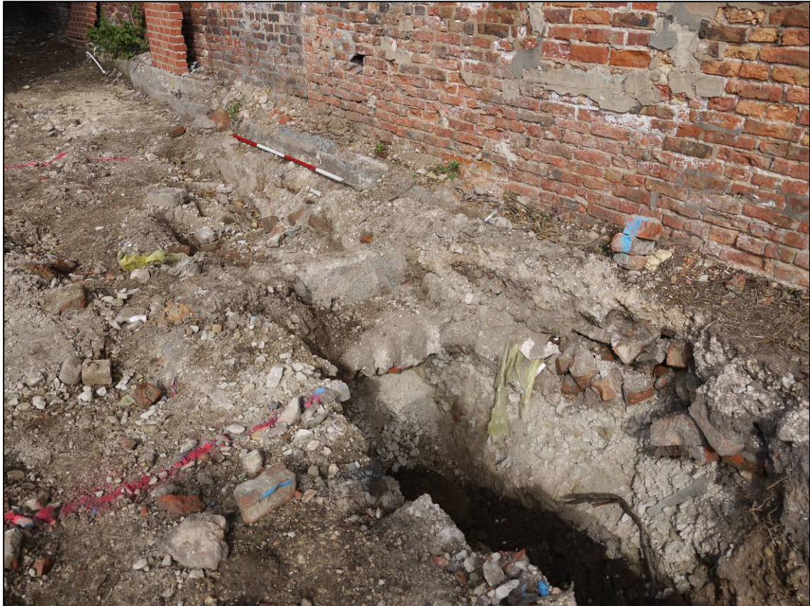
Plate 82: Concrete and brick footings (101) at west end of Trench 1, with brick and stone rubble to east (115/116), looking NW.
