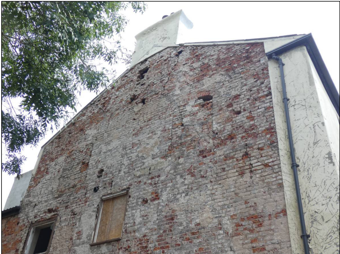
Plate 7: North gable after removal of render, showing blocked openings, looking S (photo 2/328).
