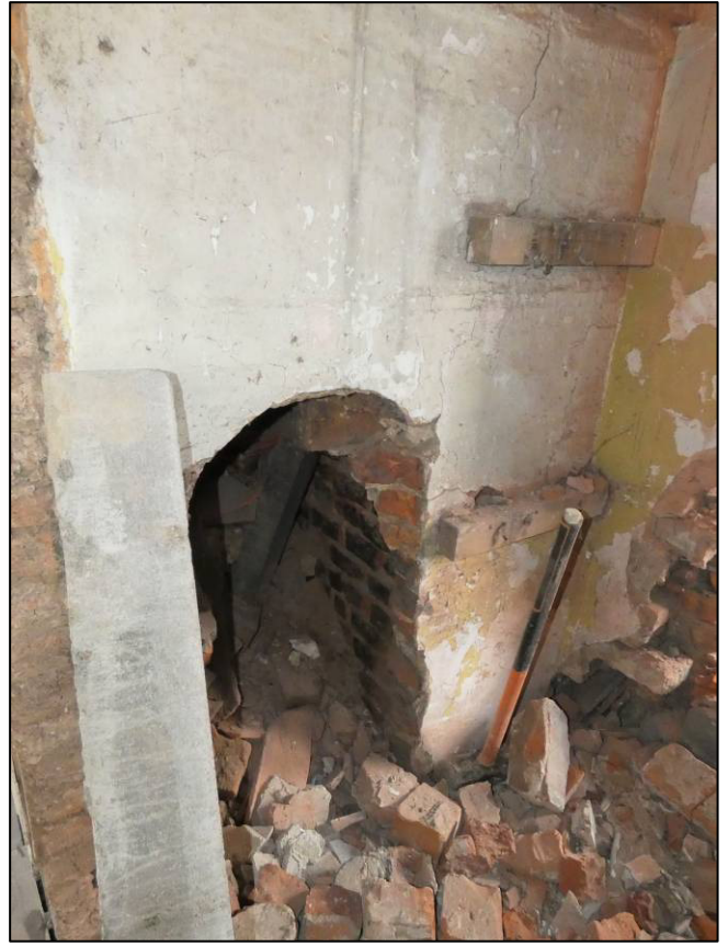
Plate 60: Rear wing first floor, east space (1F8), recess to south side of chimney breast after stripping out, looking N (photo 4/512).
