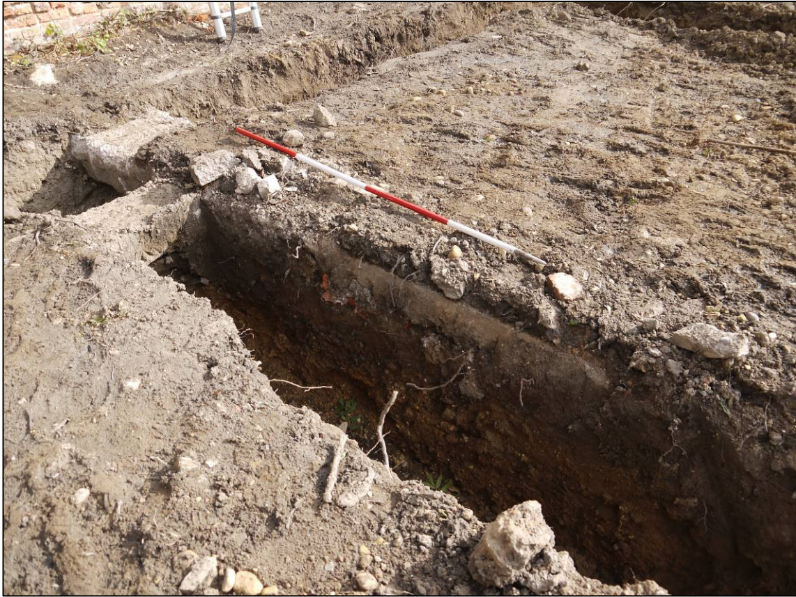
Plate 83: Concrete foundations (103) exposed at junction of Trenches 1 and 6, and along Trench 6, looking NE.
