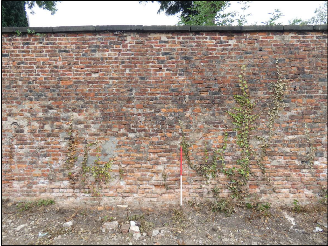
Plate 70: Rear yard, east part of north boundary wall, showing changes in build, looking N (photo 1/963).
