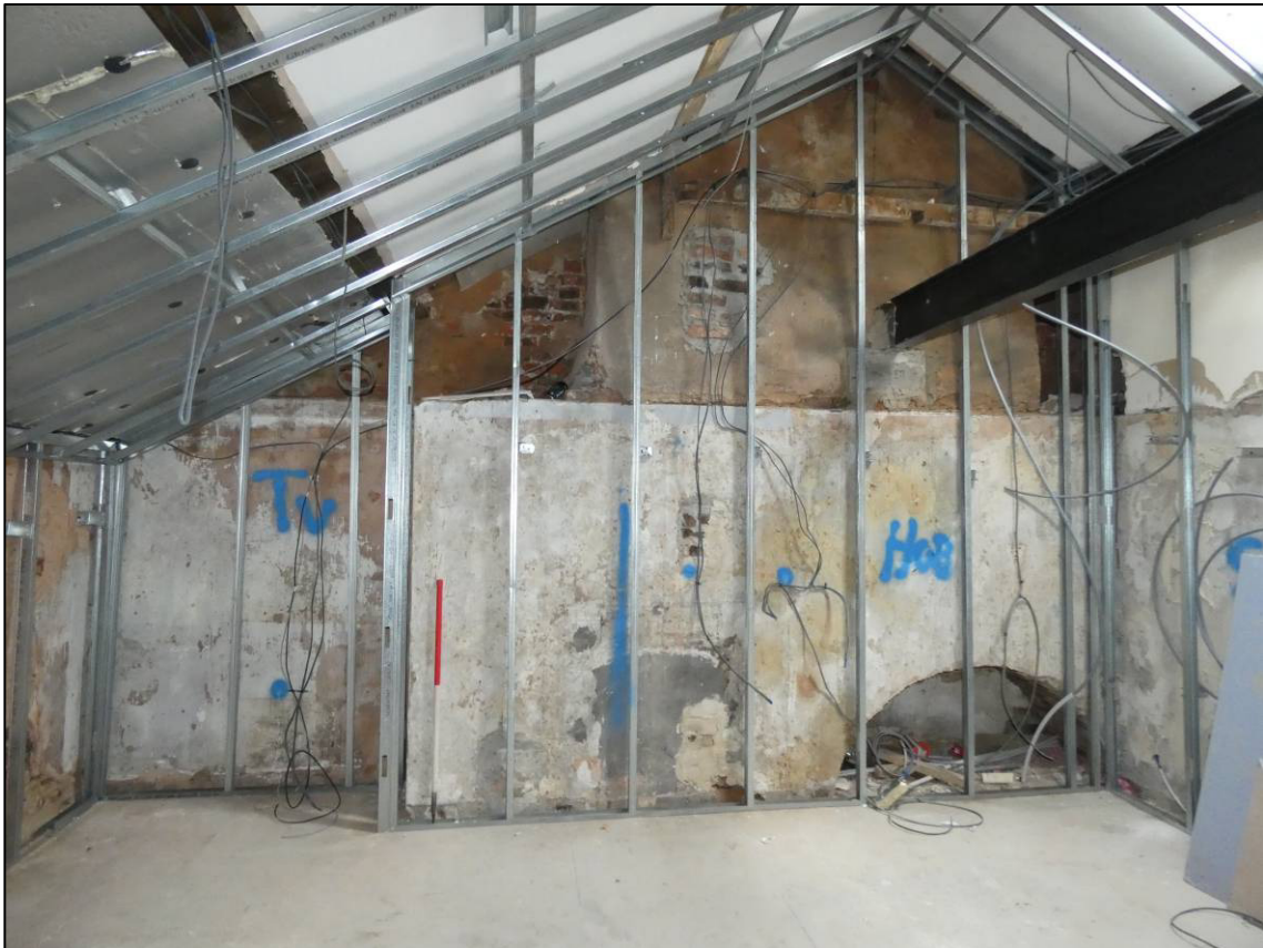
Plate 65: Second floor, north room (2F4), north wall after stripping out, showing blocked fireplace and curved recess, looking N (photo 4/502).
