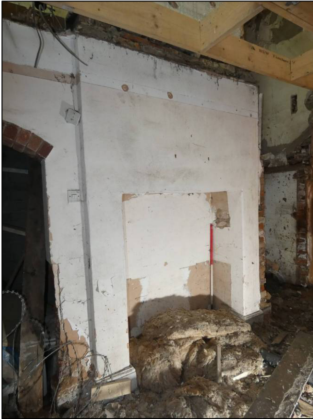
Plate 39: Rear wing ground floor, east room (GF6), fireplace to east wall, looking SE (photo 2/116).
