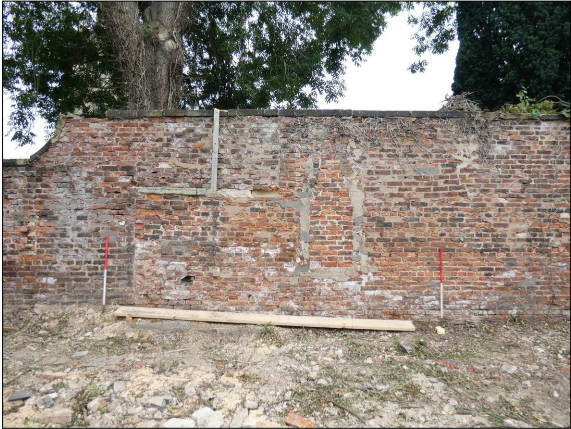
Plate 68: Rear yard, central part of north boundary wall, showing areas of blocking and repair, looking N (photo 1/965).
