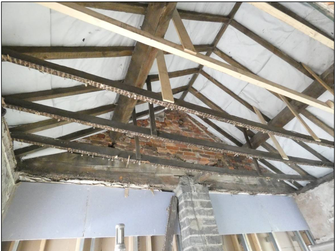
Plate 61: Rear wing first floor, east space (1F8) roof structure after stripping out, looking W (photo 4/517).
