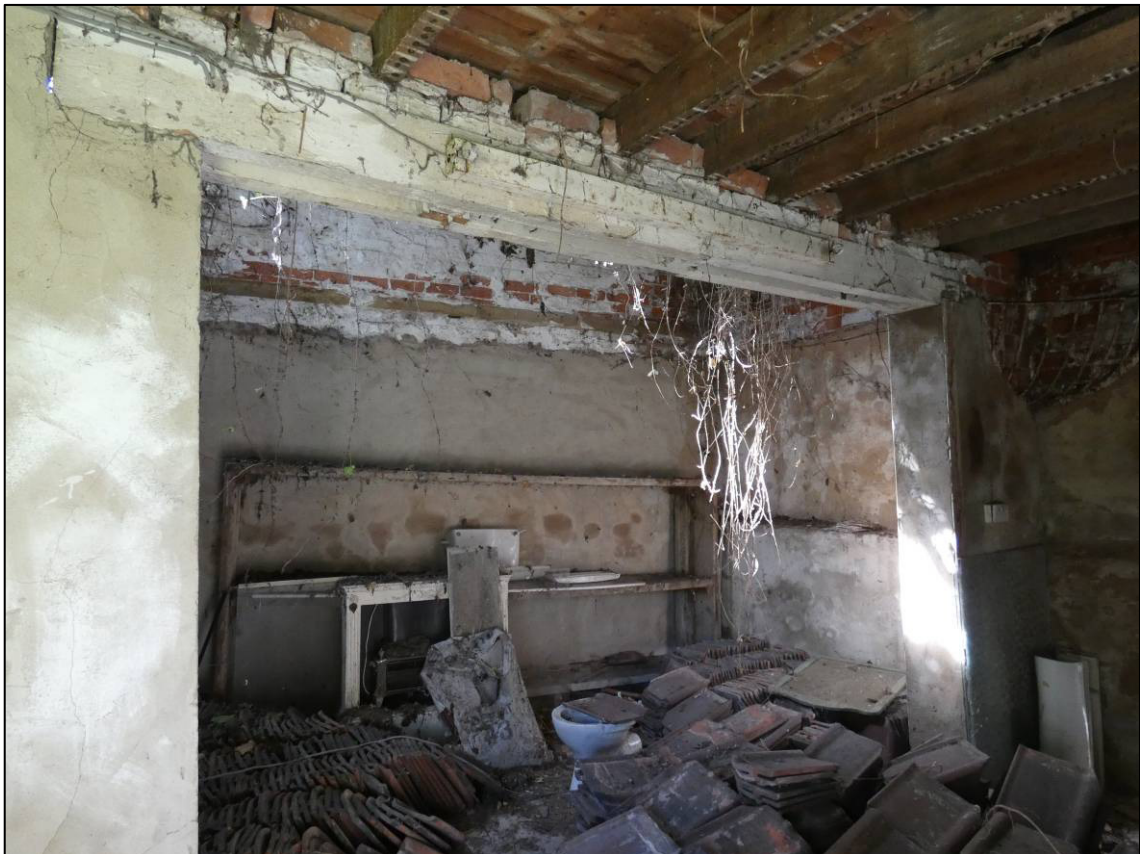
Plate 77: Former coach house/stable, interior, prior to collapse (March 2020), looking NW.
