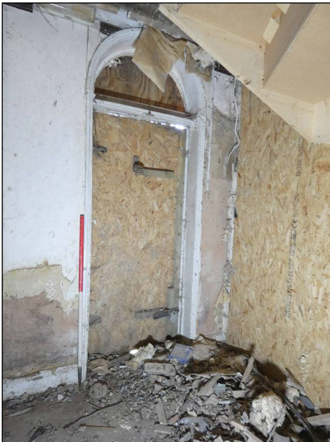
Plate 37: Ground floor lobby (GF4), external door to east wall, looking SE (photo 2/107).
