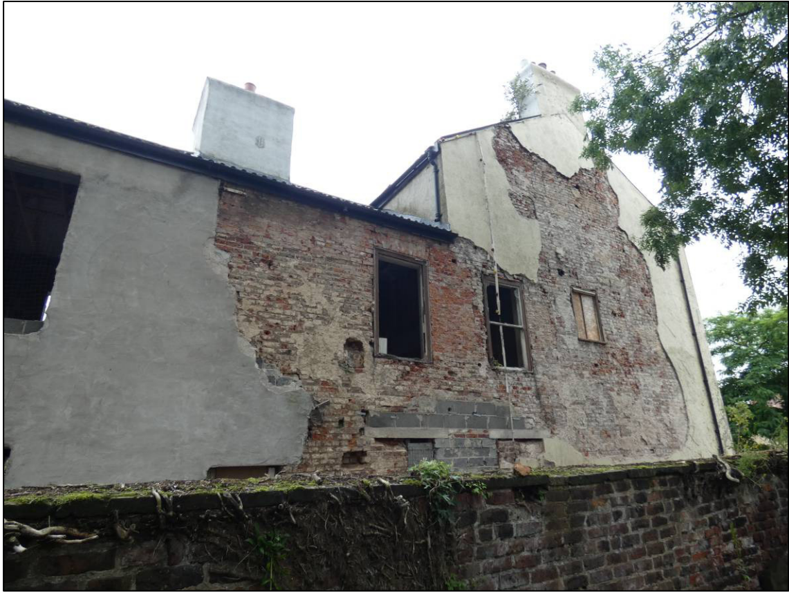
Plate 6: North elevation of rear wing, during removal of render, looking SW (photo 1/014).
