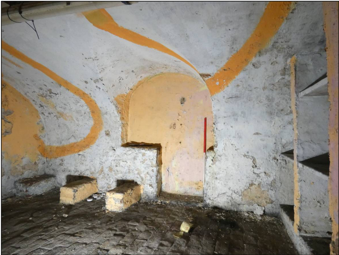
Plate 15: Cellar room C2, opening and brick piers to east wall, looking E (photo 1/095).
