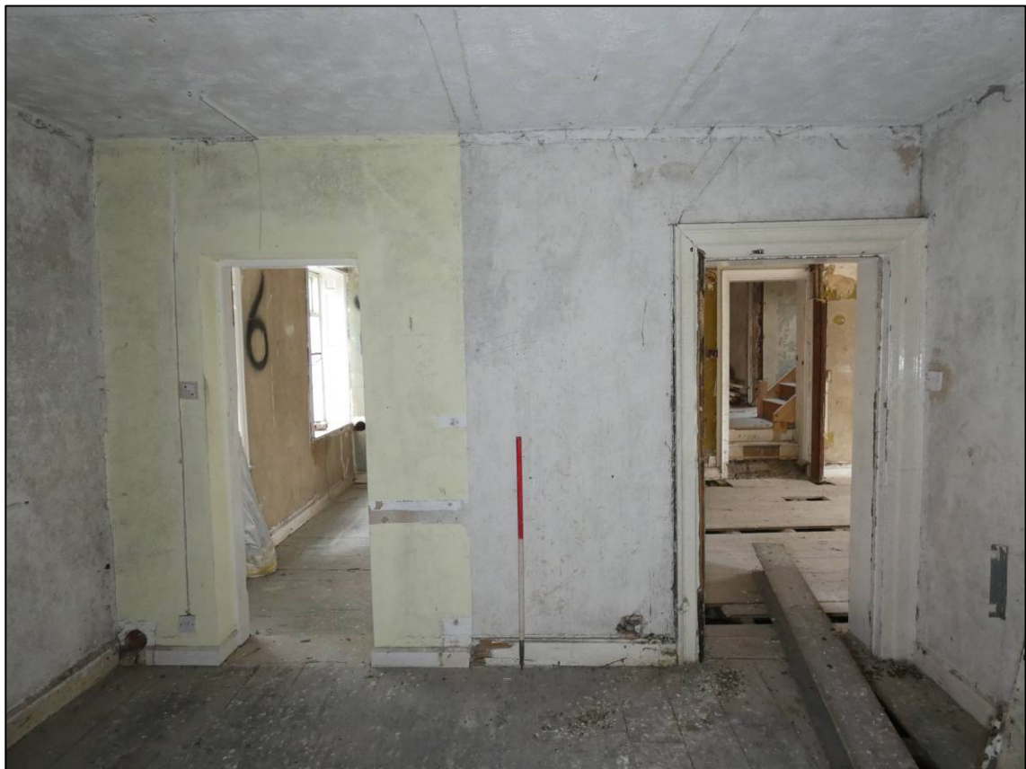
Plate 51: First floor south-west room (1F3), north wall showing inserted door to left, looking N (photo 2/283).
