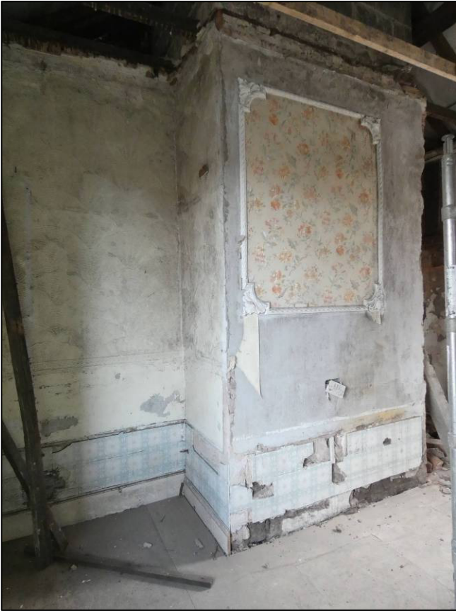
Plate 59: Rear wing first floor, east space (1F8), chimney breast to east wall after stripping out, looking SE (photo 4/514).
