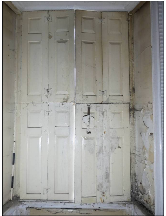
Plate 28: Ground floor north room (GF1), south window to west wall, showing shutters (closed), looking W (photo 1/081).
