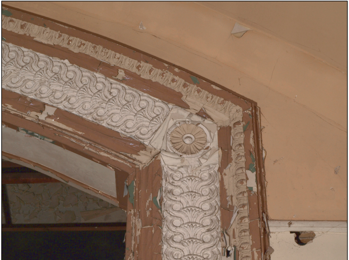
Plate 8: Detail of moulding around proscenium arch of first floor stage, looking N (photo 6/35).
