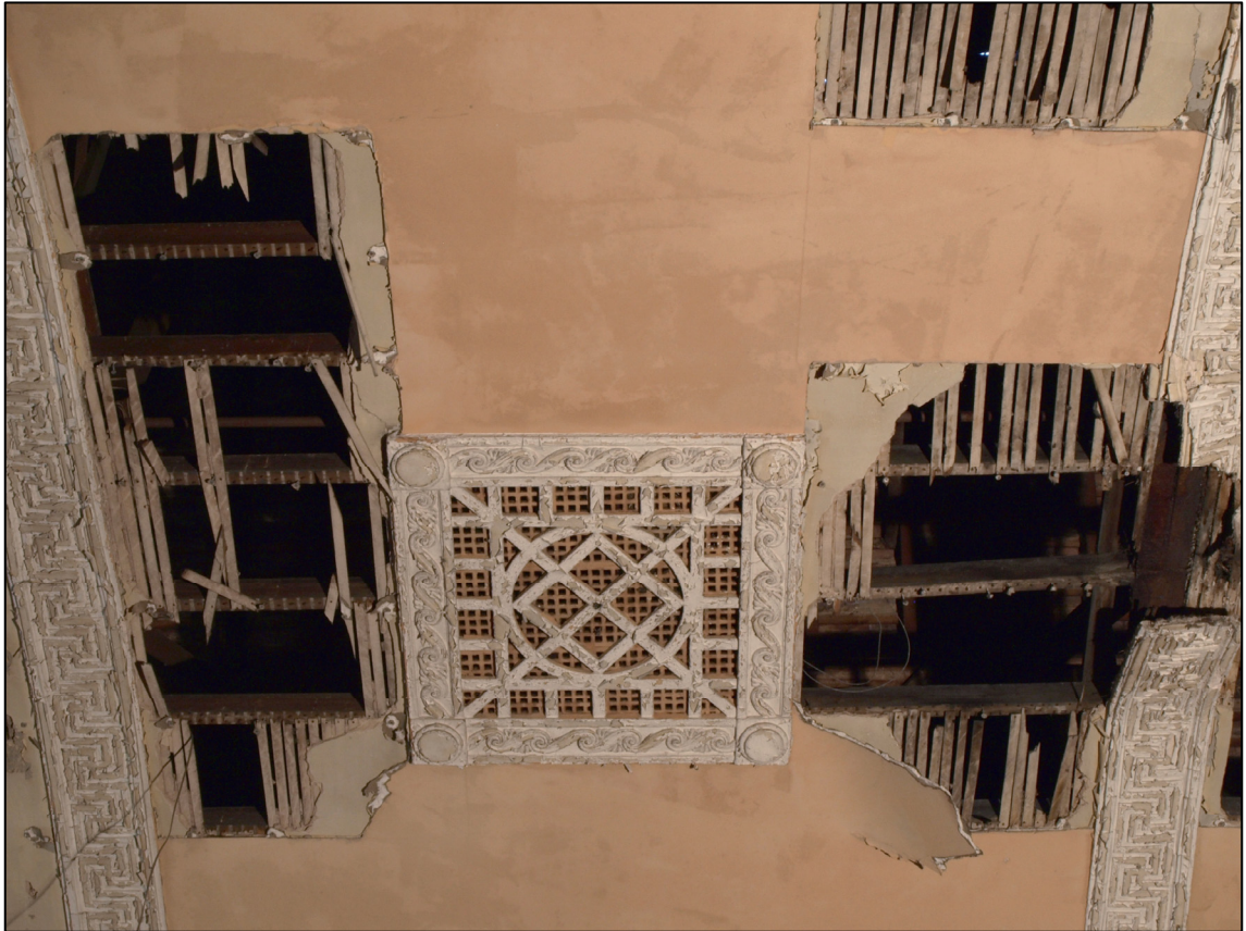
Plate 7: Detail of plaster moulding to ceiling vent over first floor auditorium (photo 6/37).
