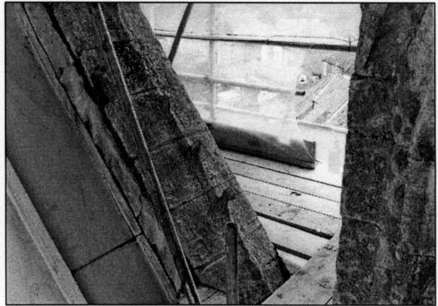
Photo 1/11: Crocketing to coping of west front gable, looking SW.
