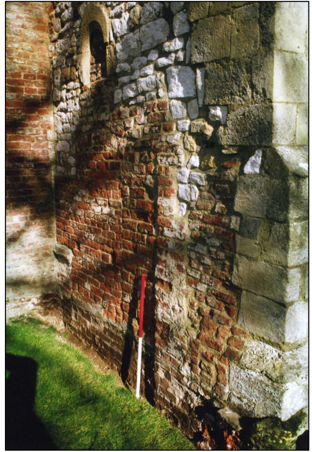
Plate 5: Blocked features and stub wall in west end of south aisle, looking north-east.
