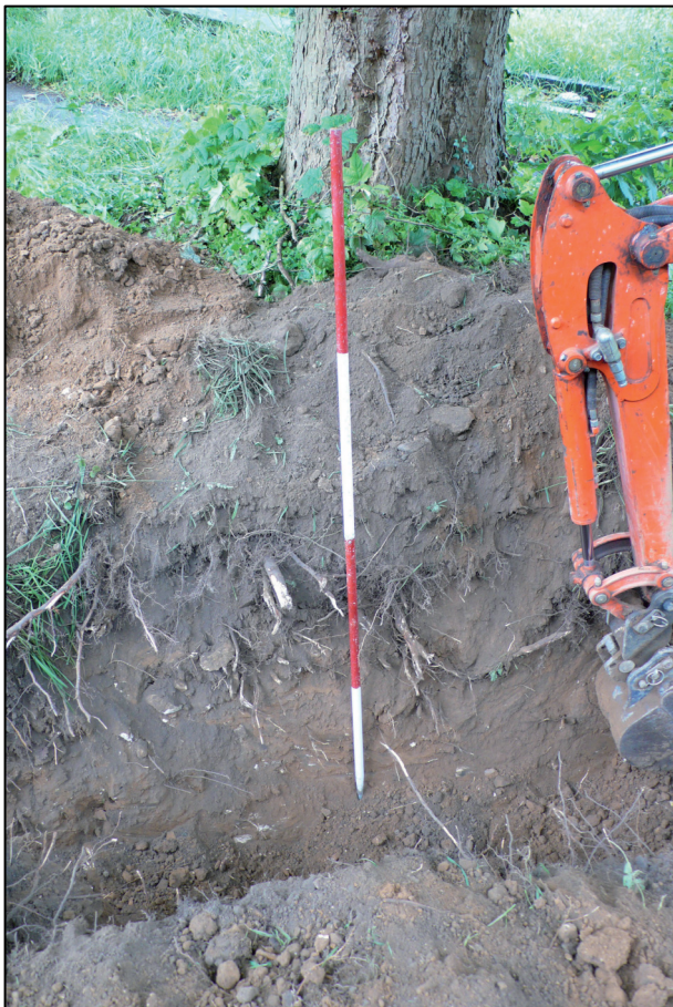
Plate 3: South side of soakaway pit, showing root damage, looking S.
