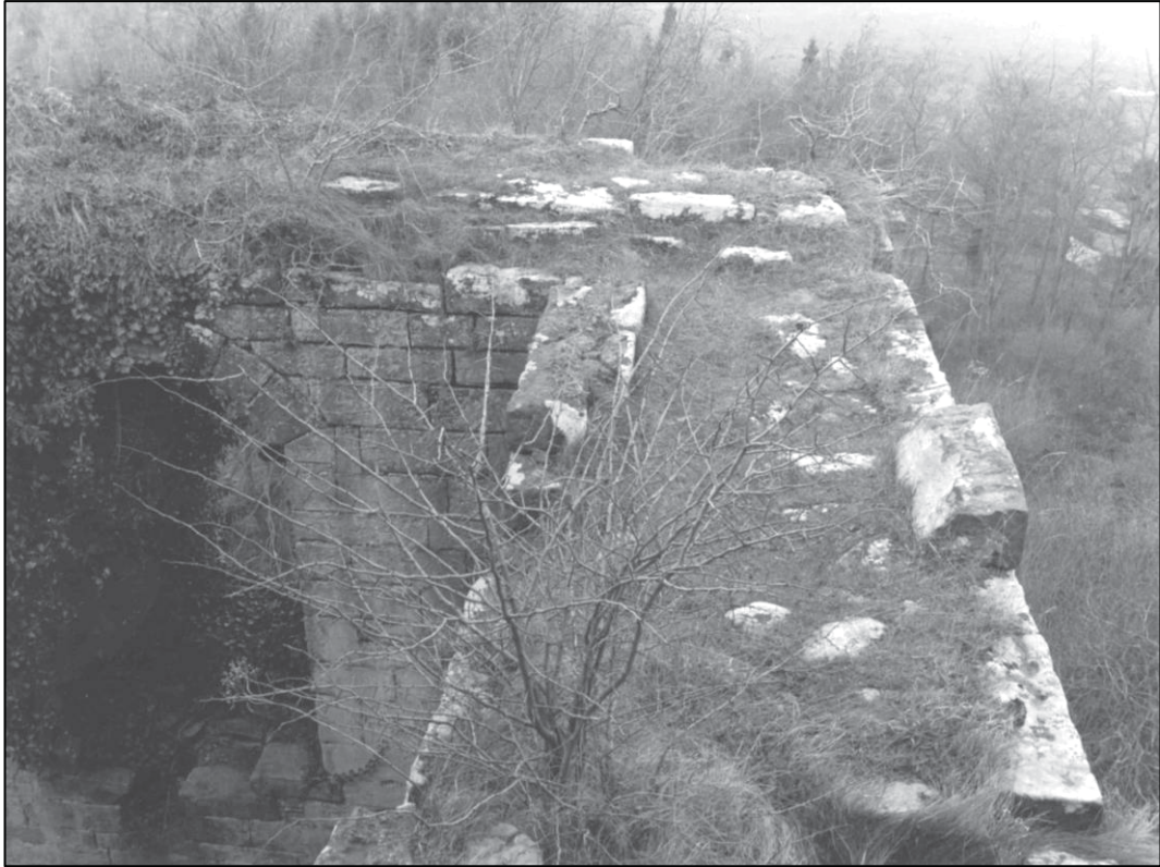
Plate 34: View across wall top of east side of north wing, looking north-west (May 2000).
