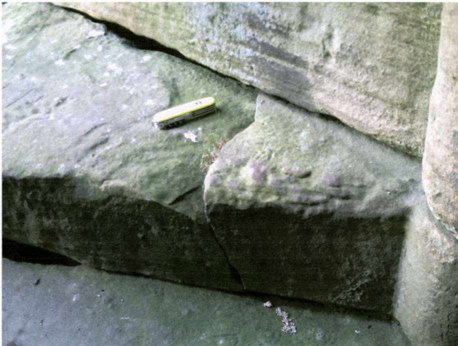
Figure 2. Failure of a slab forming a step in the north east spiral staircase.
