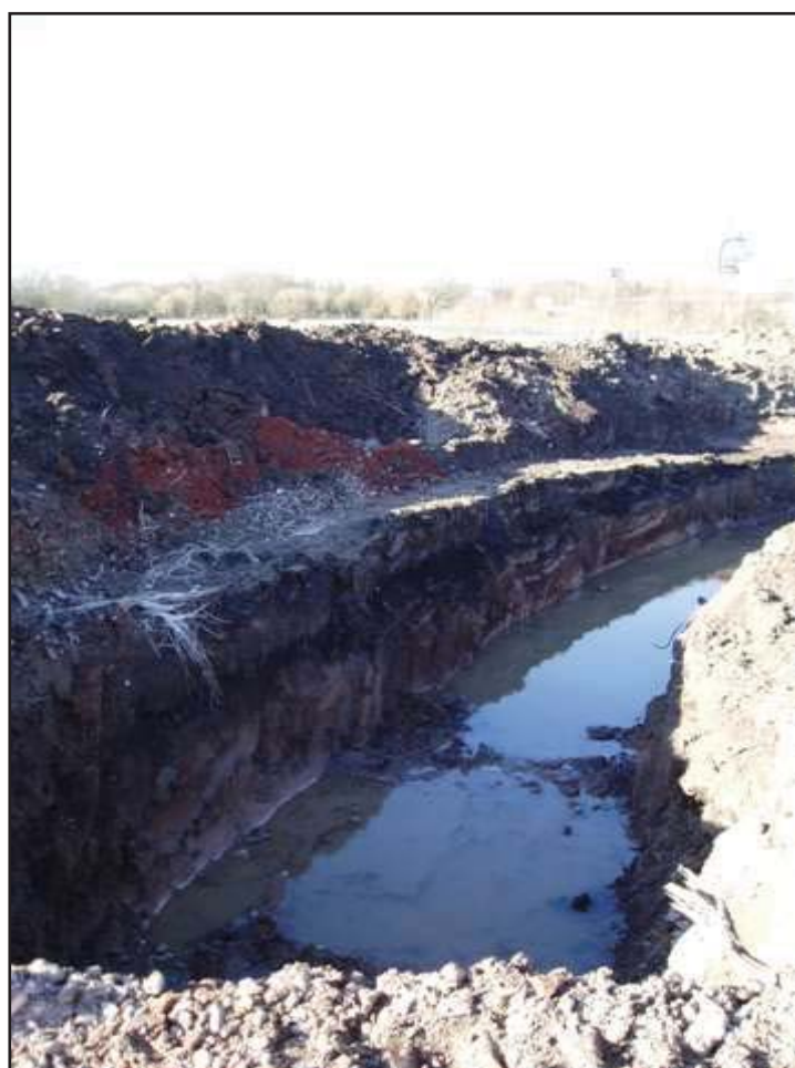
Plate 2: Excavation of Trench 5 to the South of Trench 4; Looking Northeast. No Scale.
