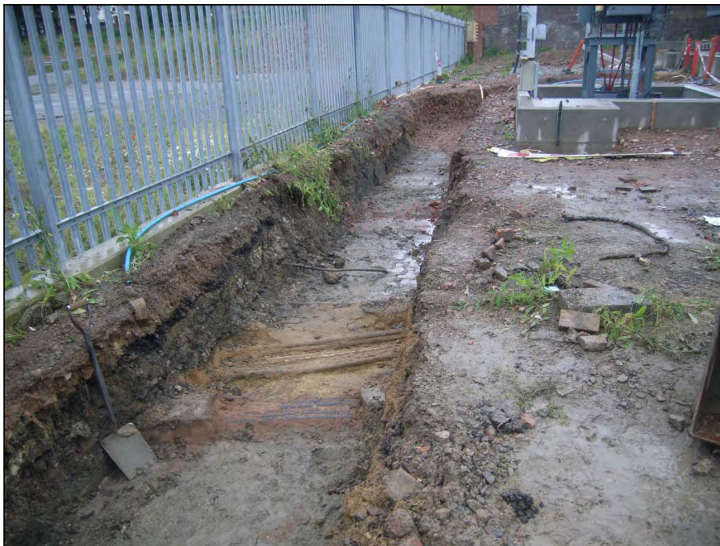
Plate 5: Western half of Trench 12 looking southwest, cables visible in base of trench (No scale).
