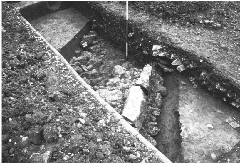
Fig. 7: Sewer diversion area B - remnant of wall 17 (right hand side) over rubble foundations (19). Facing S.
