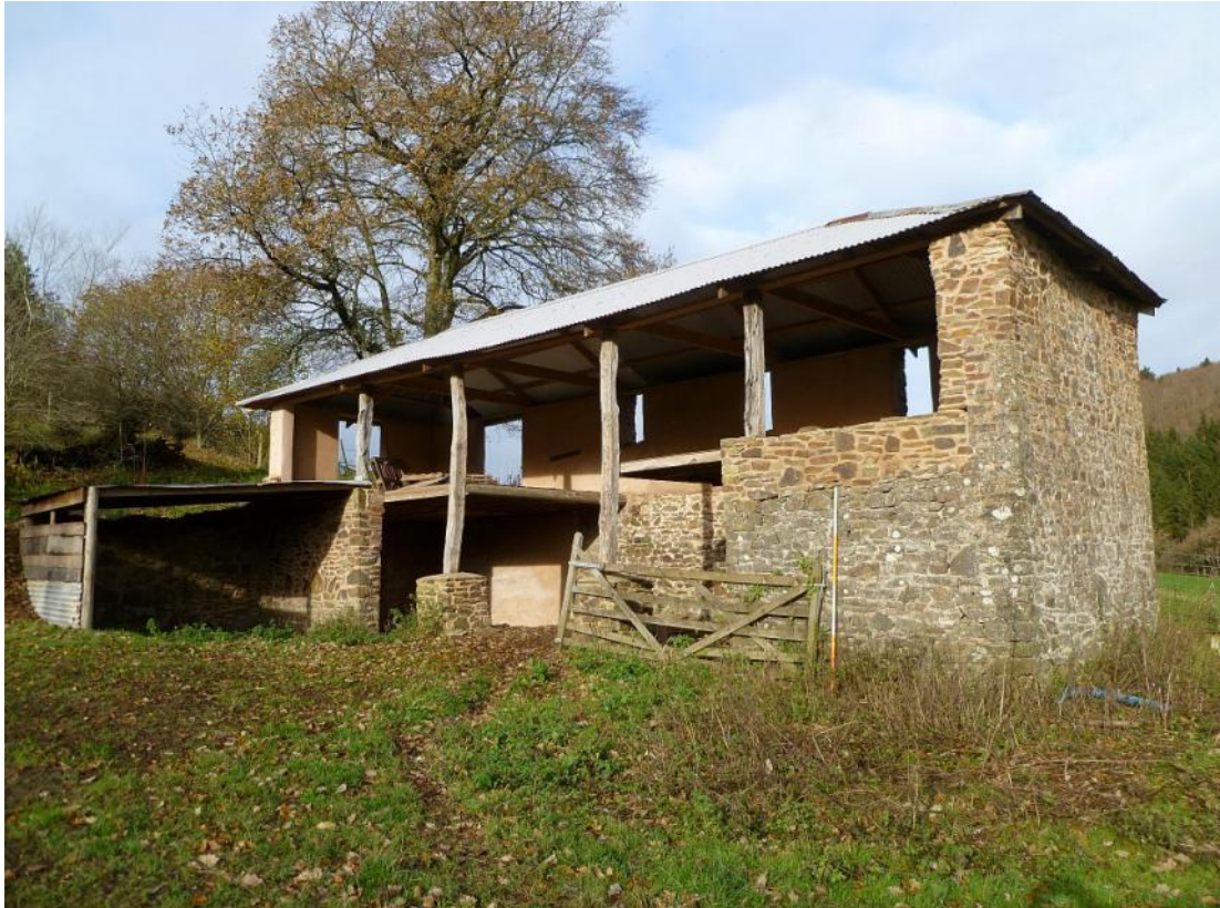
Westercombe linhay from the south east. Note areas of rebuilt masonry
