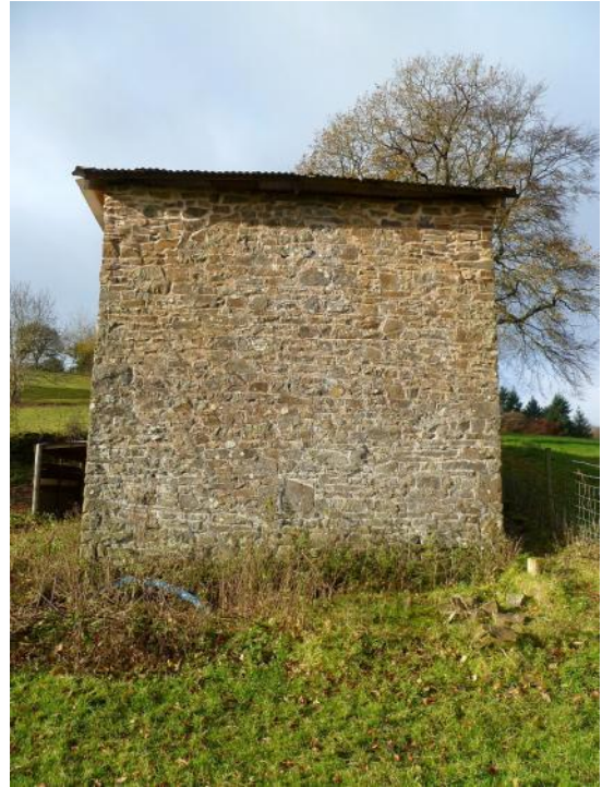
East gable end; note rebuilt masonry
