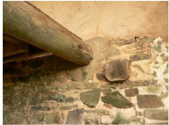
Original cross beam end and replacement first floor beam in rear wall of centre bay
