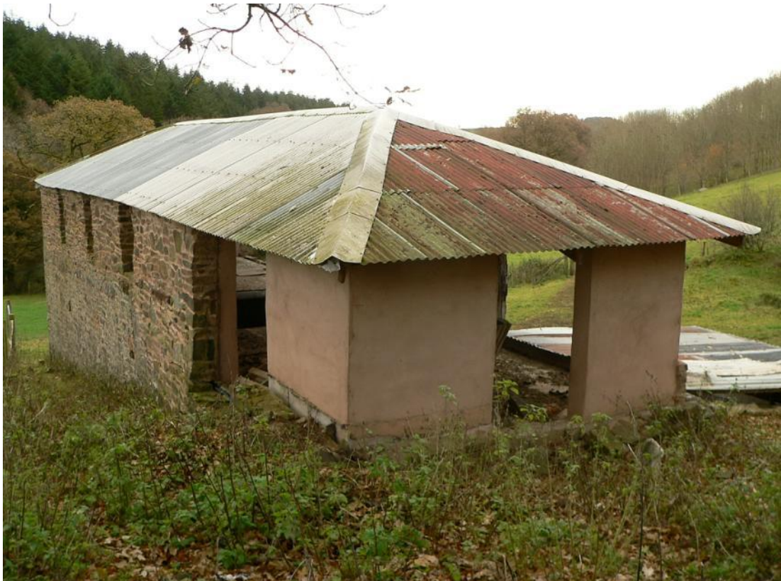
Linhay from the north west, showing extent of rebuilt rendered concrete block walling
