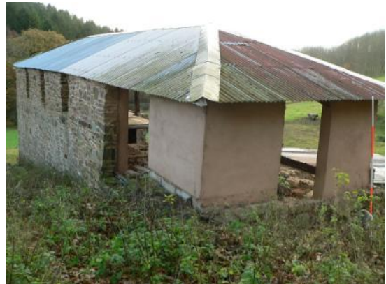
North wall - top of stonework rebuilt - and west gable, rebuilt in rendered concrete block
