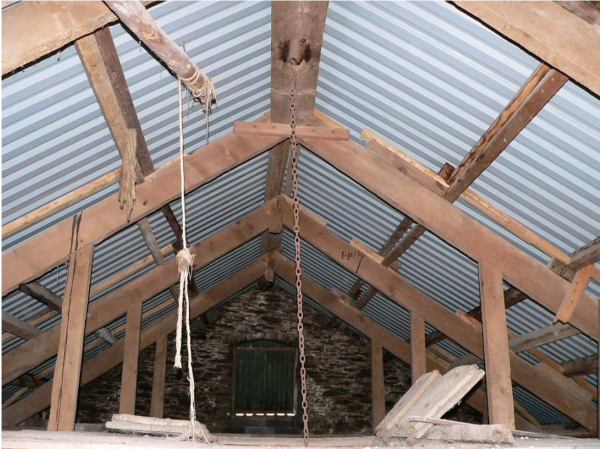
Roof structure, looking north, with sack chain to centre above gallery floor
