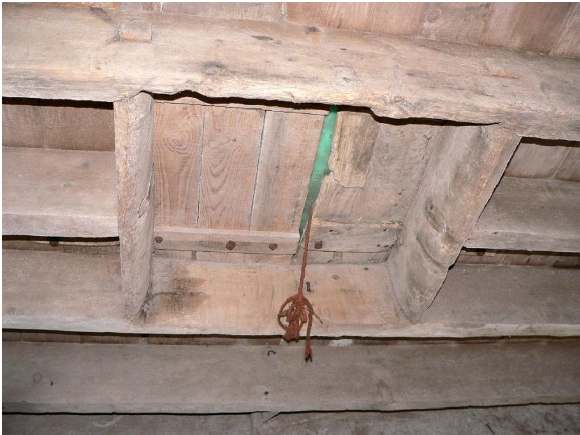
Sack trap opening in first floor. Note chain abrasion on trimmers
