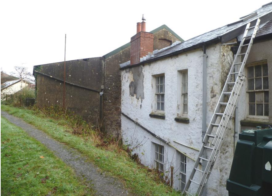
Heddon Mill: rear of villa and mill, showing south gable and extension over intake pit
