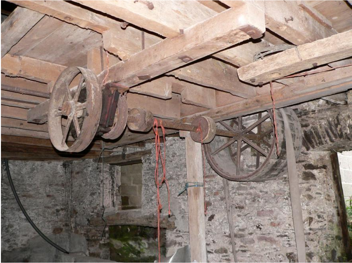
Layshaft and pulleys below first floor ceiling
