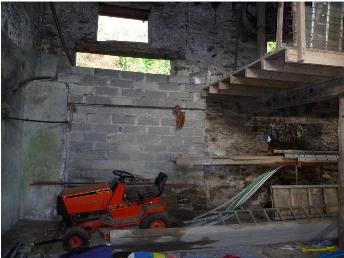
Interior view of blockwork wall to intake pit, south end of ground floor looking west
