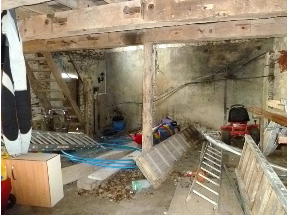
Ground floor looking south, showing ceiling beams with mortises and positions of timbers that formerly supported three pairs of millstones
