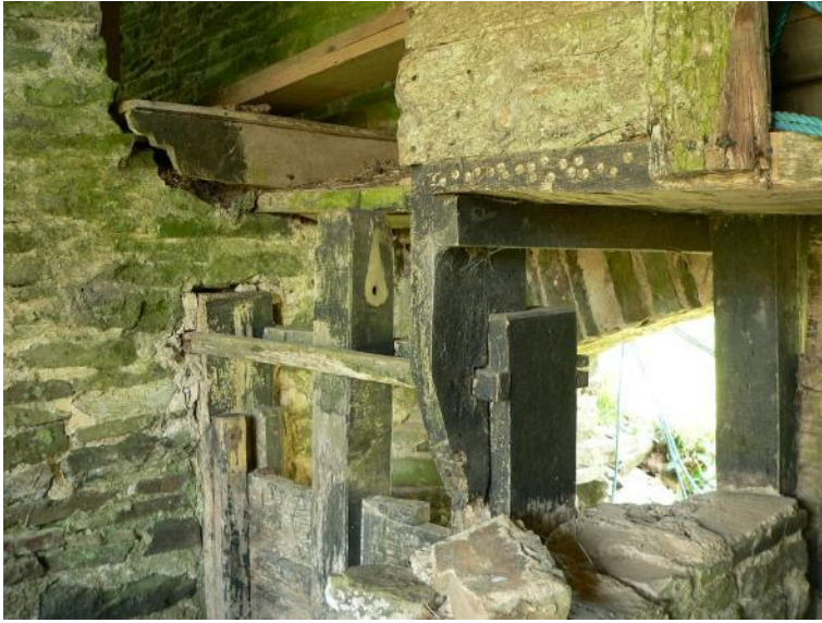
Top of penstock to north waterwheel, with timber supports for compartment over spillway
