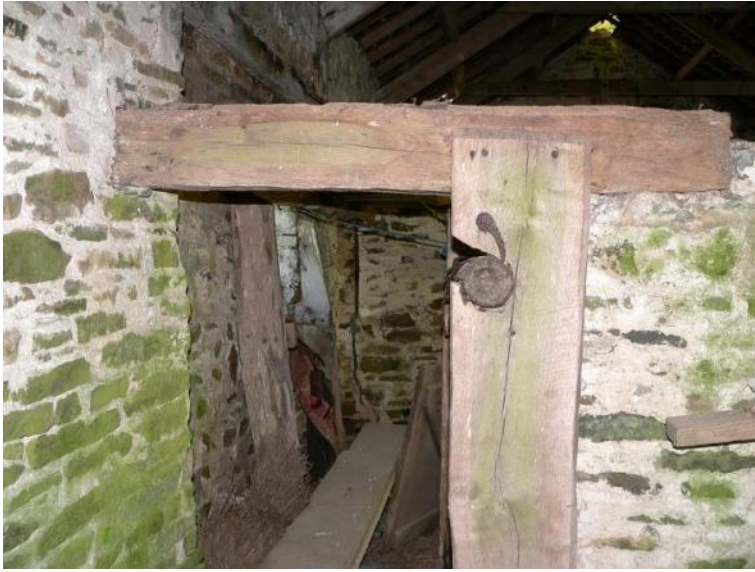
Ratchet on inner end of penstock control, north mill
