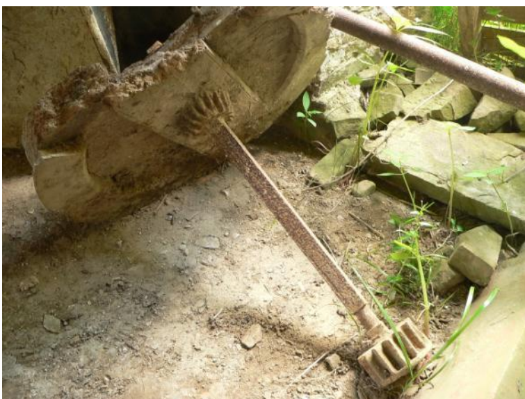
Displaced drive shaft (2), with cast-iron pinion and remains of timber pulley for belt drive to ancillary machine
