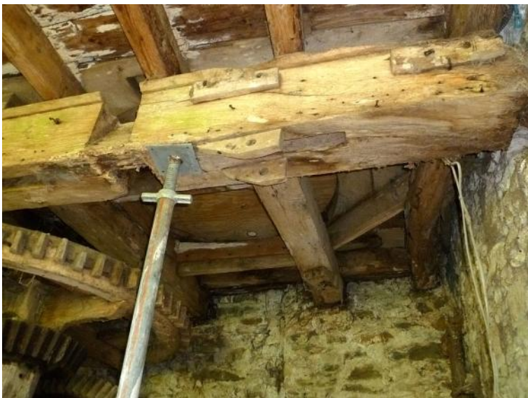
Downstream end of hurst bressummer, north mill, with cut out (left of prop) for meal spout from millstones
