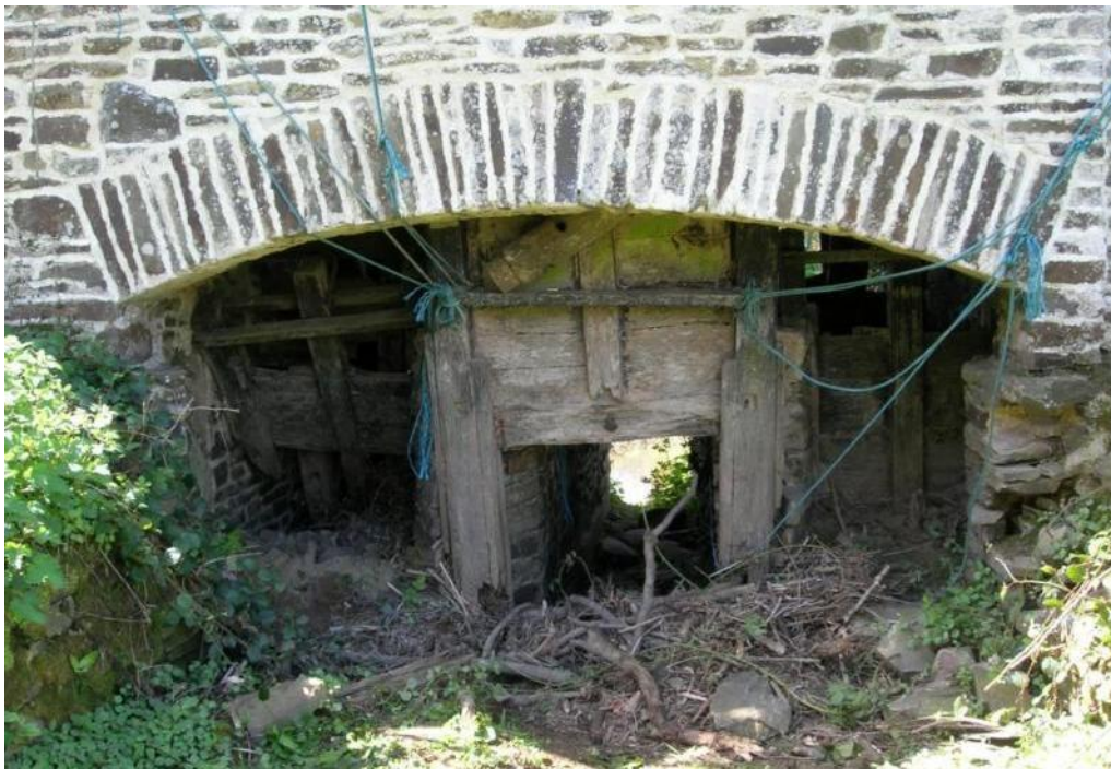
Headrace entrance, with penstocks to waterwheels each side of the central spillway
