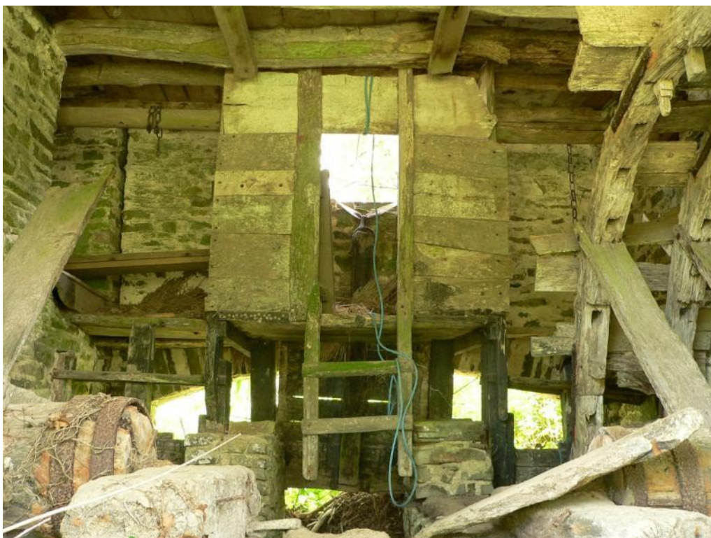
Wheel chamber with north wheel to left and south wheel to right, with central spillway. The short ladder down from the small timber boarded compartment over the spillway entrance was in place in 2012 but has now gone. There appears formerly to have been boards spanning over the spillway channel, to allow access to the outer wheelshaft bearings
