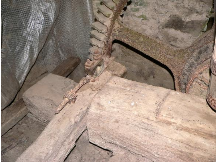
Ancillary drive shaft support timber with bearing at upstream side of pitwheel
