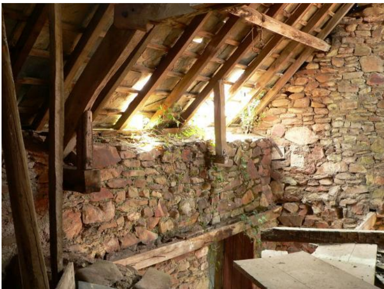
Roof and remains of upper floor over kiln, showing vertical struts under rafters
