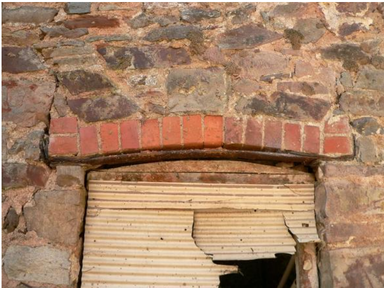
Detail of brick arched window head with iron strap lintel, northwest elevation of kiln
