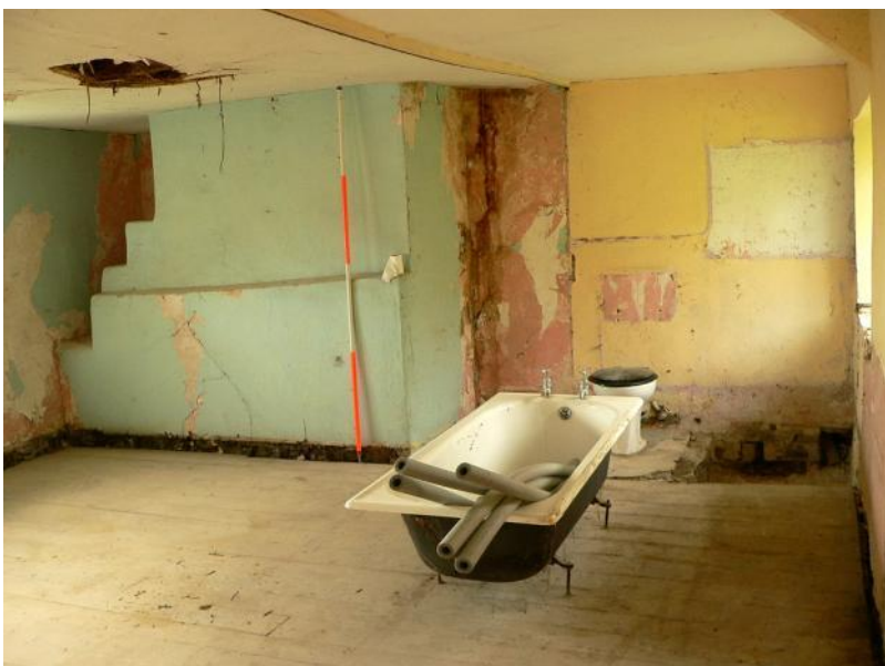
Gable end of first floor south room after removal of bathroom partition
