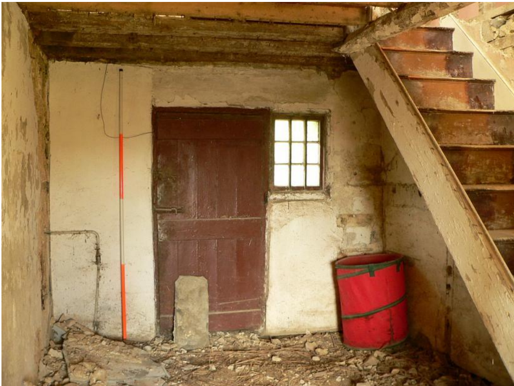
Ground floor, former dairy, looking west to back door, with stair to right
