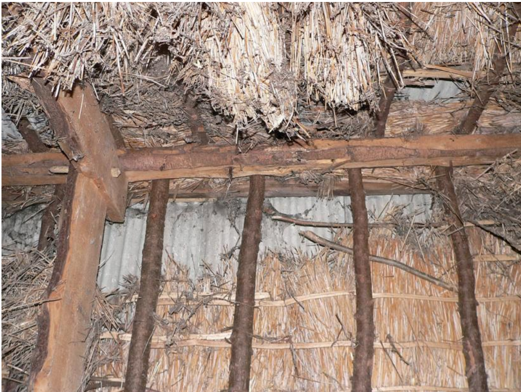
Apex of roof truss, ridge purlin and rafters with remains of thatch
