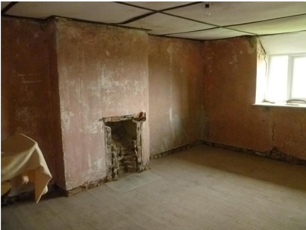
North room, looking north-eastm chimney breast with fireplace removed. Note foot of roof truss principal to left of window reveal
