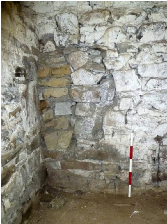
Blocked opening in north-east corner
