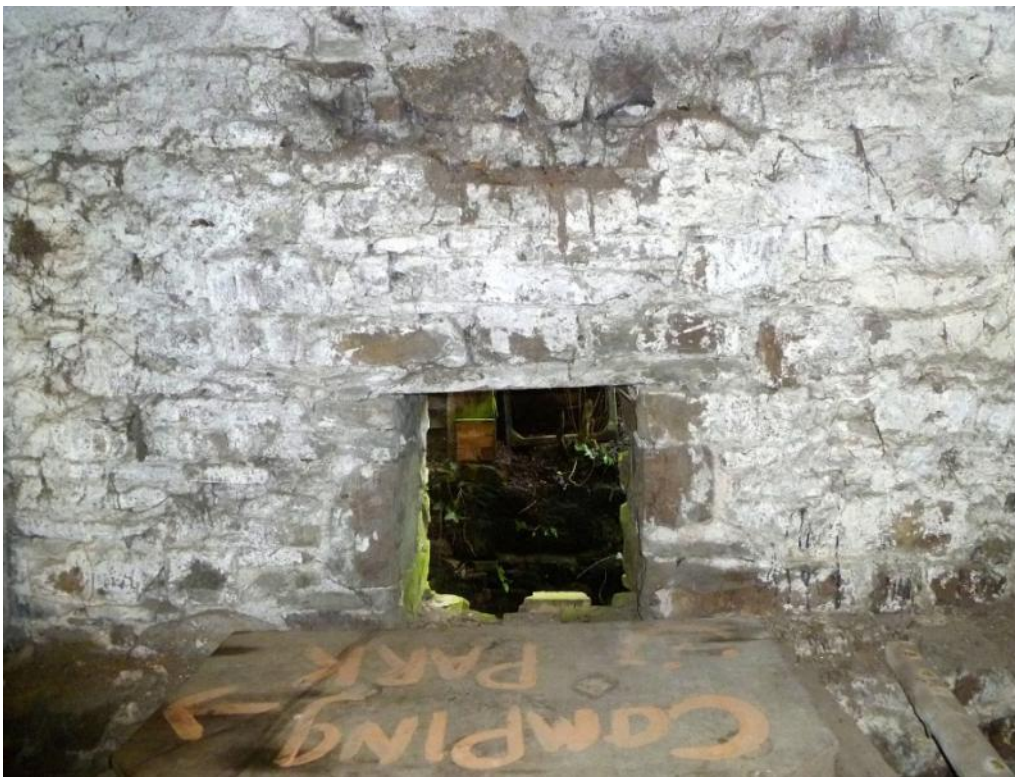
Waterwheel shaft opening through east gable end wall, with recess in wall over for clear rotation of spurwheel
