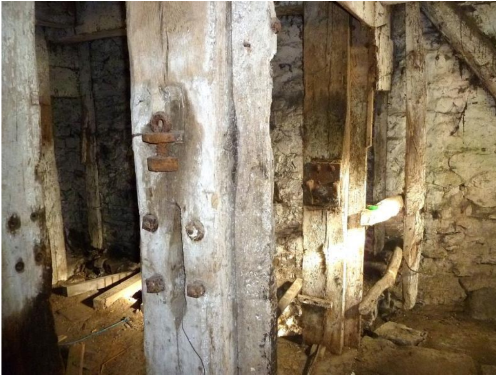
Remains of fittings to locate and adjust bridges on south side of hurst
