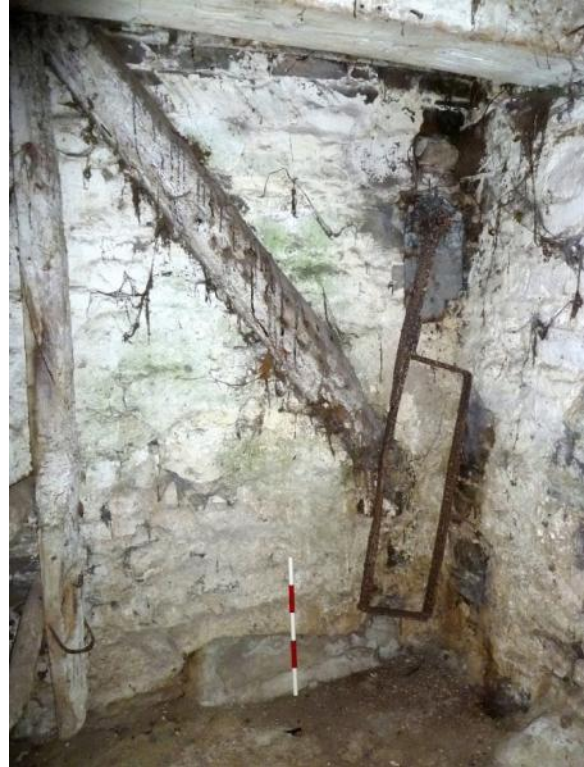
Penstock control lever in south-east corner
