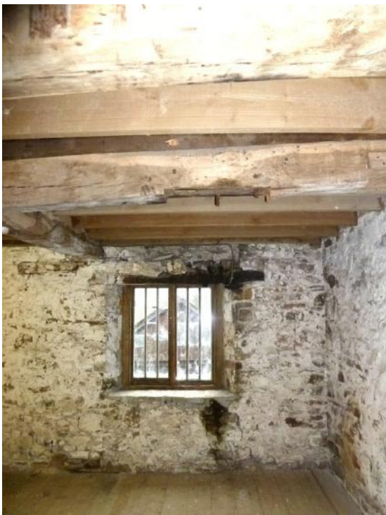
Layshaft bearing positions, hung from beam (centre) and on lintel over window
