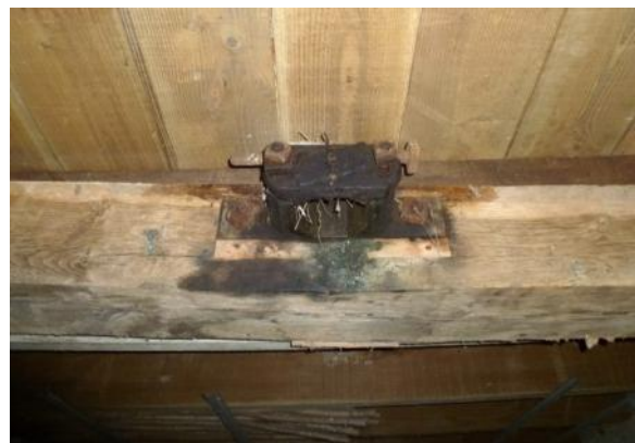
Plummer block (bearing) for head of upright shaft above first floor level
