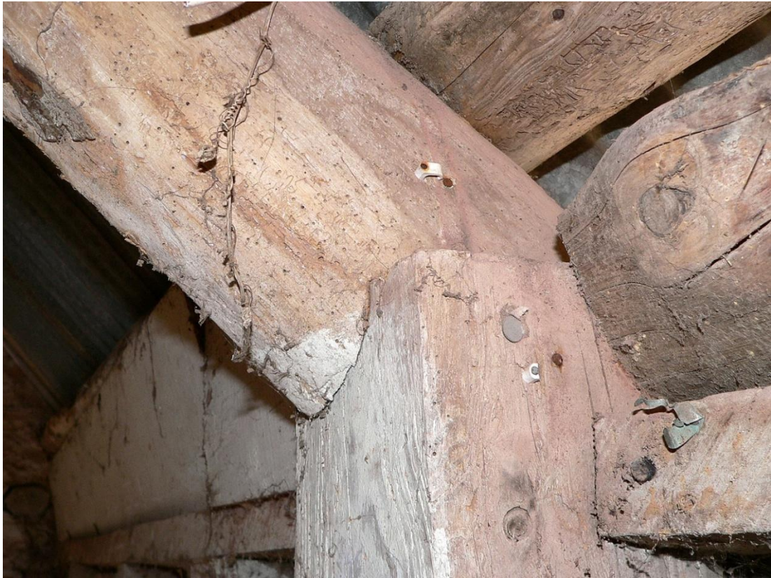
Foot of roof principal jointed to post (Note that the round object is a nail head, not a peg!)
