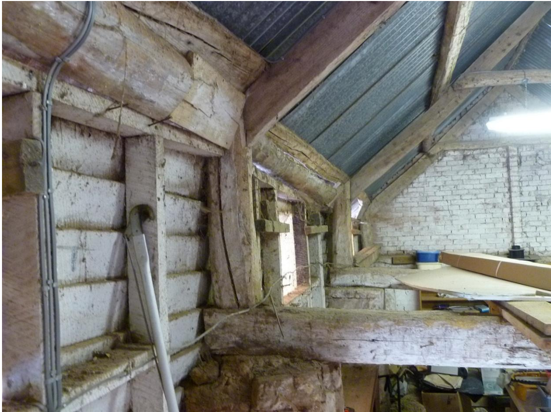
NE end of tie beam with post supporting foot of principal on head of column
