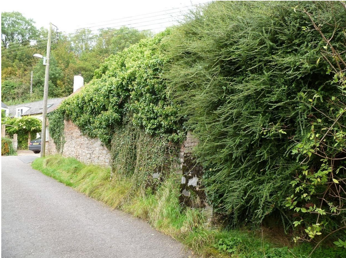
SW elevation looking up Post Office Lane; the buttresses are just visible on the right
