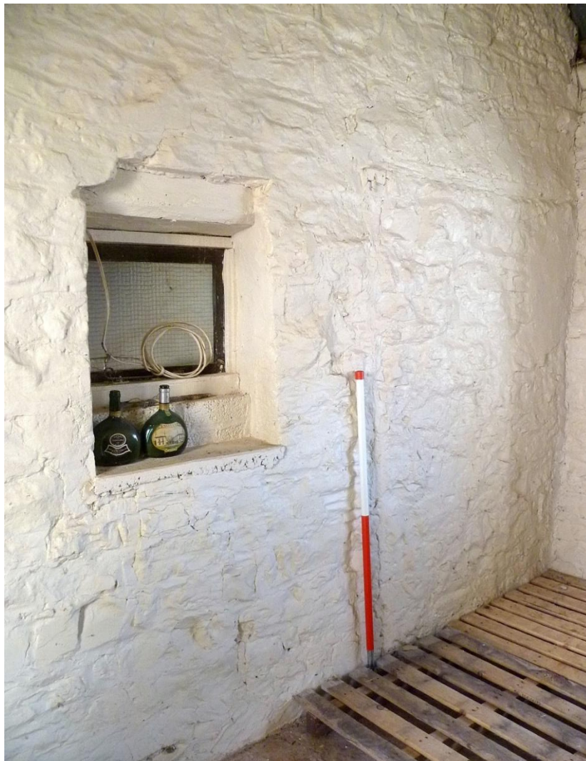
Wall between bays 5 and 6 with blocked doorway to right of 1m scale
