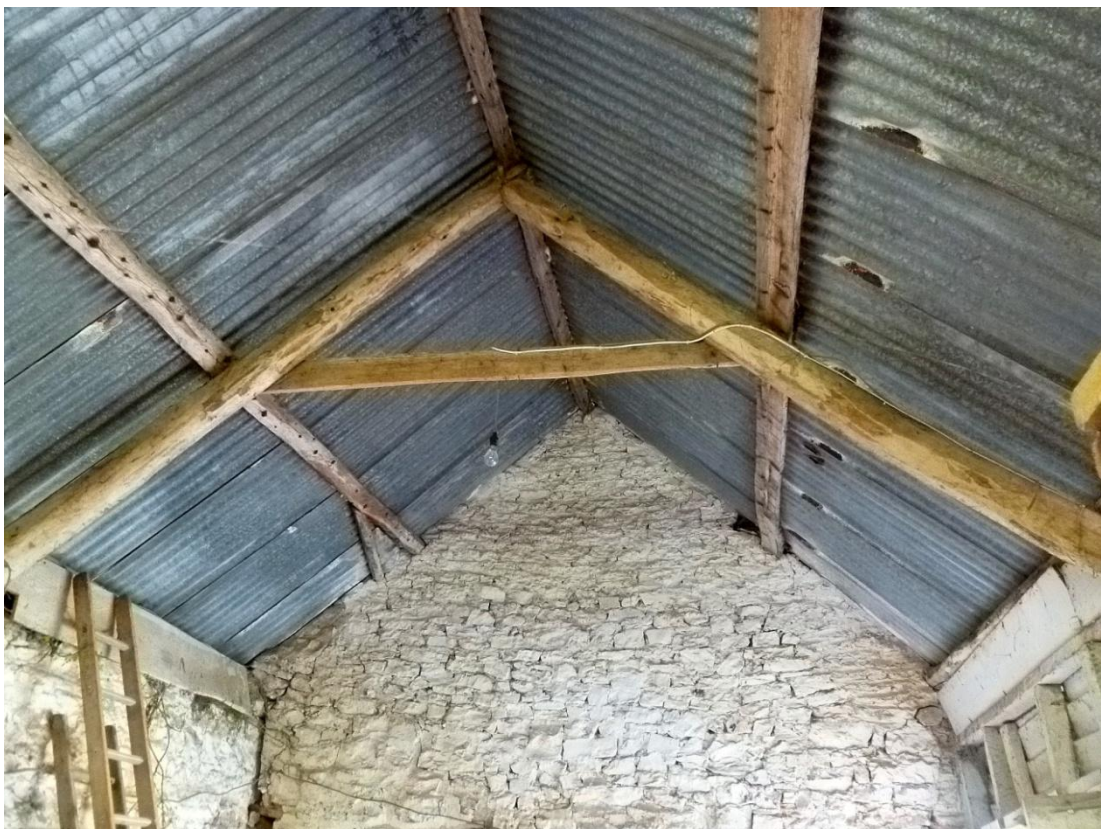
Roof truss between bays 4 and 5, from NW, with stone wall to bay 6 beyond
