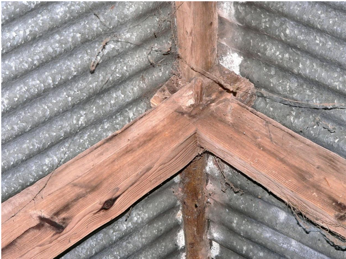
Apex of principals, from NW, showing cross over, peg and ridge support
