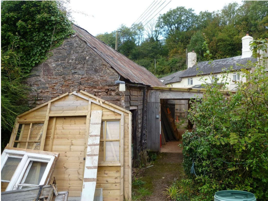
SE gable end, with modern extension to right and the former Farmer's Hotel in the background
