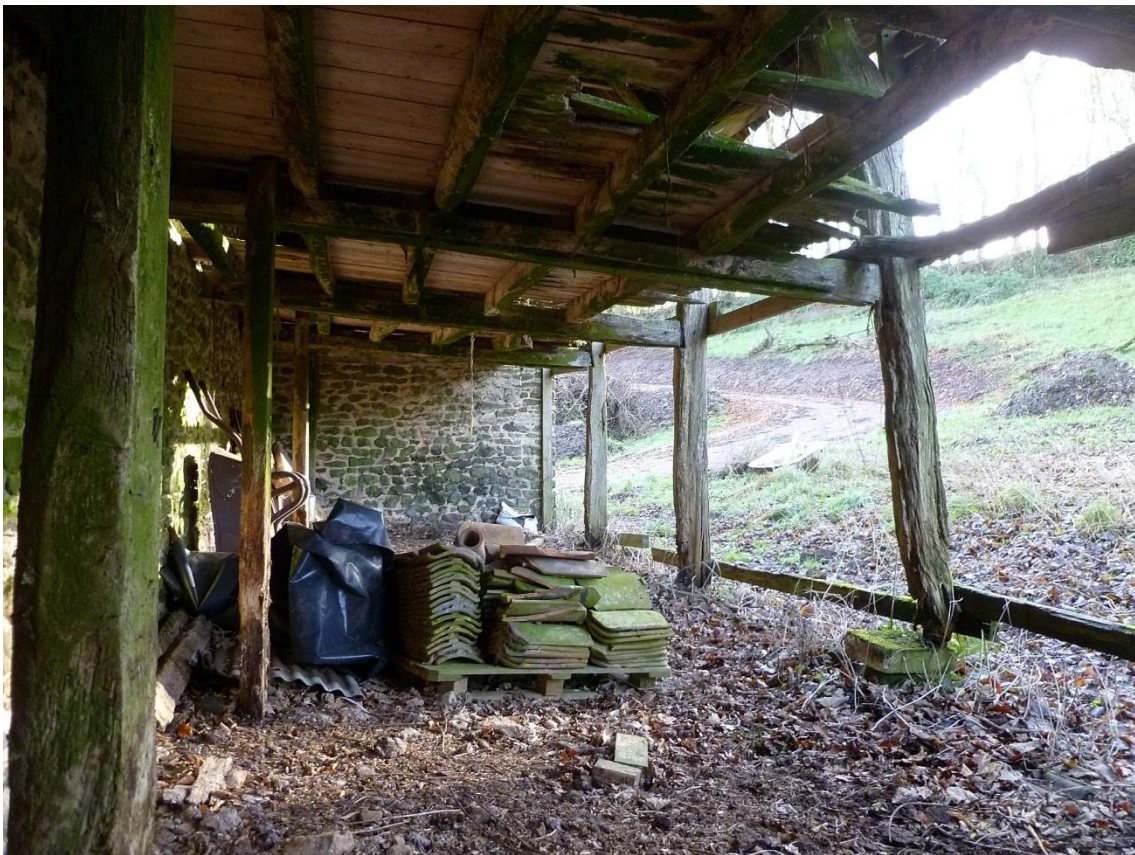
Interior looking east, showing tallet floor and secondary props under cross beams to left
