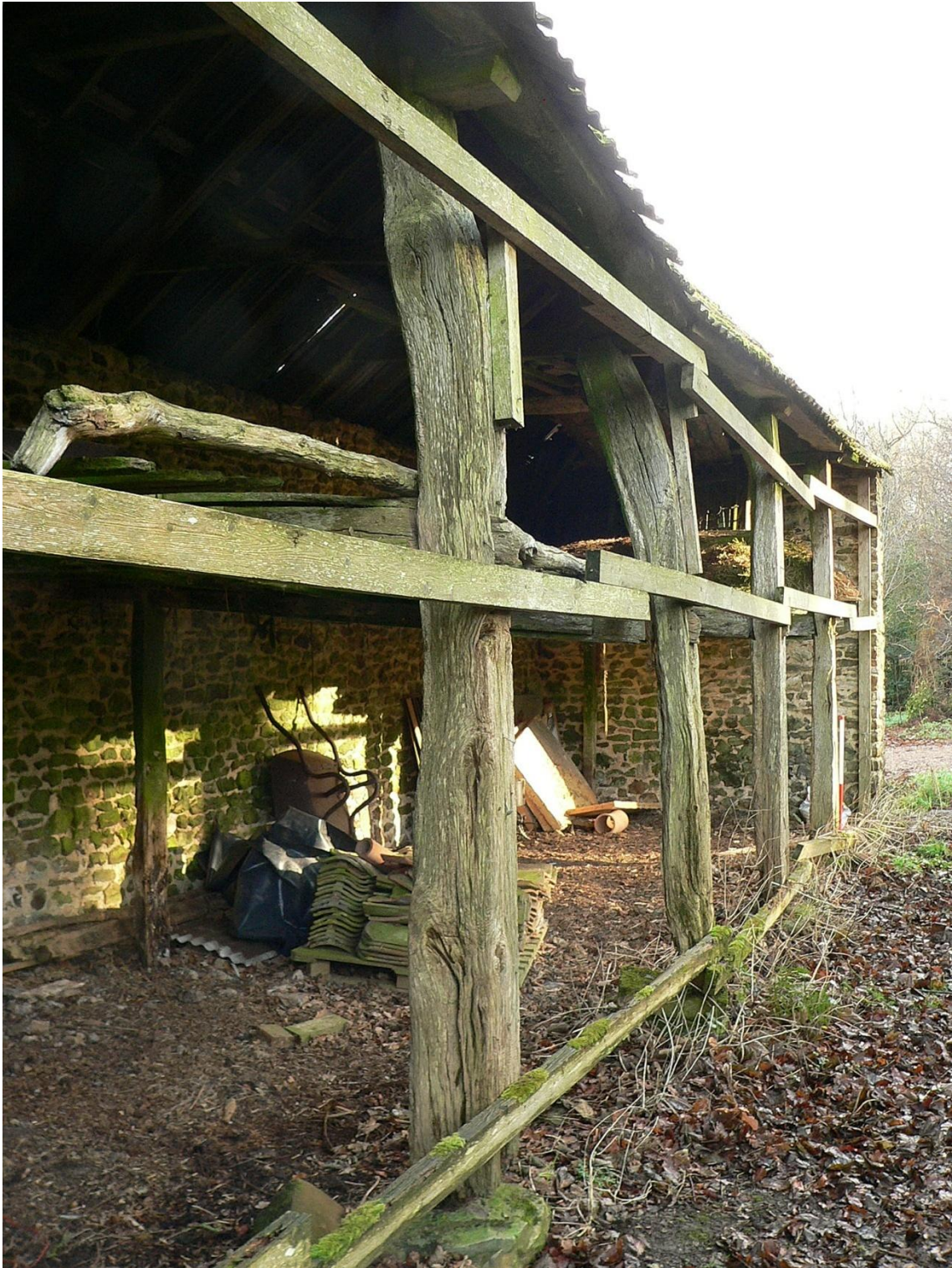
South front of linhay, looking east, showing curved tops to P1 and P2
