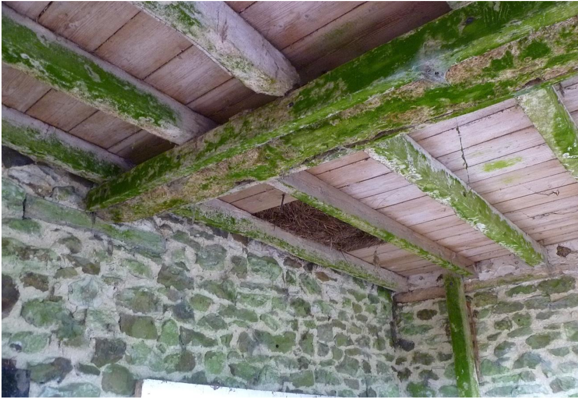
Cross beam and joists on timber plates built into walls in north-east corner
