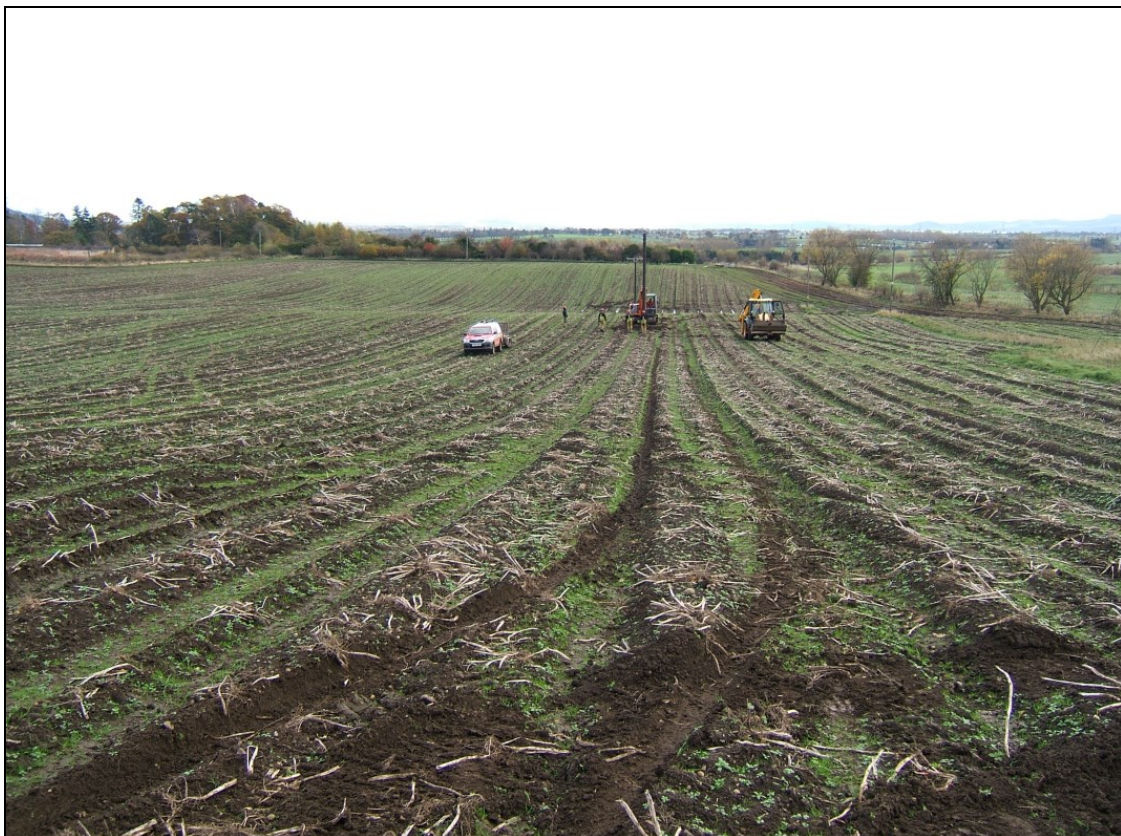
View from the west across the east field, Pole 48 being inserted in the distance
