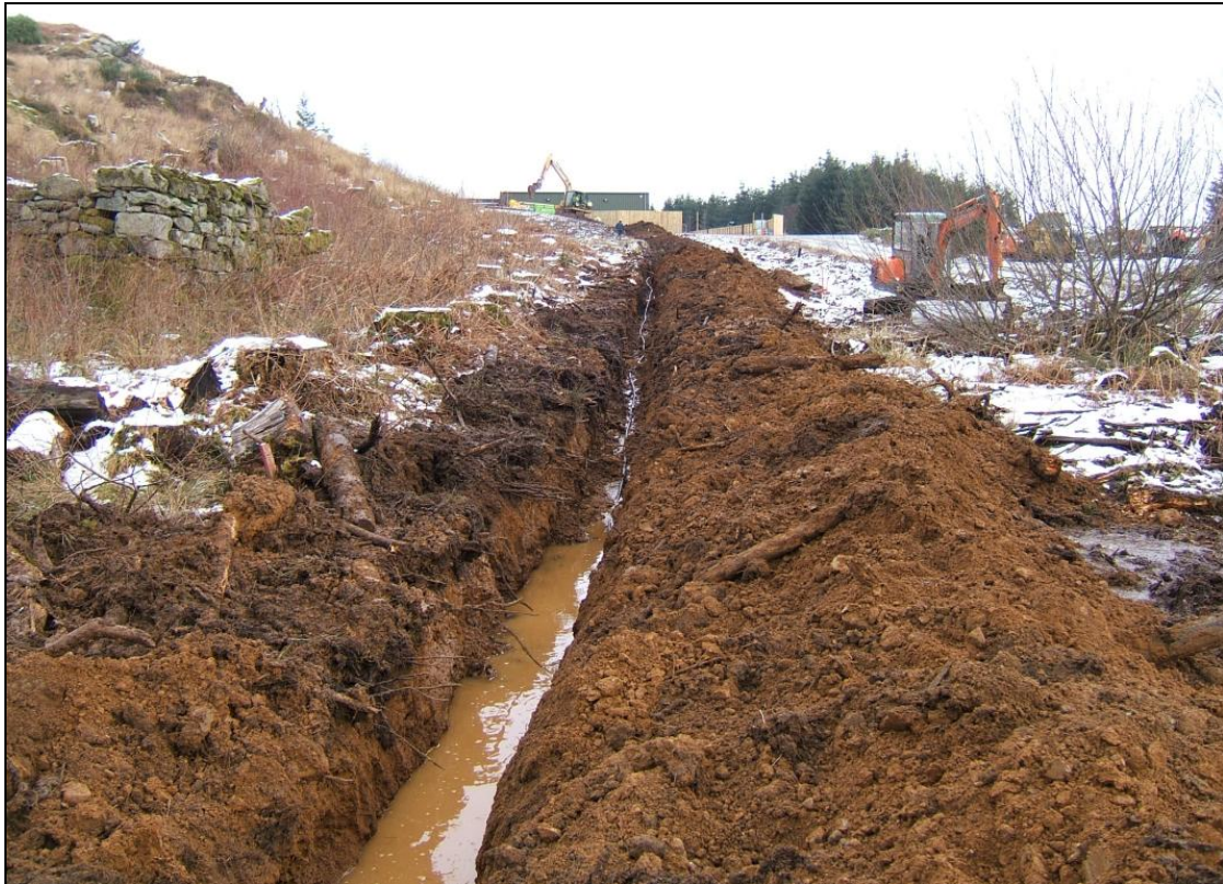
The cable trench viewed from the south-west with the ruins of one of the buildings of Tomdow on the left
